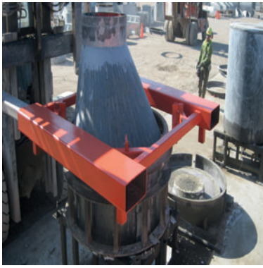
A forklift attachment allows the operator to set the header and pallets in a safe and efficient manner
