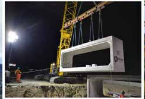
Placing a 24 x 6.5 Box Culvert Section for "The Point" Project, Utah Photo: Oldcastle Precast
