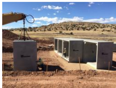
Four-barrel (10-ft-by-10-ft) dry-cast concrete box culvert for storm water management and cattle crossing.
