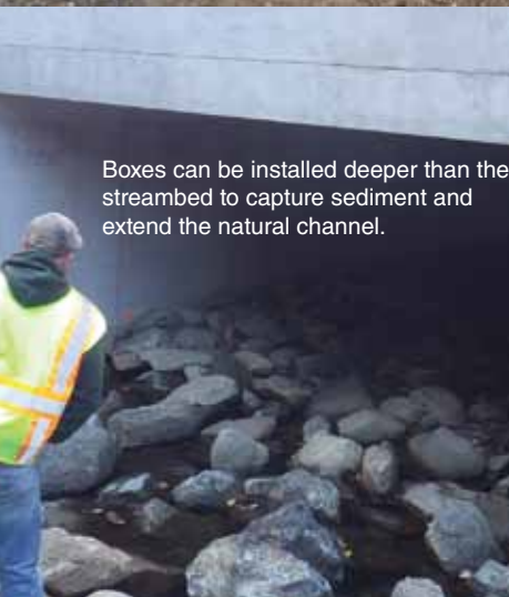
Replacement of CMP culverts that have reached the end of their service life before the design life of the Interstate highway system in Vermont.
