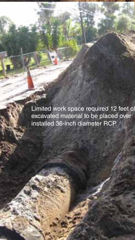
36-inch diameter RCP installed to Standards with compaction to spring-line and finished grade.
