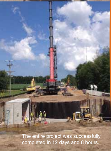
4-foot box sections that weighed 52,000 lbs. each were designed to MDOT's HL-93 Modified Design requirements.
