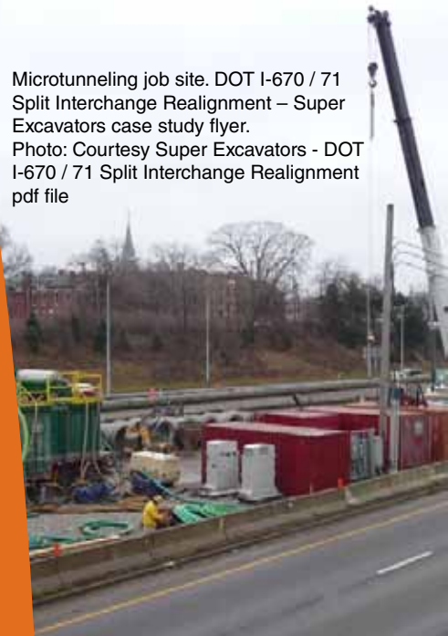
One of 6 work shafts for microtunneling Class 4 RCP. Photo: Hanson Pipe & Precast
