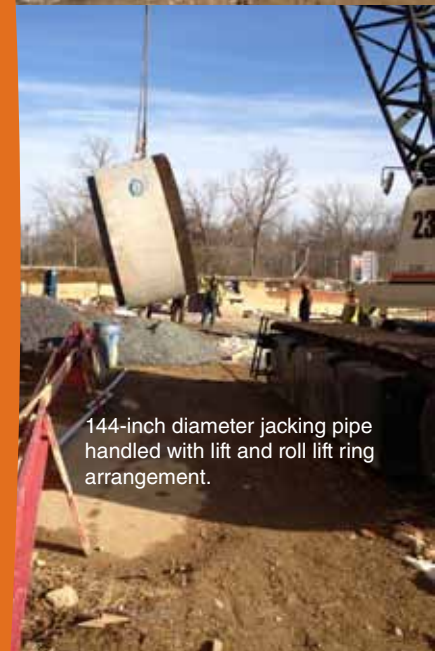
144-inch diameter jacking pipe offloaded with lift and roll lift ring arrangement.
