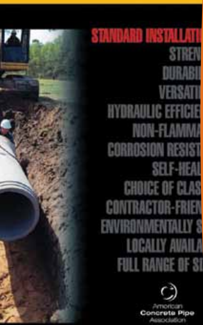
Type 2 Standard Installation of 1800mm RCP on Powell Street Overpass project in Vancouver, B.C.
