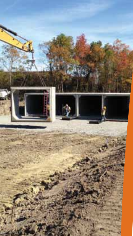
Installation of four 210-foot runs of 10-foot x 8-foot box sections for construction of quad-cell culvert. Photo: Scott Jordon, P.E., ACPA
