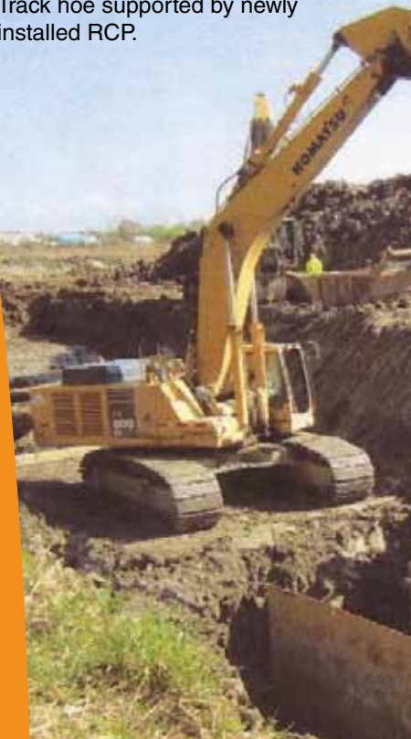
Pre bed RCP C76 CL V with a T-Lock PVC liner being lowered into trench.
