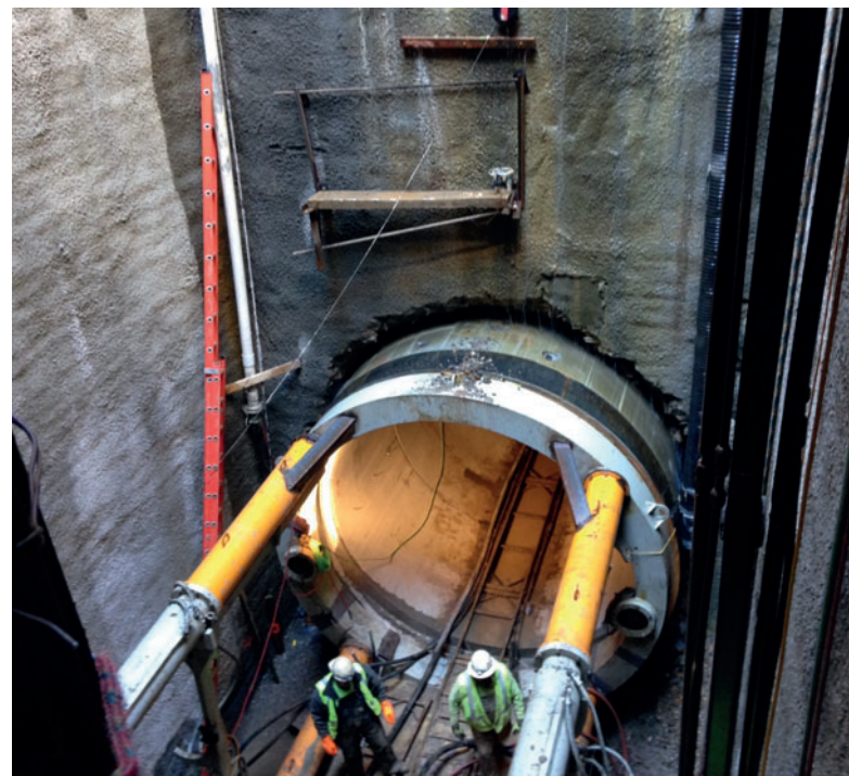
144-in. dia. Jacking Pipe for Blue Plains Influent Sewers. Photo: Mike Barna, Concrete Pipe & Precast, LLC, MBarna@concretepandp.com
