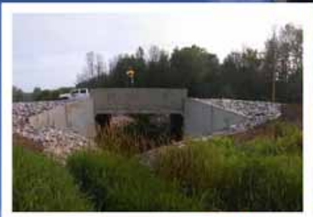
Completed Installation of the Phillip Drain Bridge Replacement Photo: Northern Concrete Pipe Inc.
