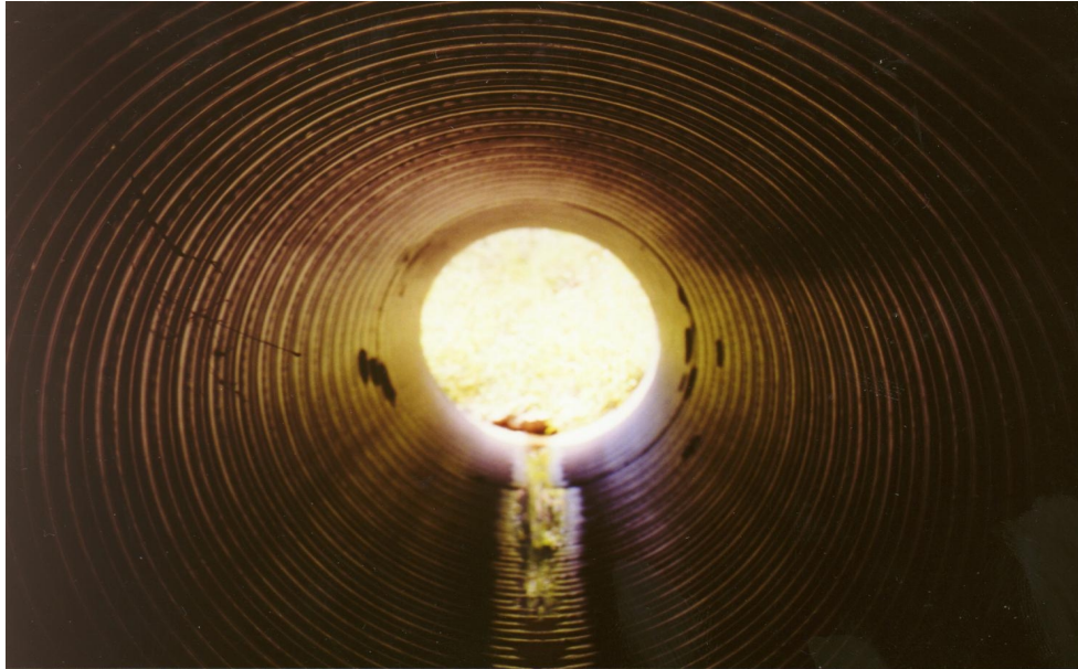
Good shape and alignment – Pipe 3
