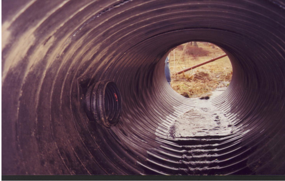
Bulge at the bottom of the pipe and cracks in the top of the pipe – Pipe 7
