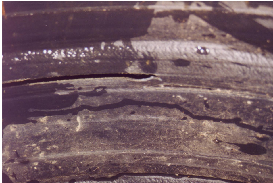
Crack at 10-ft. – Pipe 5
