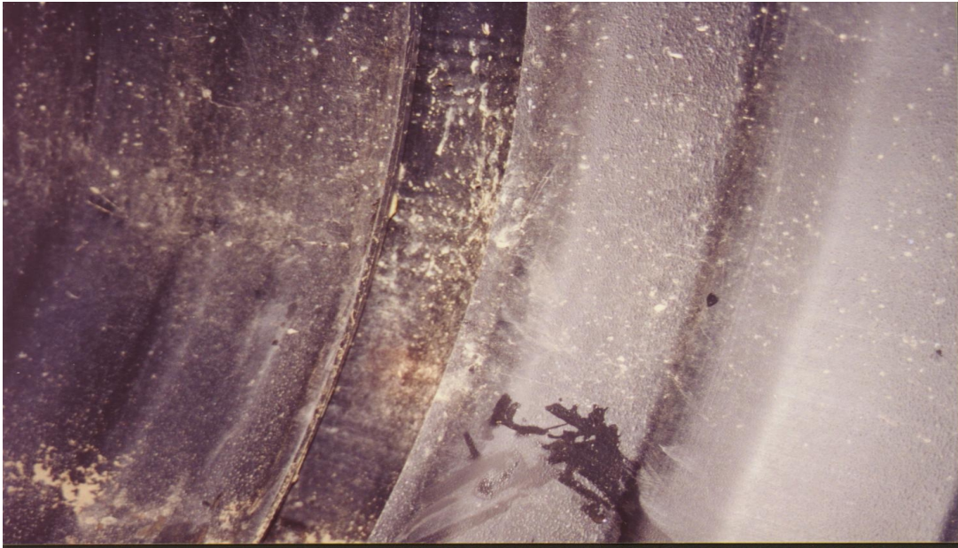
Separation at Joint 1 – Pipe 8
