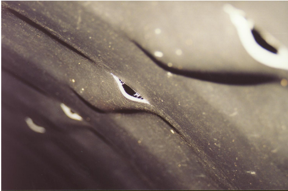
Splitting of Pipe 6
