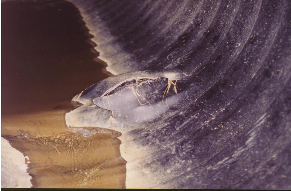
Bulge and crack in bottom of pipe – Pipe 8
