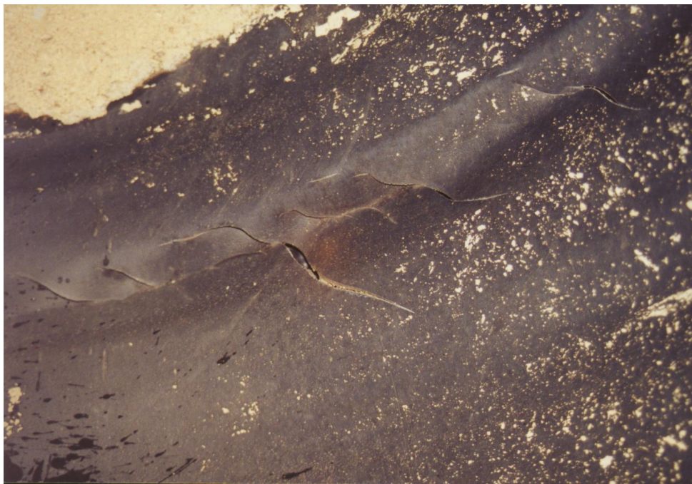
Cracking of Pipe 7
