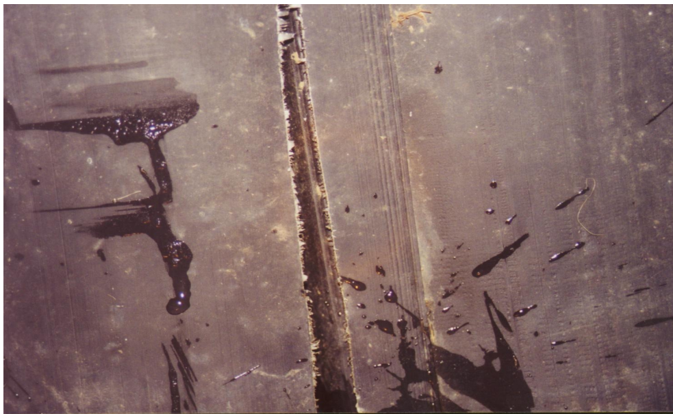
Crack at 7-ft. – Pipe 7
