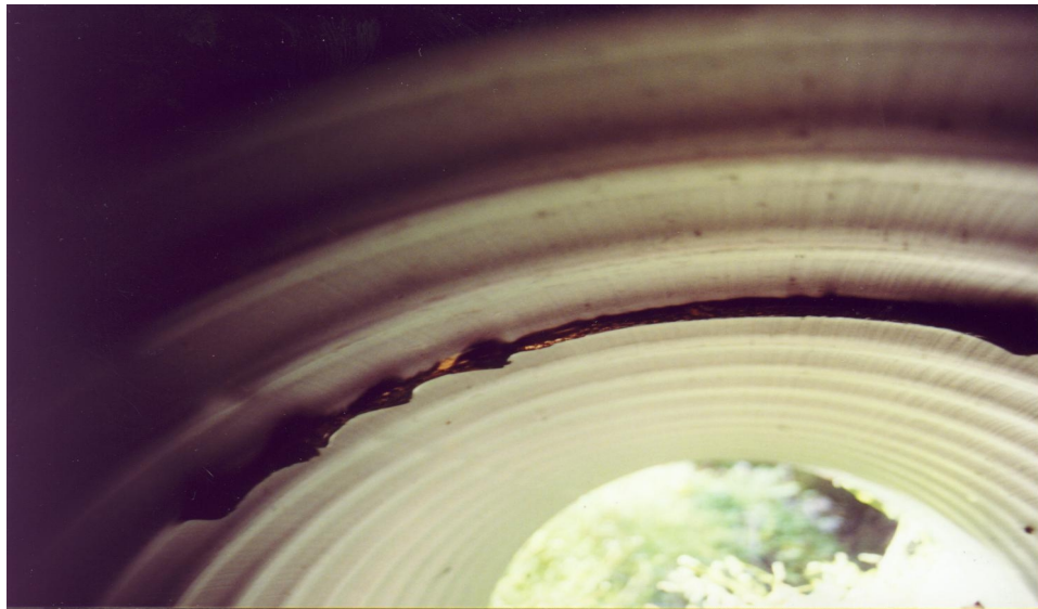
Lacerations in top of pipe – Pipe 5
