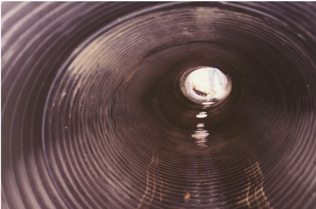
Profile of pipe: Note wall buckling and obvious oval shape – Pipe 9
