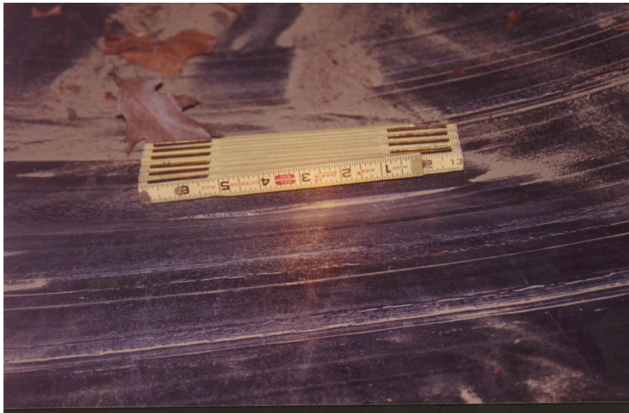
Crack on top of the bulge at 34-ft – Pipe 6
