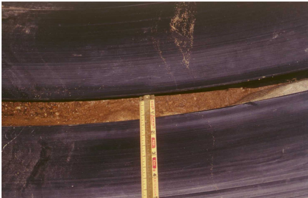
Separation at Joint 1 – Pipe 9
