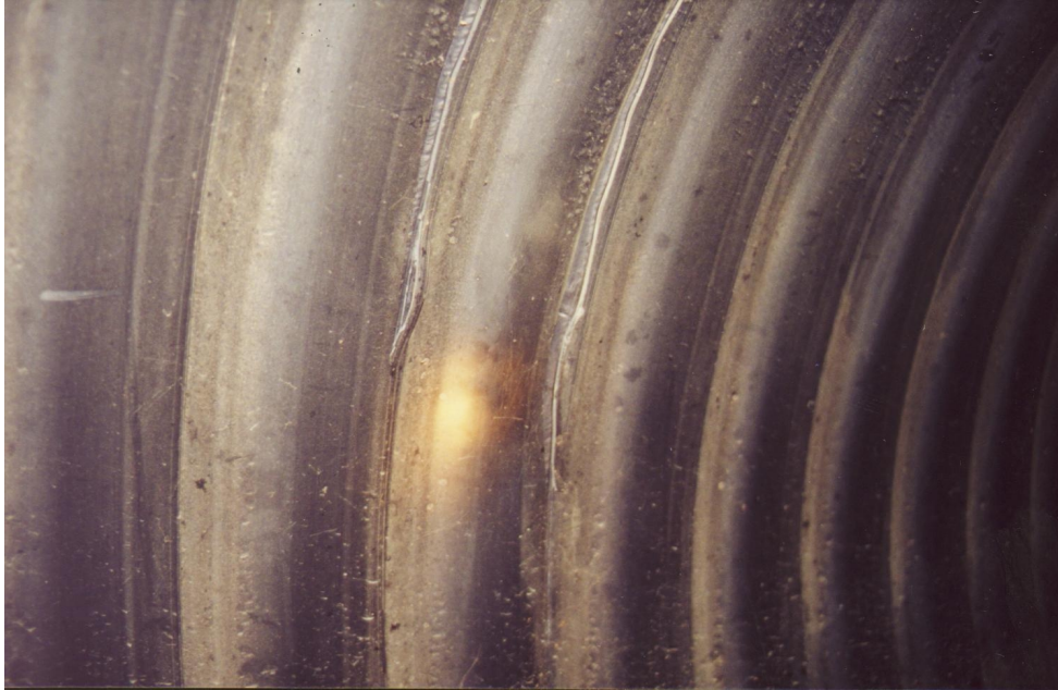
Two cracks that have developed in the pipe – Pipe 5
