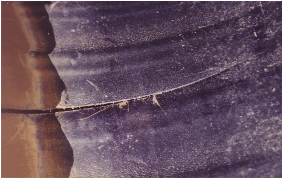
Crack at 50-ft. - Pipe 8
