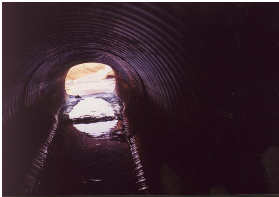
Obvious deflection of the pipe- Pipe 1
