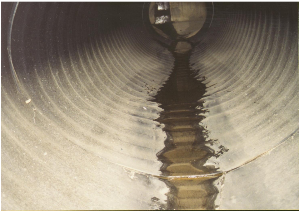
Bulge in the bottom of Pipe 6
