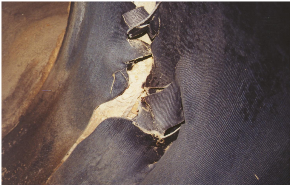
Cracking at outlet of Pipe 7
