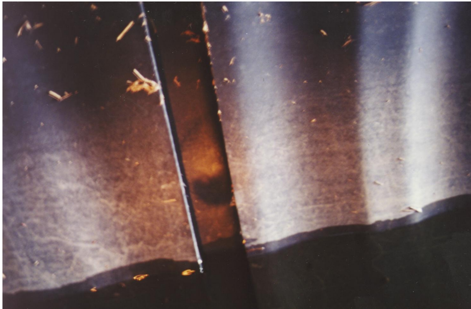
Separation at Joint 1 – Pipe 2
