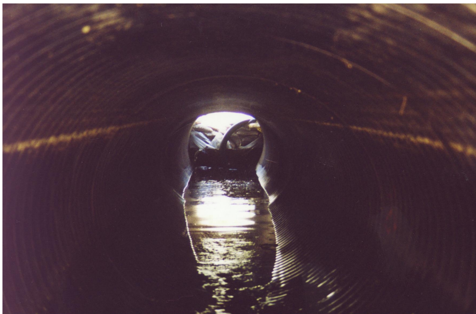
Oval shape of the pipe – Pipe 3
