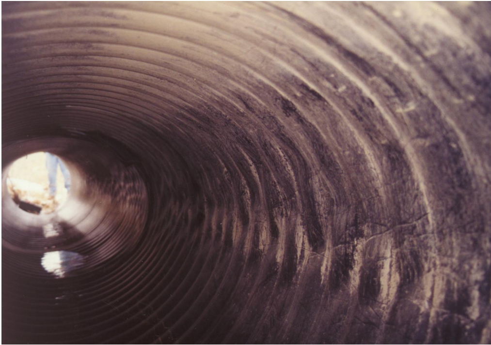
Rippling of the sidewalls – Pipe 9
