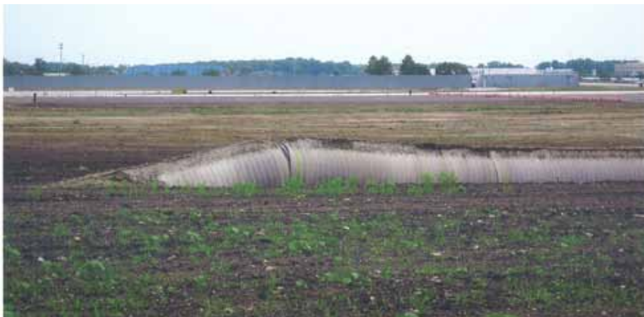
Figure 1. Floatation of 60-inch Polypropylene Pipe at Port Columbus International Airport
