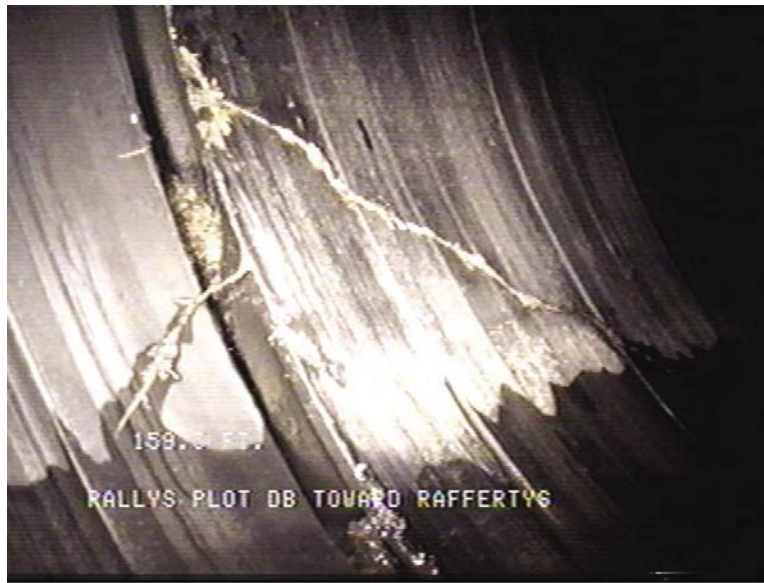
Video Image on Project 1, Nicholasville Road, showing severe radial cracking near a joint.
