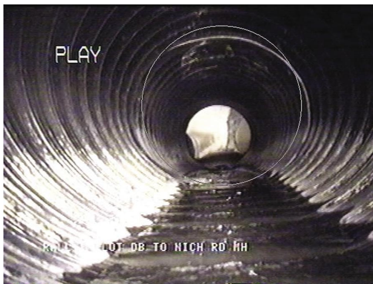
Video Image on Project 1, Nicholasville Road, showing 10% deflection and corrugating growth.
