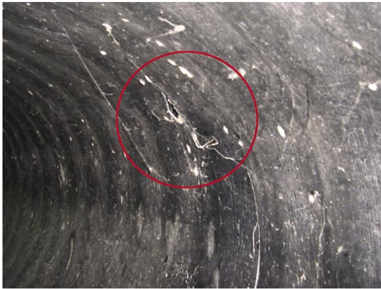
Project 11, Homer, showing cracking and buckling approximately 2 feet from outlet
