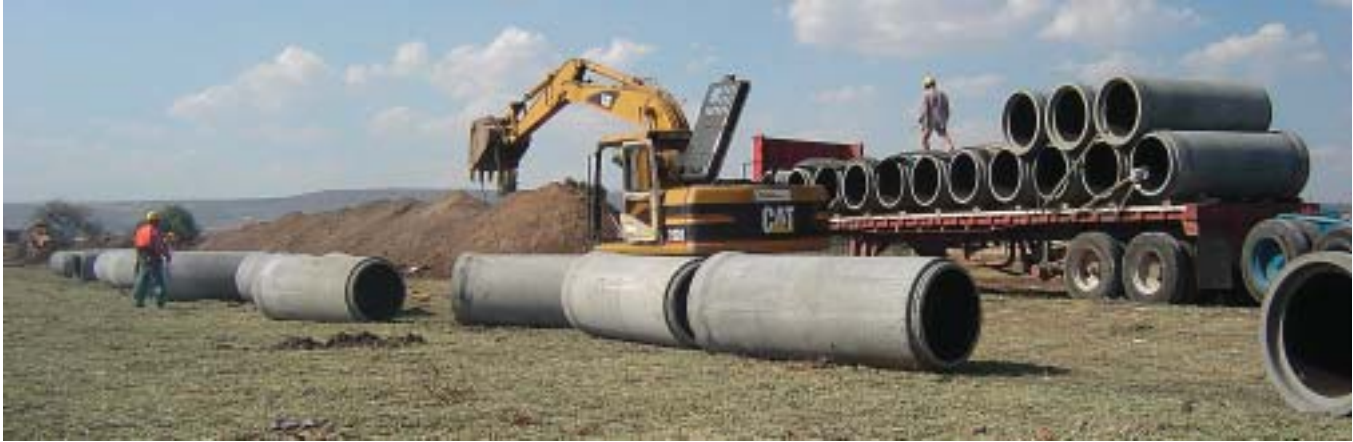
Delivery of 750 mm and 900 mm diameter reinforced concrete pipe for three kilometer sanitary sewer.
