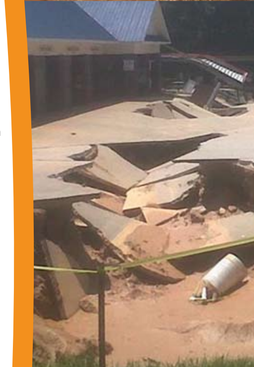
Dramatic 2010 washout of the storm sewer at the Sonic Restaurant.
