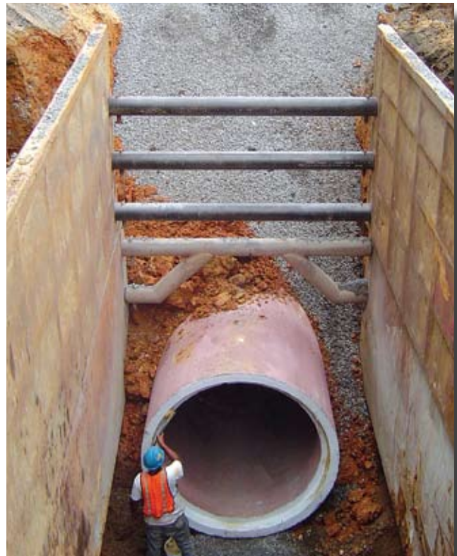
1,000 feet of 72-inch diameter Class III RCP installed by open cut method.
