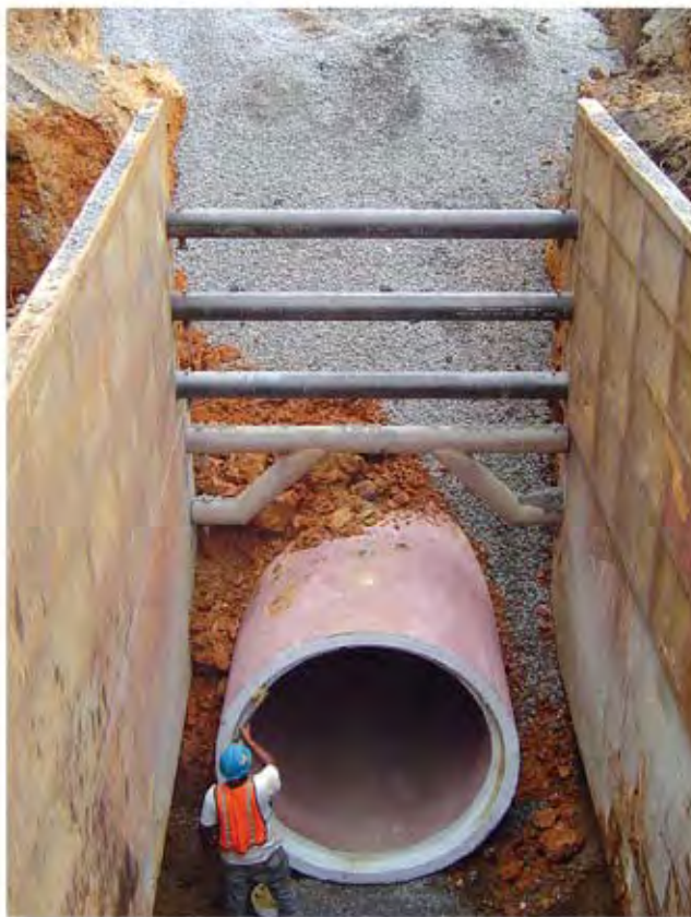
1,000 feet of 72-inch diameter Class III RCP installed by open cut method.
