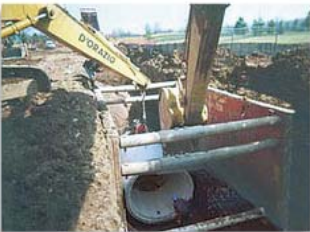
A fast-paced schedule and safety considerations required the use of trench boxes for much of the 15.5 kilometers of RCP installed along the Highway 25 right-of-way.
