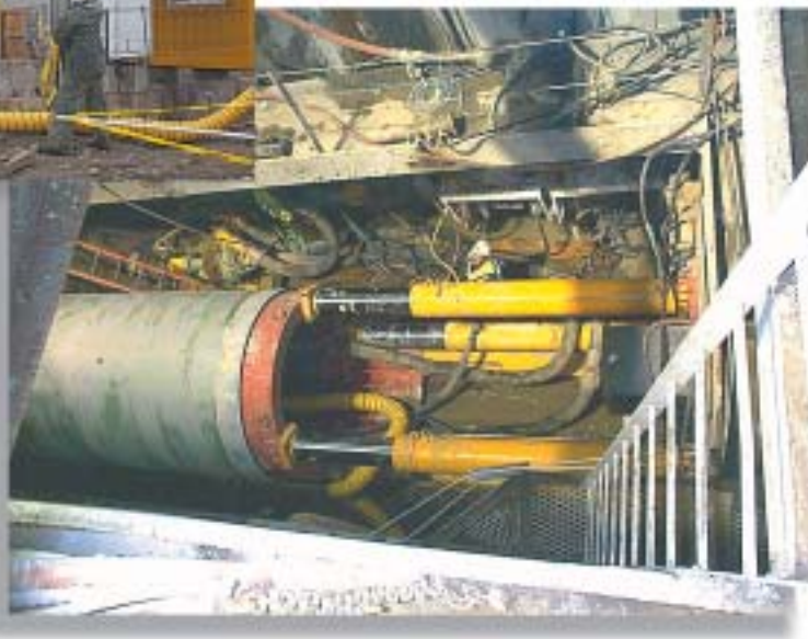
Around-the-clock deliveries of microtunnel pipe were required to allow pipe to be fed continuously into the jacking pits.
