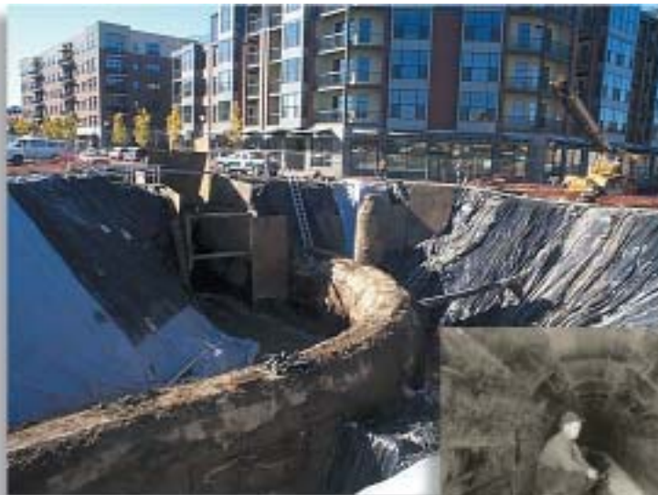
72-inch diameter RCP is being installed adjacent to the original Tanner Creek Diversion sewer in downtown Portland.
