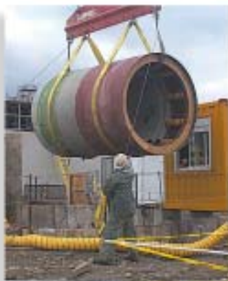
A 72-inch diameter intermediate jacking station section being lowered into the jacking pit.
