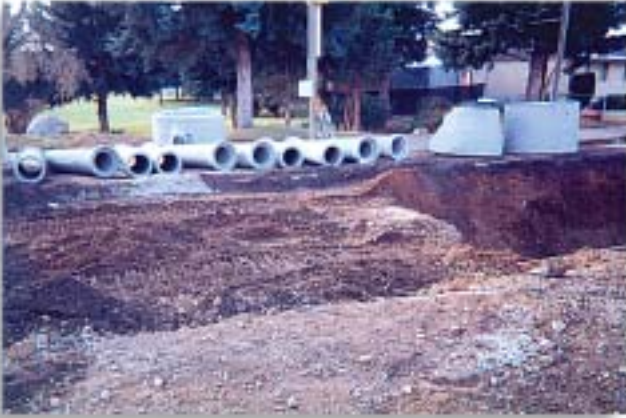
Rigorous testing, on site inspection and quality installation helped assure a successful project.
