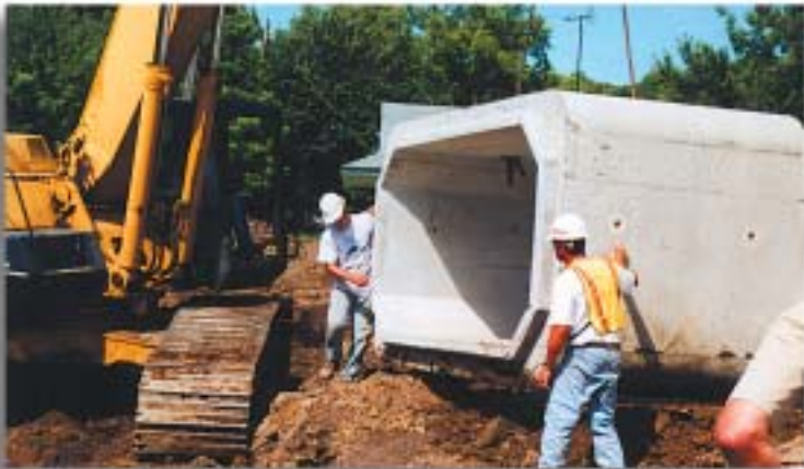
Precast concrete box sections allowed crews to complete the project in 13 days, with limited traffic disruption and inconvenience to businesses and residents.
