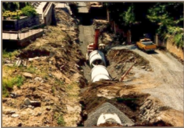
Kiewit laying 84" pipe down the middle of the Haxal Canal on CSO 3.
