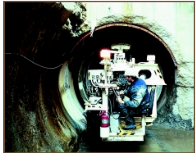
A unique pipe carrier was used to install 90-inch diameter pipe in a rock tunnel that extends under the James River on the southside for Phase 1.
