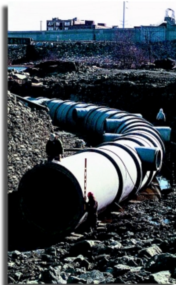
Workers lay 90-inch diameter pipe with 36-inch outlets near the outfall of Phase 1.
