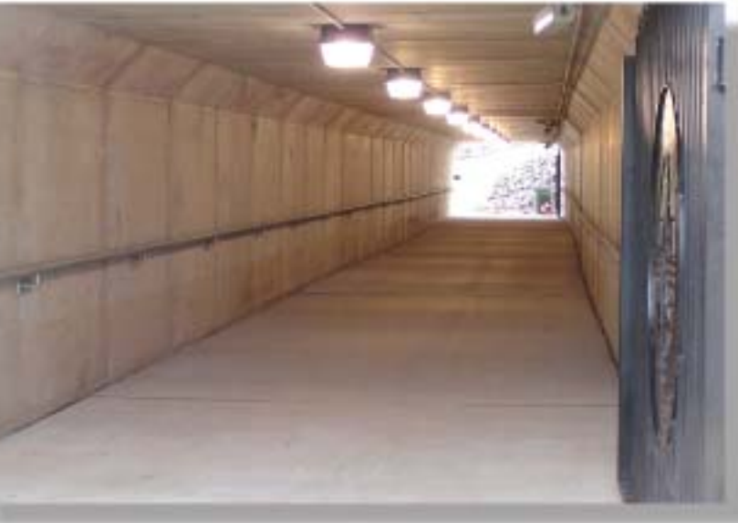
City of Houghton provided lighting, security cameras and gates for the tunnel.
