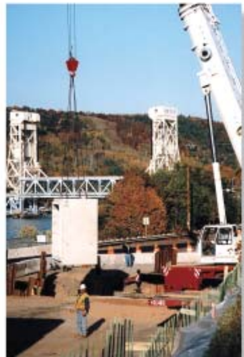
Photo: John Kloet, Upper Peninsula (U.P.) Concrete Pipe Co.
