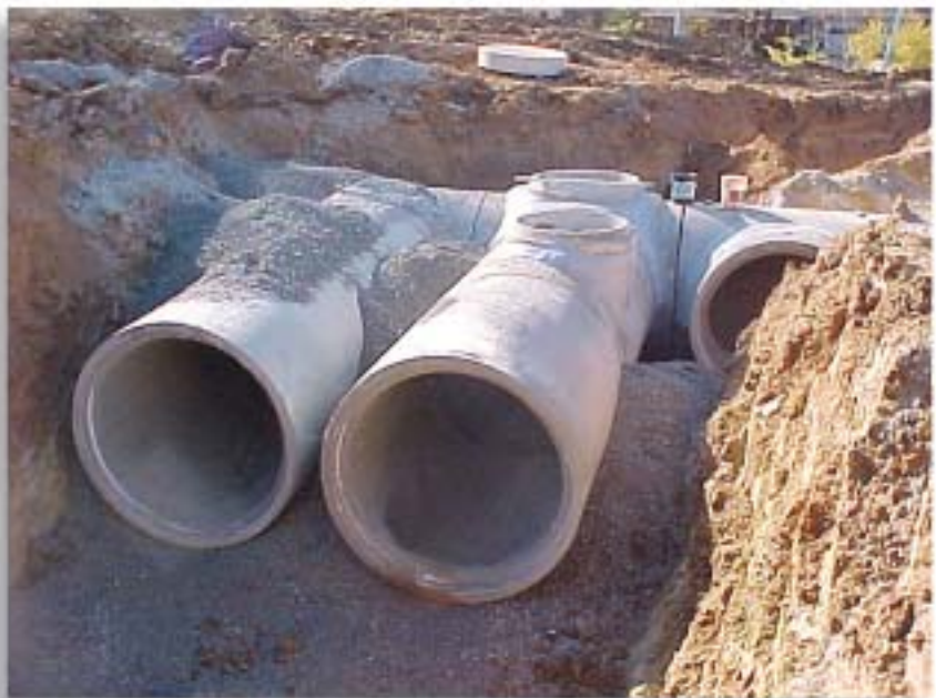
Installation of the 72-foot runs of 66-inch diameter RCP went smoothly and provided the owners with the ability to add a parking surface above the structure.
