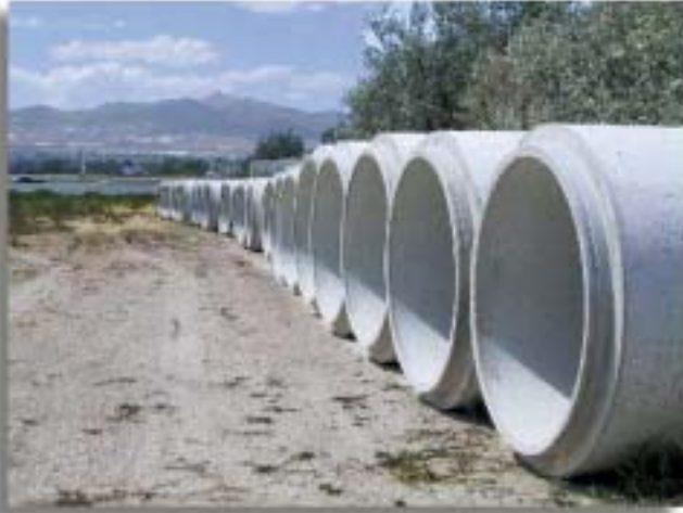
60-inch and 48-inch diameter RCP was staged for installation along Interstate 15 in Sandy City. Utah's Oquirrh Mountains provided a scenic backdrop for crews.
