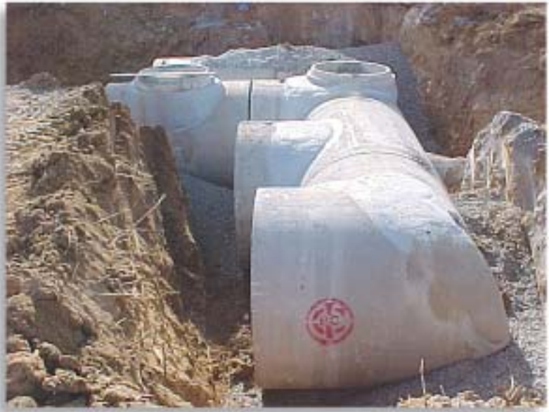
The system included 66-inch x 66-inch diameter 90° elbows and tees with four 72-foot runs of 66-inch diameter reinforced concrete pipe.
