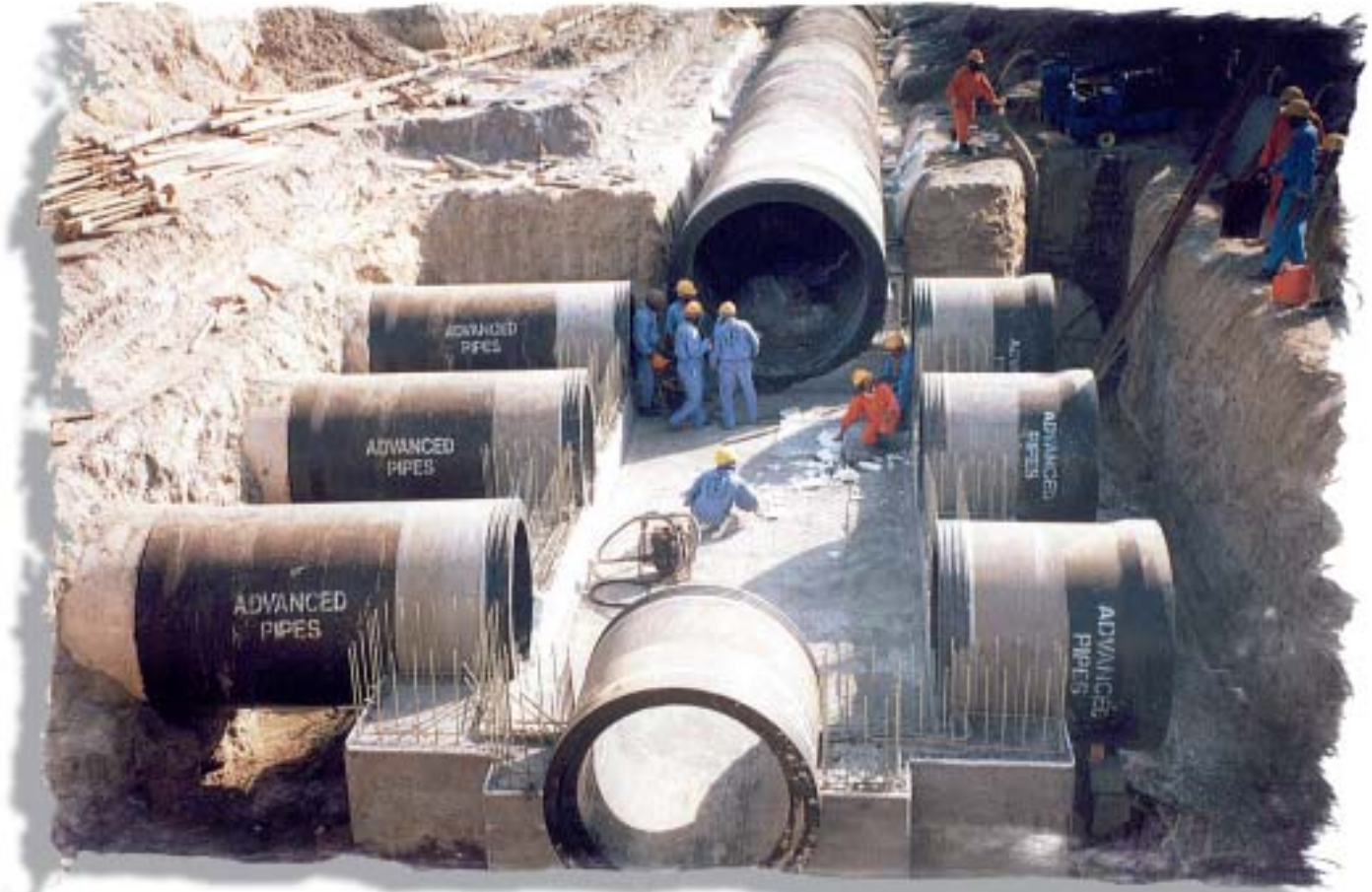
Seven lines of 1400-mm (54-inch) diameter reinforced concrete pipe converge in a manhole where a 2400-mm (96-inch) diameter line will transport the water to a treatment station.
