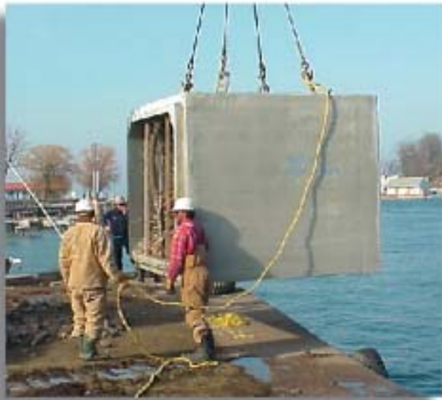
The installation of 2400-mm wide x 1800-mm high x 2500-mm long (8-foot x 6-foot x 8.2-foot) precast concrete box units helped divert strong currents and water surges and provide a safer docking area for boaters.
