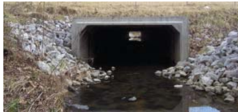
12-foot x 6-foot reinforced concrete box culvert replaced failed multi-plate cmp arch
