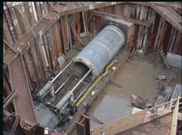
Denver's T-REX Transportation Project includes 1,500 feet of precast concrete pipe that will be bored and jacked into position.
