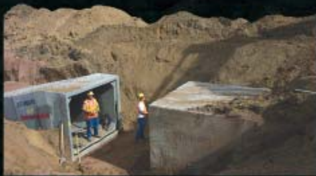
The installation crew gets ready for placement of the final section in grade transition box culvert line.
