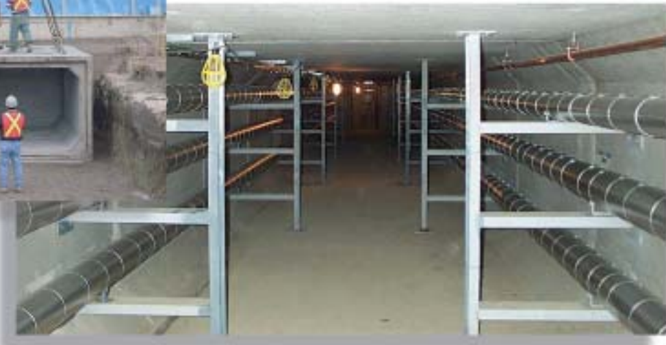
The below-grade precast concrete box structure provides excellent security and convenient access to the HVAC piping systems.
