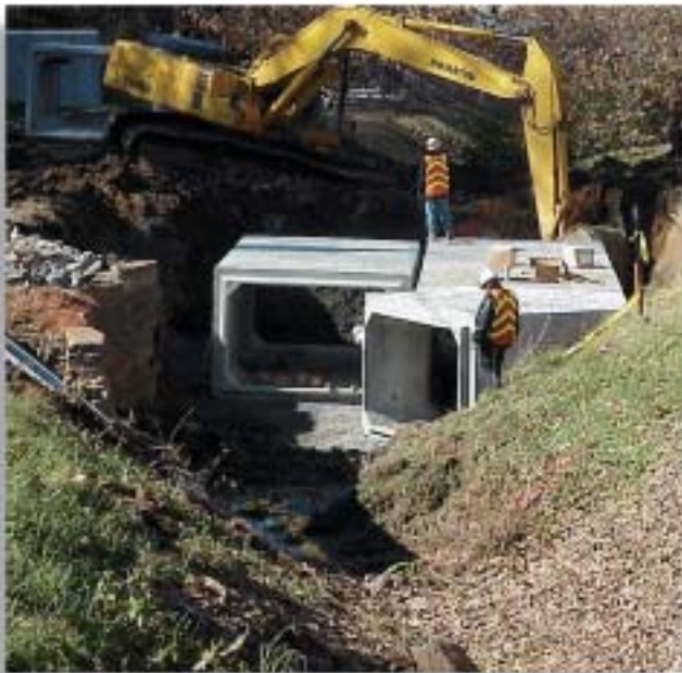
The final layout included two parallel lines of 8-foot x 5-foot precast concrete box sections.
