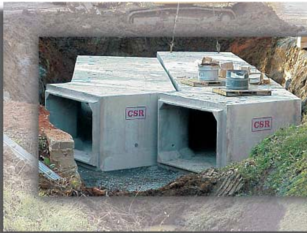
Horizontal bend precast concrete box sections allow the drainage system to follow the existing drainage course along Sedley Road in Charlotte, N.C.
