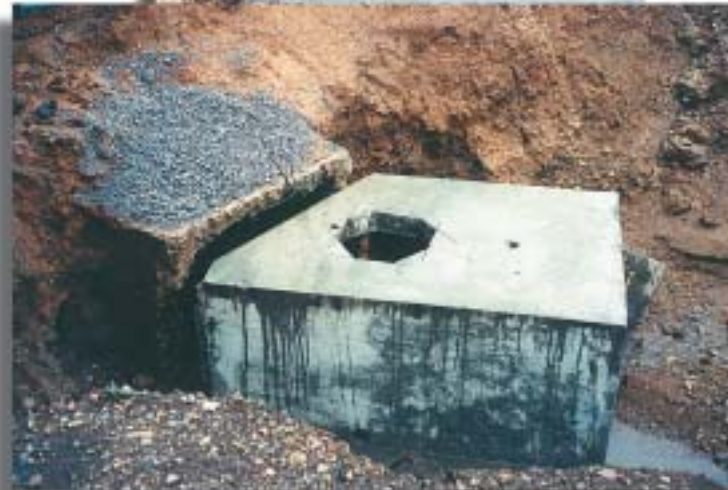
◀ New precast box section cut on site to fit existing structure and accommodate storm sewer pipe.
