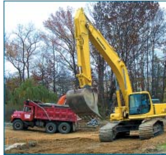
The contractor worked quickly to replace the failed CMP with precast concrete pipe.
