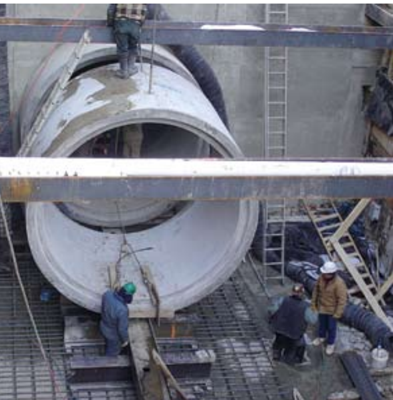
A 150-ton Linkbelt crane was used to lower the 34-ton pipe through the cross bracing.
