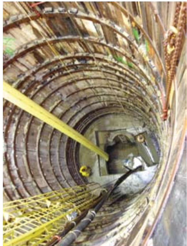
Shaft drilled to access a tunnel crown to connect bypass pressure pipelines.
