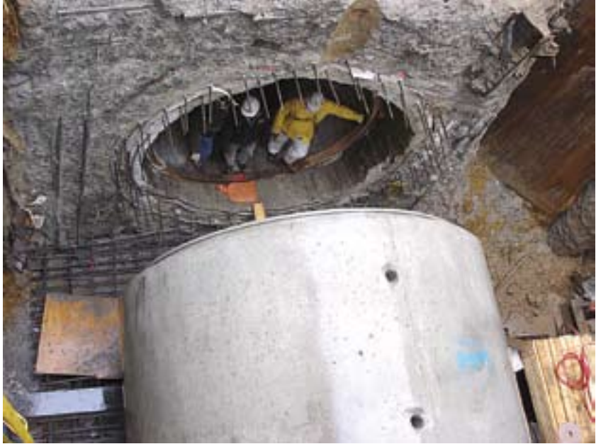
Installation of 132-inch diameter Class V RCP to connect with existing tunnel fitted with steel doweled pins to facilitate the connection.
