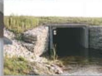
...and provide an attractive and structurally sound culvert solution under the TransCanada highway.
