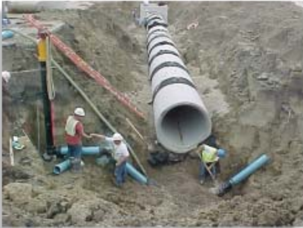
Fire hydrants are lowered into the trench for connection while work on the water, sanitary sewers and storm drain continued.
