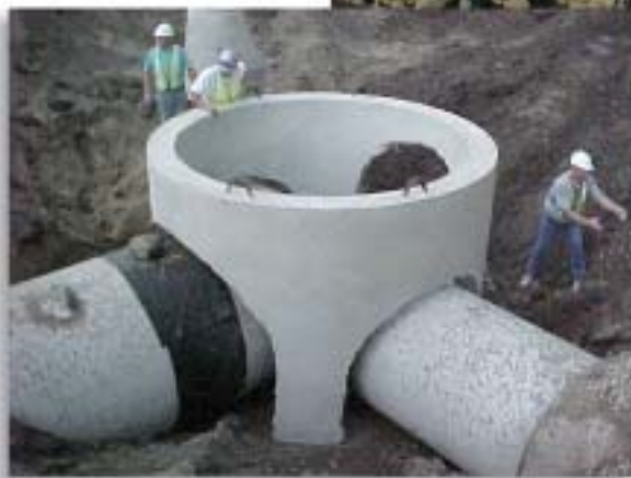
Several multi-inlet precast structures were fabricated by North Dakota Concrete Products Company for the South Broadway project.
