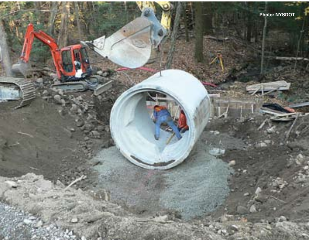
60-inch diameter RCP with dissipater baffles.
