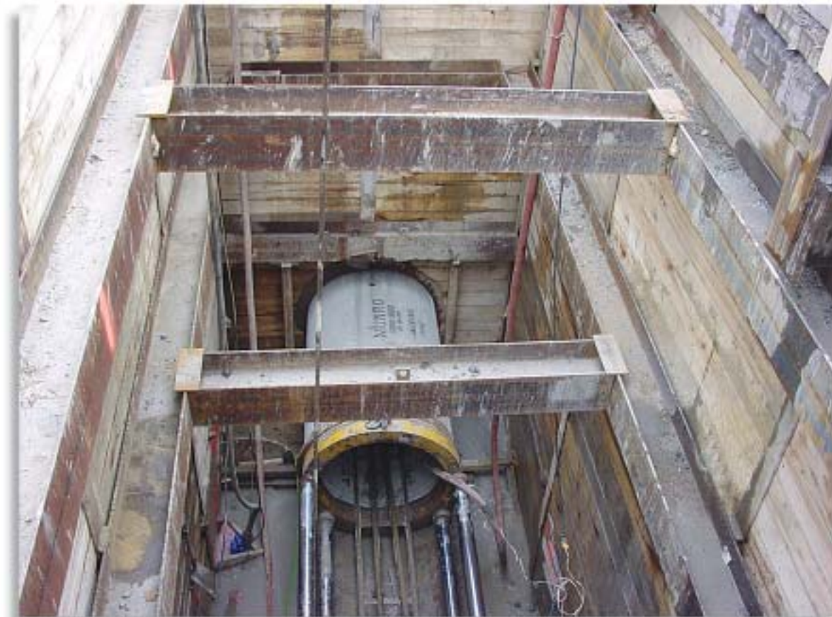
Two different jacking contractors, working from two locations, enabled Toronto's Works and Emergency Technical Services Department to complete the 1200 mm, 100 D (48-inch diameter Class IV) jacking project in only 90 days.
