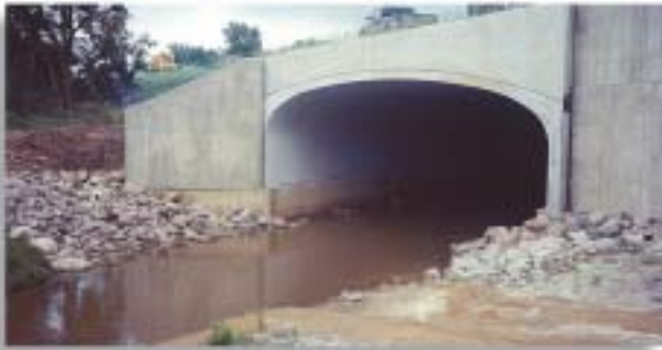
The M-6/US-131 Interchange project included the use of a CON/SPAN® bridge system crossing over Buck Creek.
