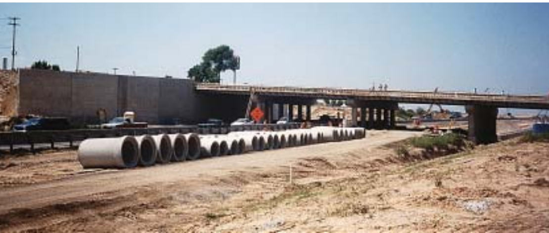
The scope of the M-6/US-131 Interchange project includes over 4-1/2 miles of precast concrete pipe, 600 drainage structures, 28 new bridges and 14 new ramps.
