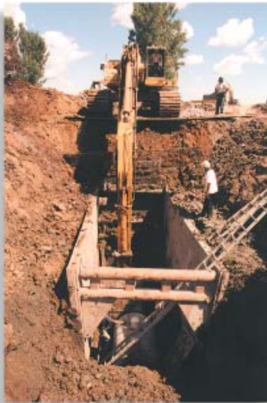
6,900 meters (22,638 feet) of precast reinforced concrete pipe was used for the Matte Collector System. The line was designed to accommodate flows from sub-basins.
