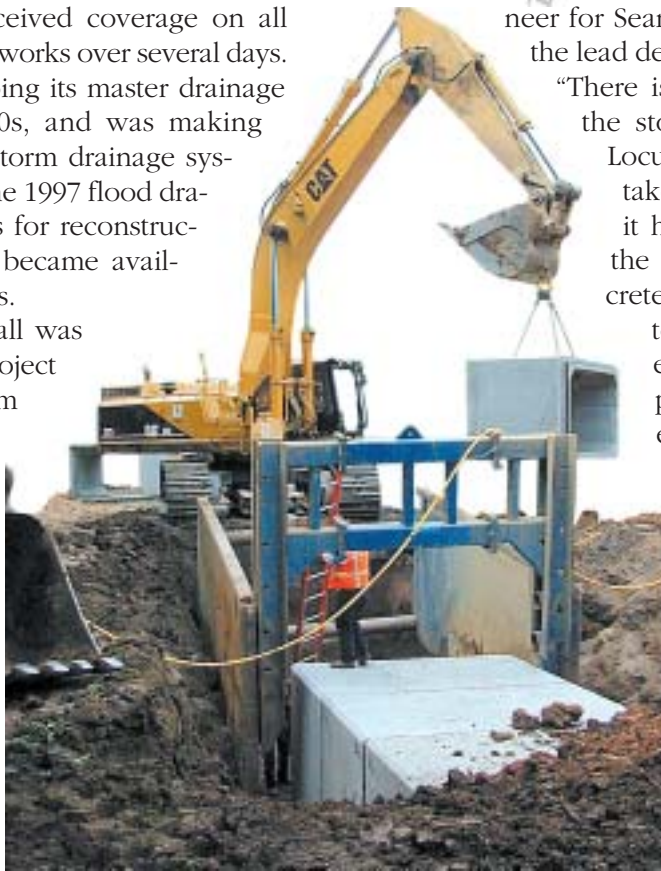
The trench box used during installation of 8-ft. x 5-ft. reinforced concrete box sections allowed for smaller excavation and minimized site problems from wet weather runoff.
