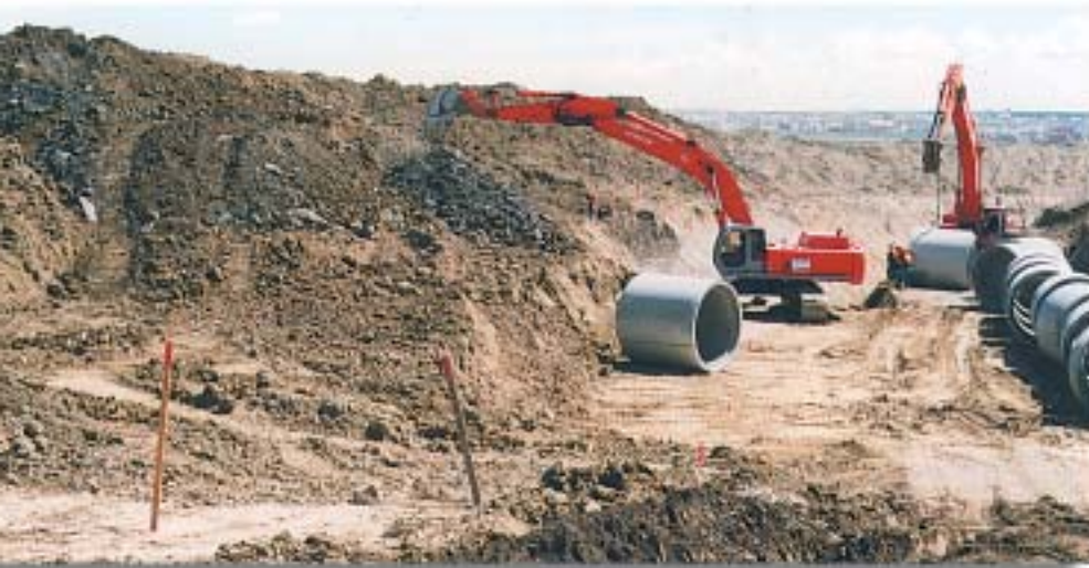
Installation of 516 meters (1,693 feet) of 2100-mm (84-inch) diameter RCP at Country Hills Town Centre, Calgary.
