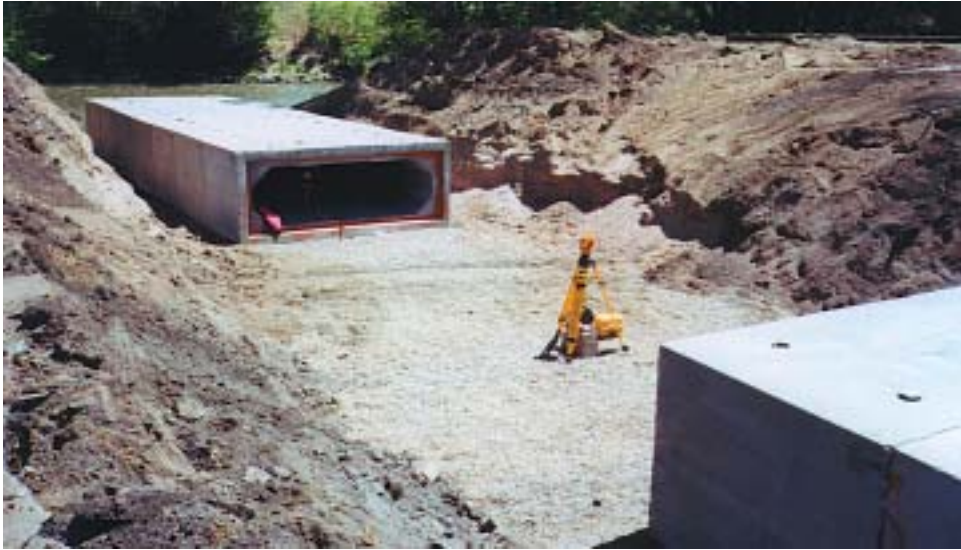
Lasers were used to align 10-foot x 3-foot reinforced concrete box culvert sections. The RCBC line will discharge storm water runoff into the South Platte River.
