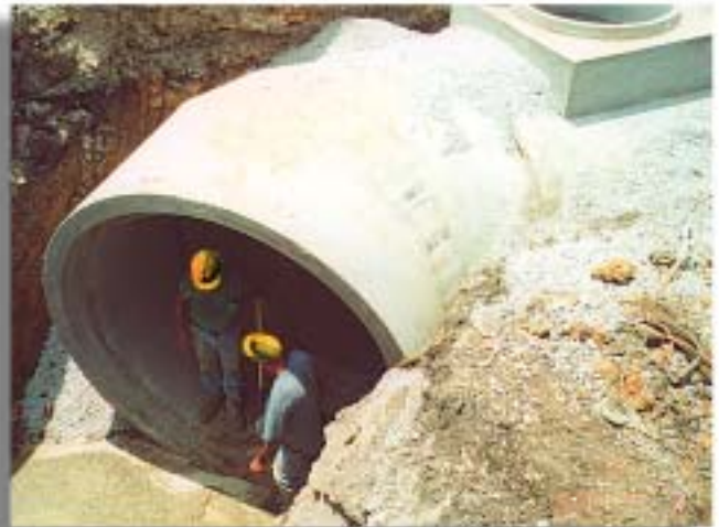
45 degree bends and saddle tees were used to overcome site restrictions for the RCP storm water detention facility.
