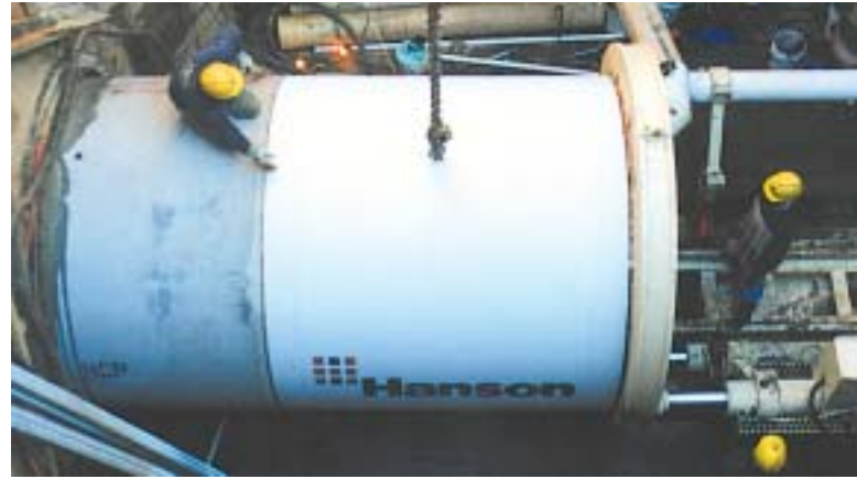
Only two 30-foot diameter jacking pits were required to install 1,300 feet of 84-inch reinforced concrete pipe.
