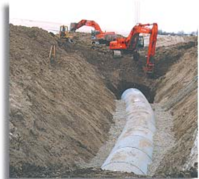
Standard installations helped the developer save $250,000 at Country Hills Town Centre in Calgary, Alberta.
