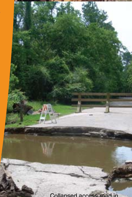
Collapsed access road in River Grove Park, Kingwood. Photo: Hanson Pipe & Precast
