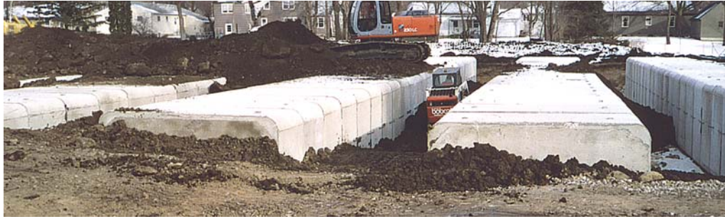
Five parallel lines of 12-foot x 8-foot precast concrete box sections used for stormwater detention under parking lot and lawn.
