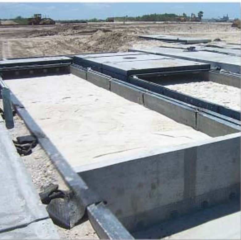
Three-sided boxes designed to hold a special sand media filter.
