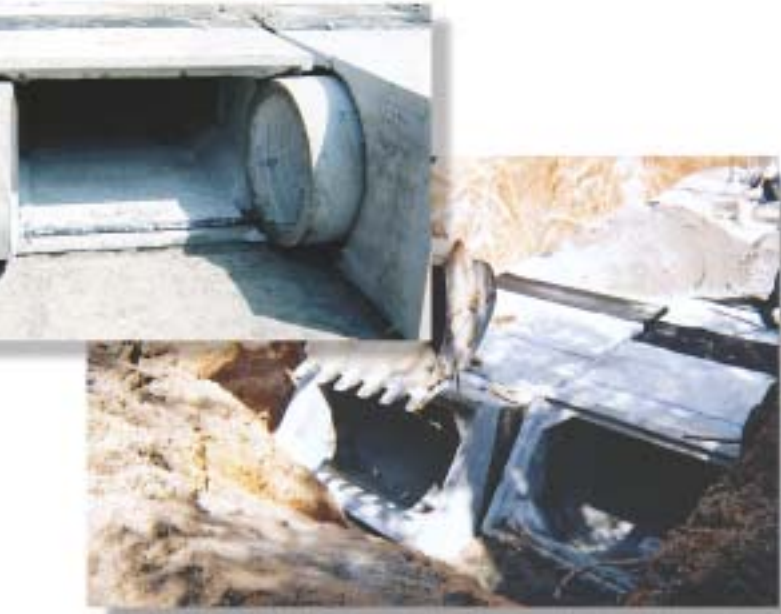
Installation of precast concrete box culverts with 54-inch diameter reinforced concrete pipe equalizer.
