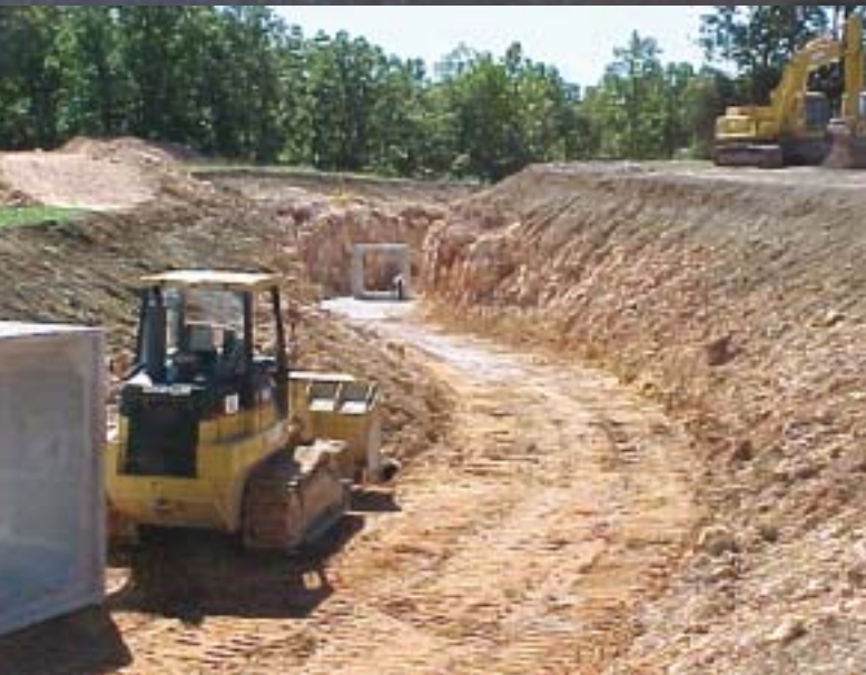
The tunnel sections had to be cut and blasted through rock to maintain the level grade for the train and rail system.
