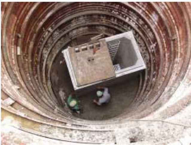
Assembly of 96-inch x 48-inch transition riser with specially designed elliptical pipe connection.
