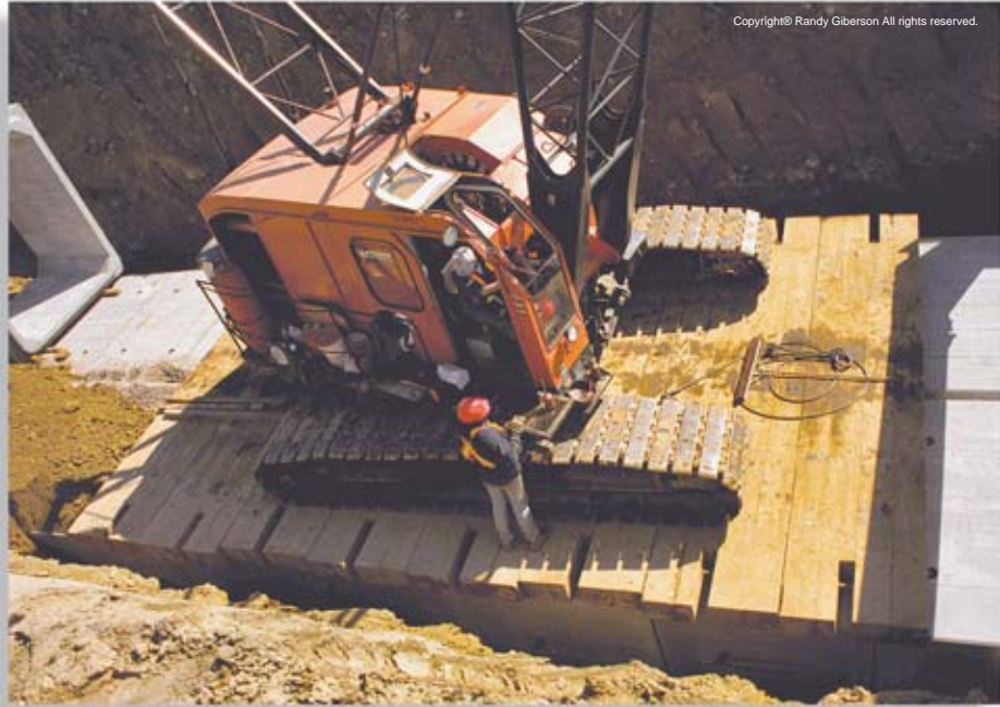
Boxes designed to support weight of crane as well as backfill material.
