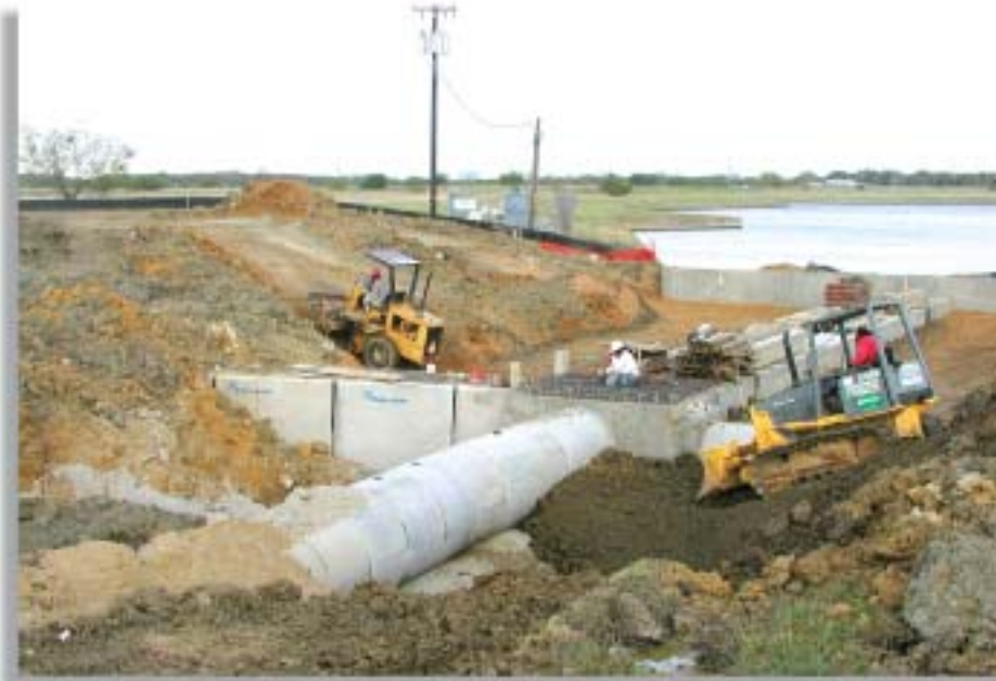
Box storm sewer also serves as a cross culvert beneath the extension of Las Colinas Boulevard.
