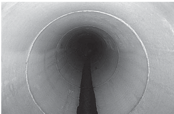
RCP Pipe Installed in 1987
