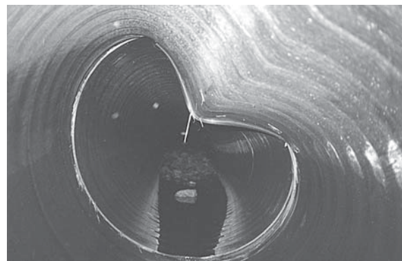
HDPE Pipe Installed in 1997
