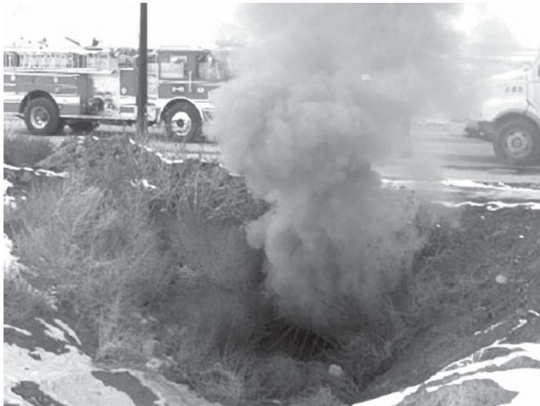
Smoke pours out of 42" HDPE storm drain after catching fire.
