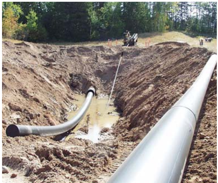
The failed HDPE pipeline at Shell Lake is now being slip lined with another pipe product to help alleviate flooding problems for residents ... finally.
