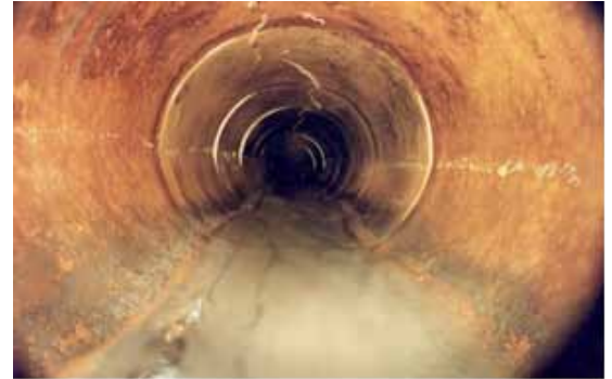
RCP exhibiting a crack with vertical offset in obvert (Top) of pipe
