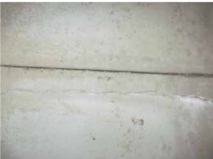
Small crack near joint.
