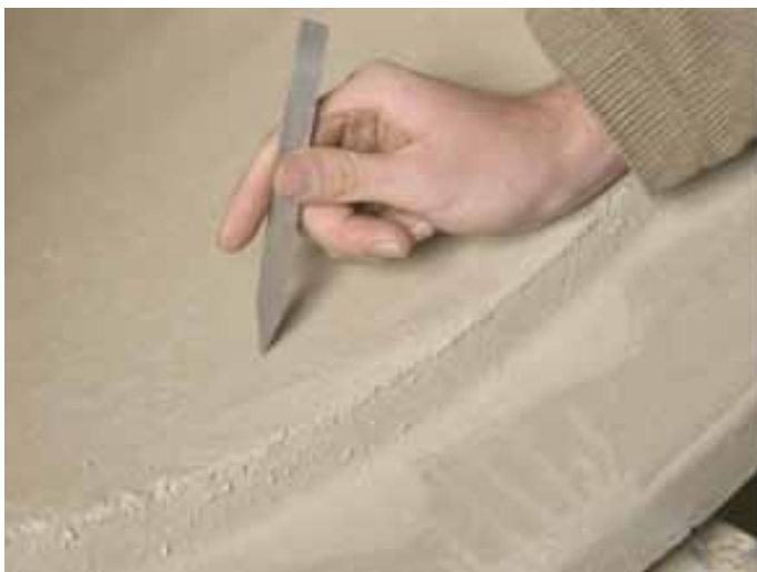
Measurement of crack with feeler gauge.
