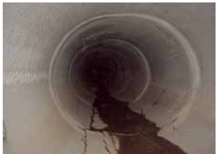
Interior view of RCP with cracks in haunch area with vertical offset. Early sign of possible slabbing and radial tension shear forces present in wall of pipe.
