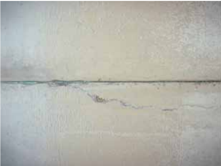
Crack near joint of RCP.
