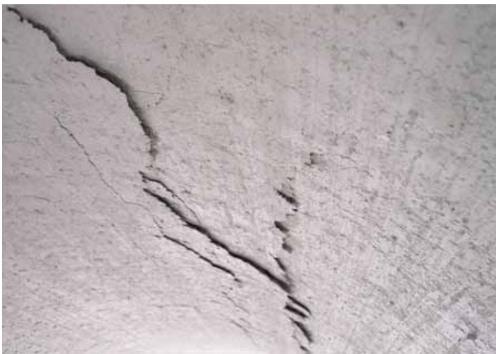
Crack with vertical offset – early indication of possible radial tension shear in pipe wall.
