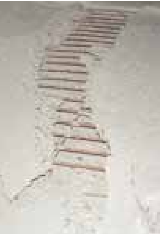
Concrete slabbing near invert due to radial tension shear.
