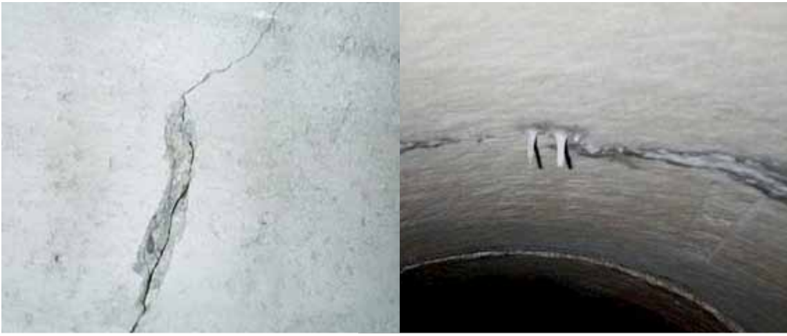
Circumferential Crack with minor spalling along crack & circumferential crack with autogeneous healing.
