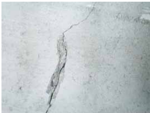
Crack exhibiting minor spalling along edge of crack.
