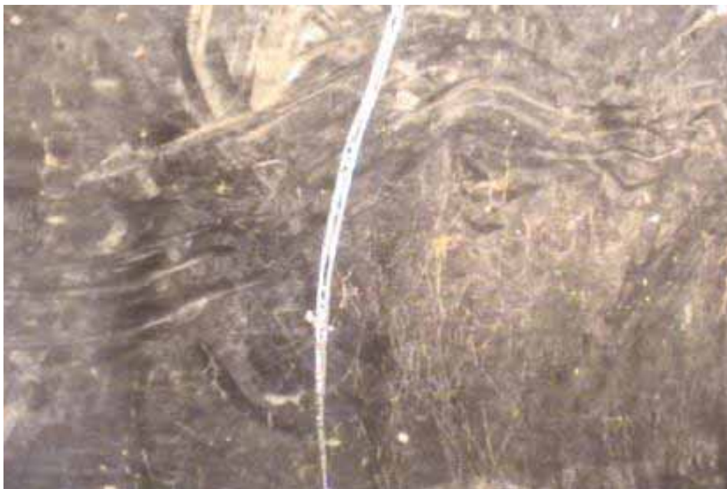
Figure 282 Cracking/fracture failure for Pipeline No. 5 (Site No. 1: Route 101)
