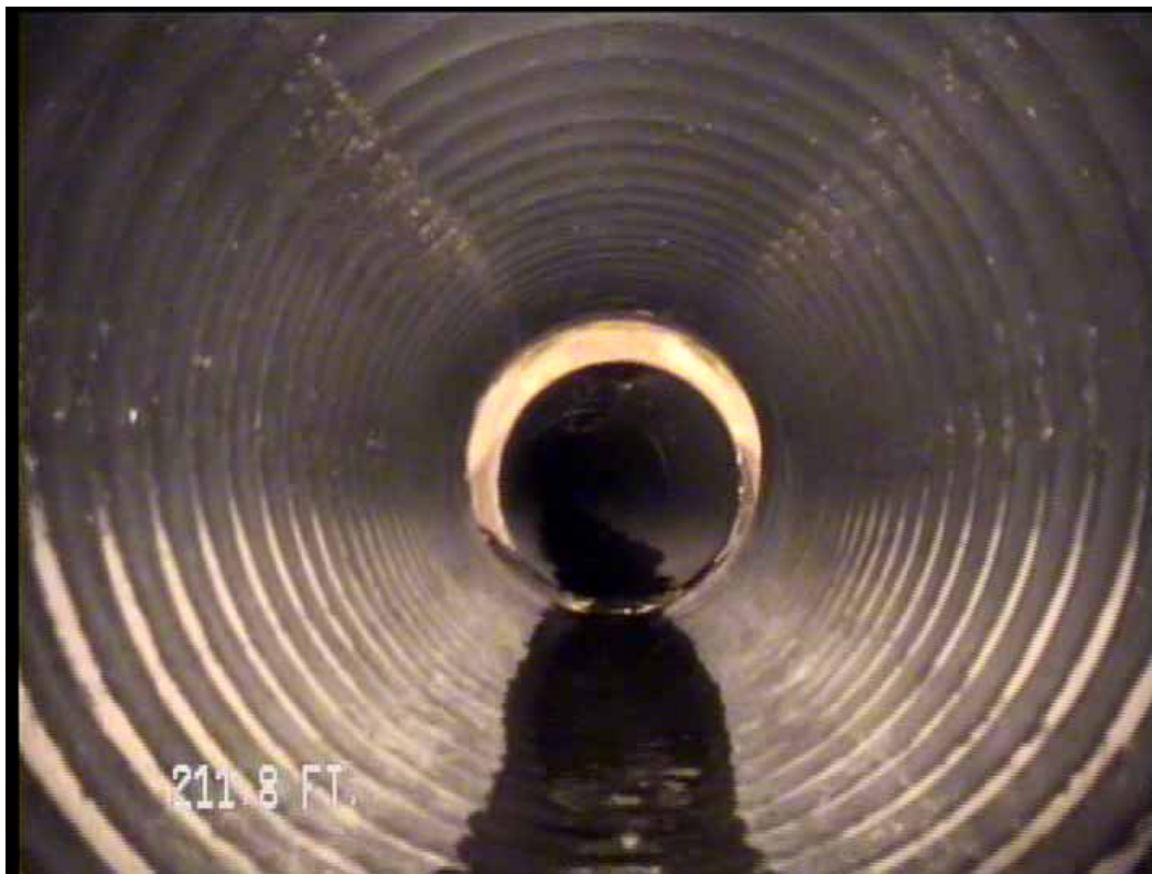
Figure 497 View of the corrugation growth failure for pipeline No. 3 (Site No. 1: Orlando)
