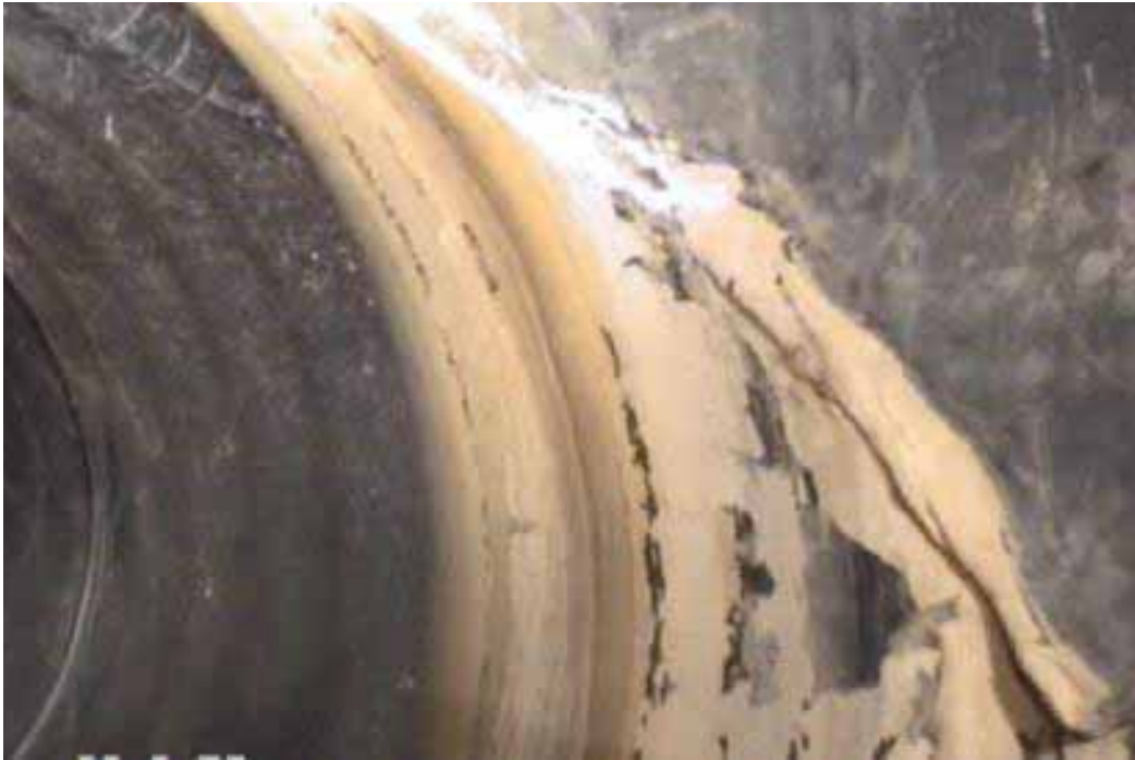
Figure 279 Cracking/fracture failure for Pipeline No. 5 (Site No. 1: Route 101)
