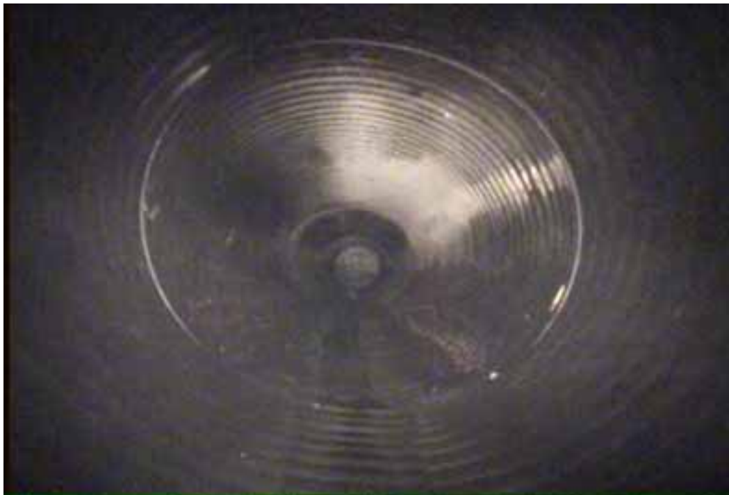
Figure 137 View of excessive deformation failure for pipeline No. 10 (Site No. 5: Staunton)
