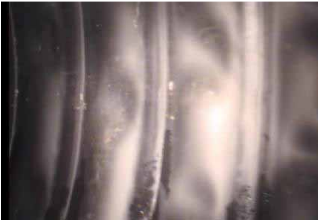
Figure 215 View of the buckling failure for pipeline No. 5 (Site No. 1: Lenexa)
