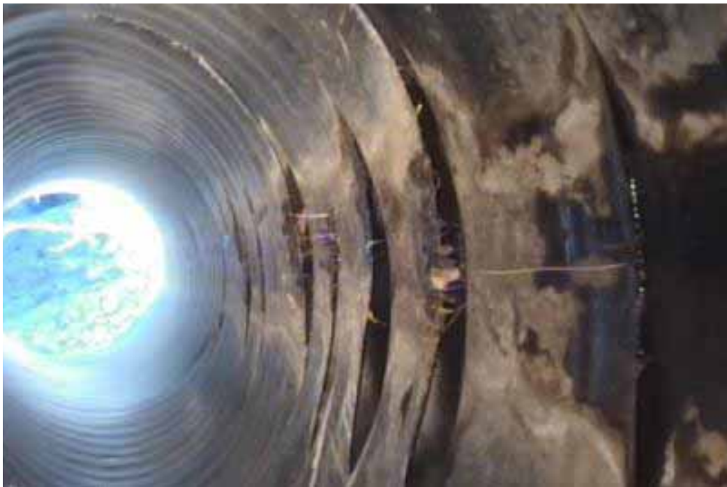
Figure 267 Corrugation growth and cracking/fracture failures for Pipeline No. 2 (Site No. 1: Route 101)
