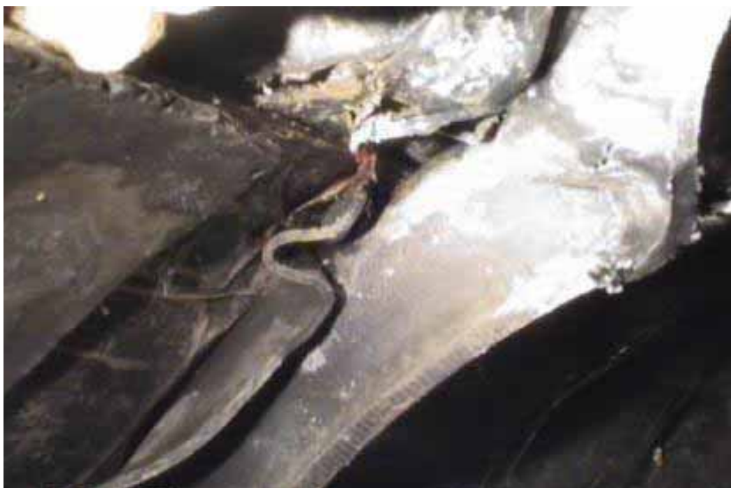
Figure 264 Cracking/fracture failures for Pipeline No. 2 (Site No. 1: Route 101)
