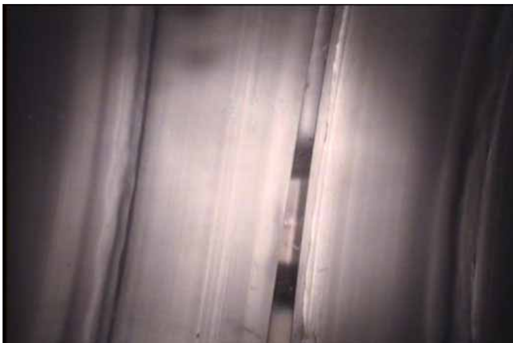
Figure 192 View of joint displacement failure for pipeline No. 27 (Site No. 8: Fairmont)
