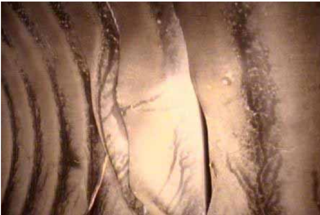
Figure 466 Cracking/fracture, buckling, and corrugation growth failure for Pipeline No. 24b (Site No. 13: Burlinghame Avenue)
