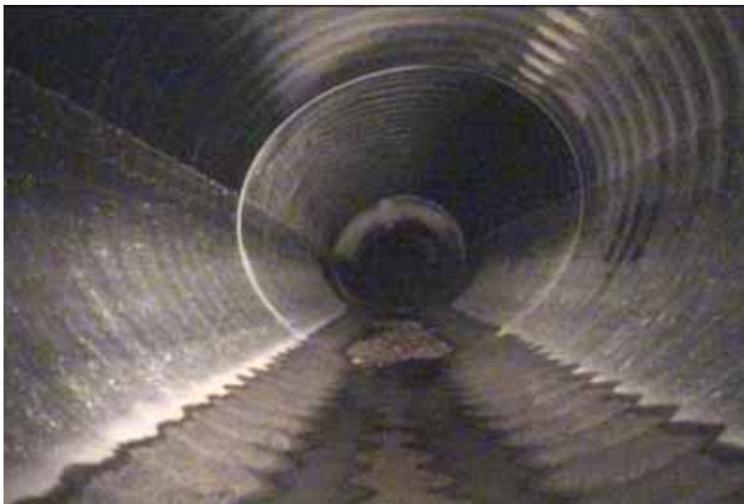
Figure 112 View of the excessive deformation failure for pipeline No. 2 (Site No. 1: Chesterfield - Commonwealth Pkwy)
