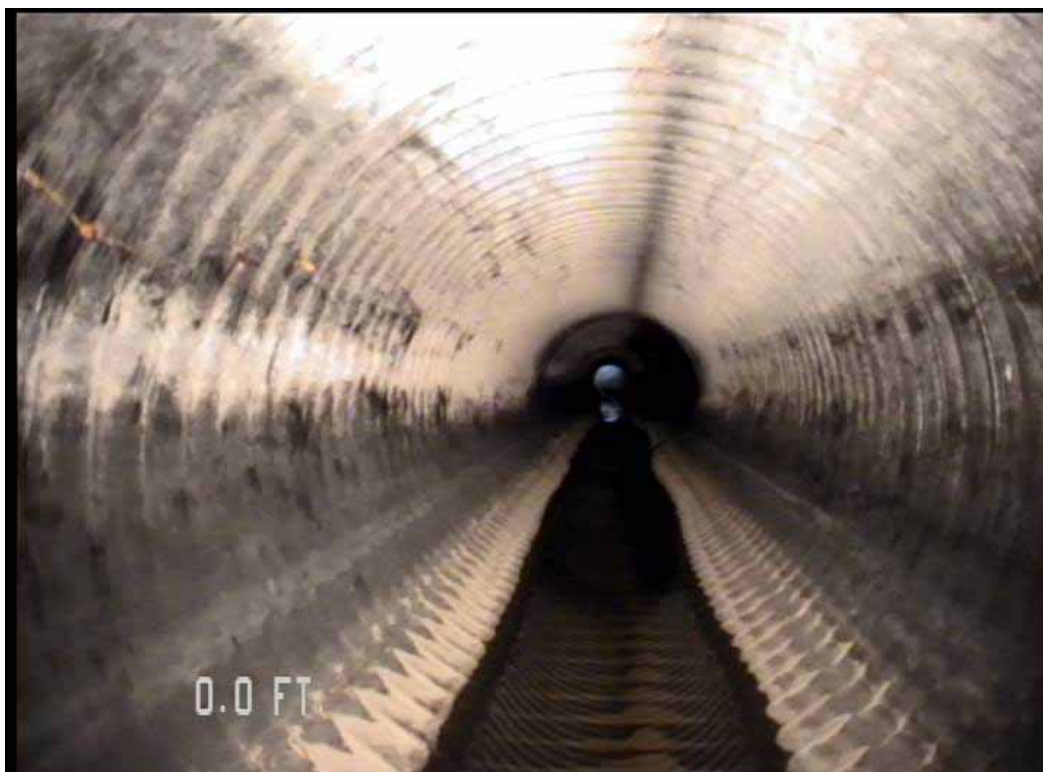
Figure 562 View of corrugation growth failure at the opening for pipeline No. 12 (Site No. 2: Apopka)
