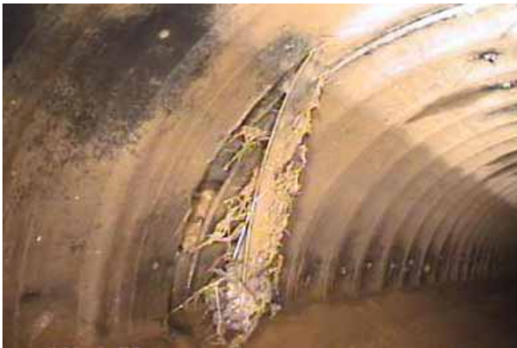
Figure 416 Cracking/fracture, major joint displacement, and corrugation growth failure for Pipeline No. 7 (Site No. 7: West Island Road)
