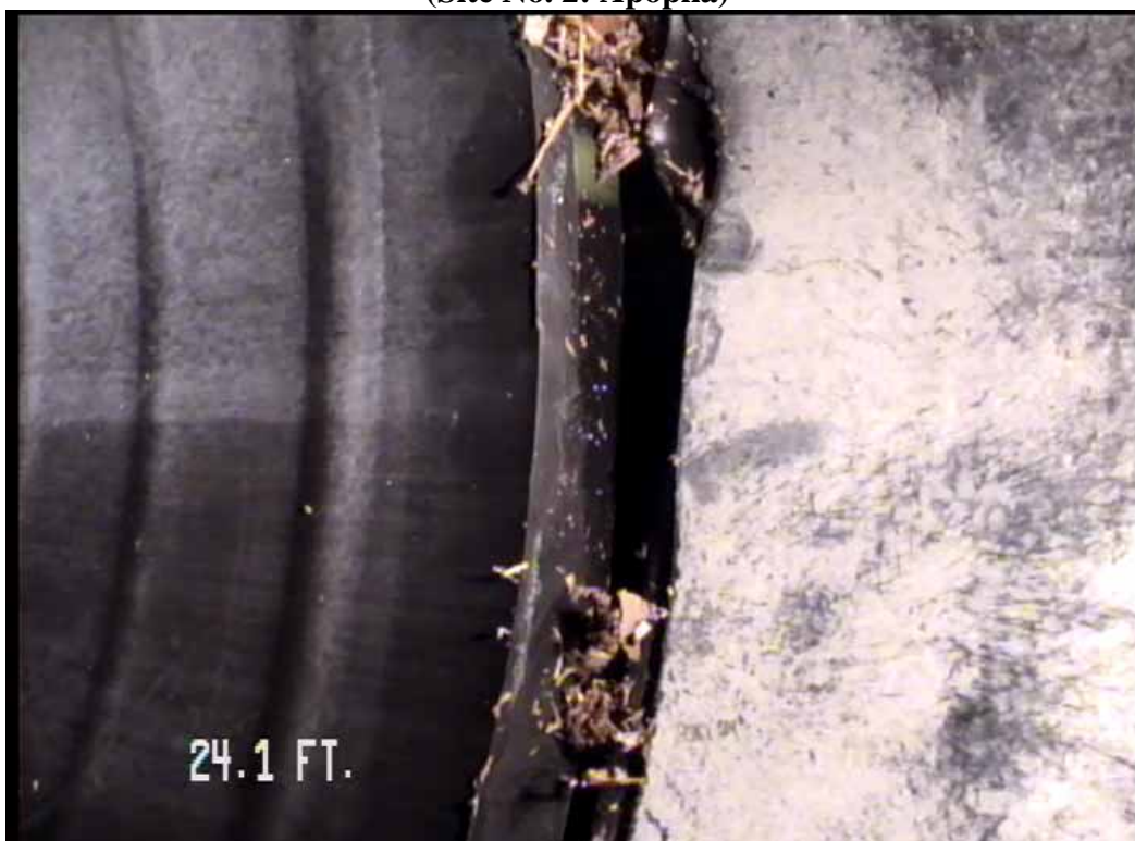
Figure 554 View of the major joint displacement/crack/fracture failures for pipeline No. 11 (Site No. 2: Apopka)
