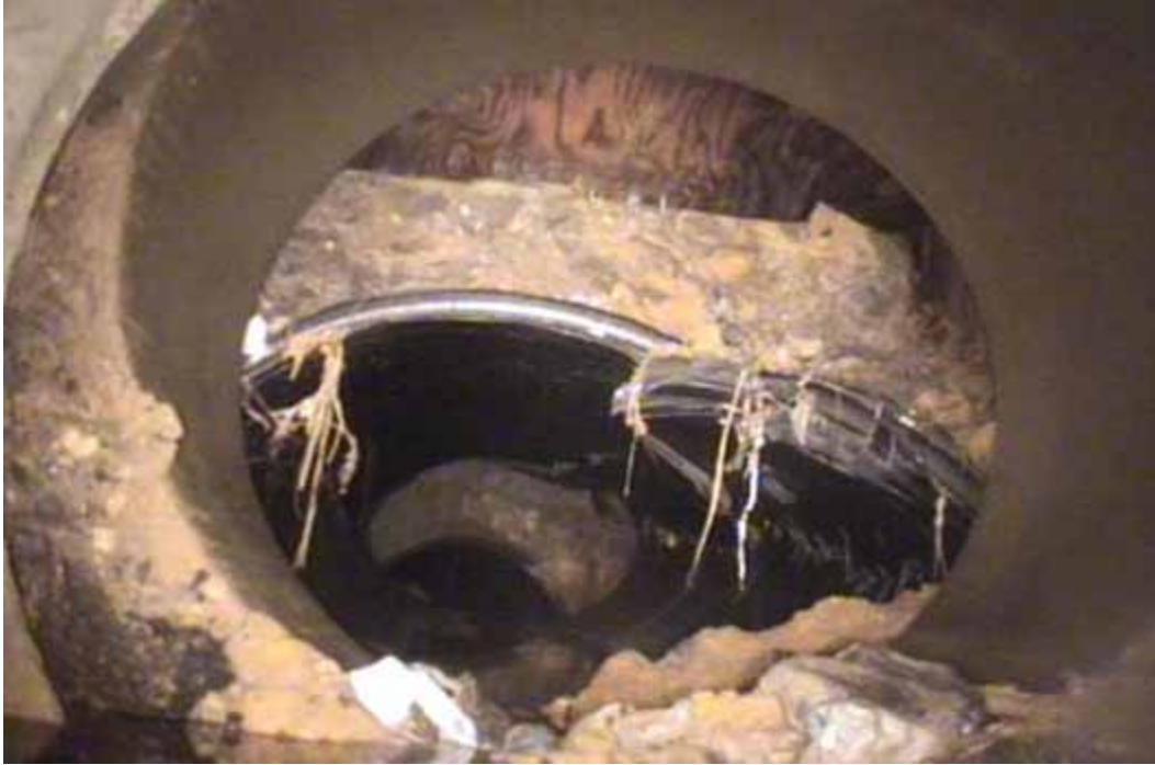
Figure 56 Major cracking/fracture, minor cracking/fracture, and inverse curvature failures for pipeline No. 20 (Segment 2) (Site No. 8: Houston – Fennell)
