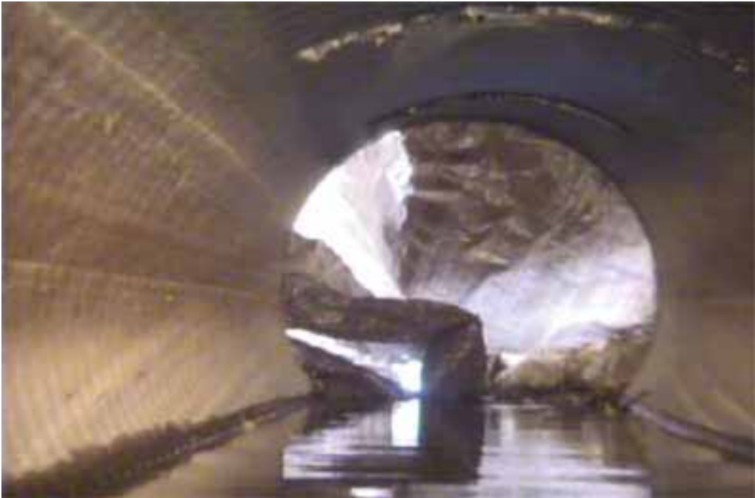
Figure 68 View of cracking failure for pipeline No. 5 (Site No. 2: Elm City – Lake Wilson Rd)
