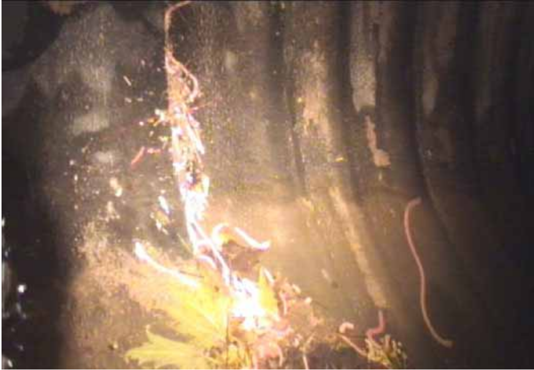
Figure 164 View of the major joint displacement failure for pipeline No. 5 (Site No. 2: Brooklyn Park - 71st Ave)
