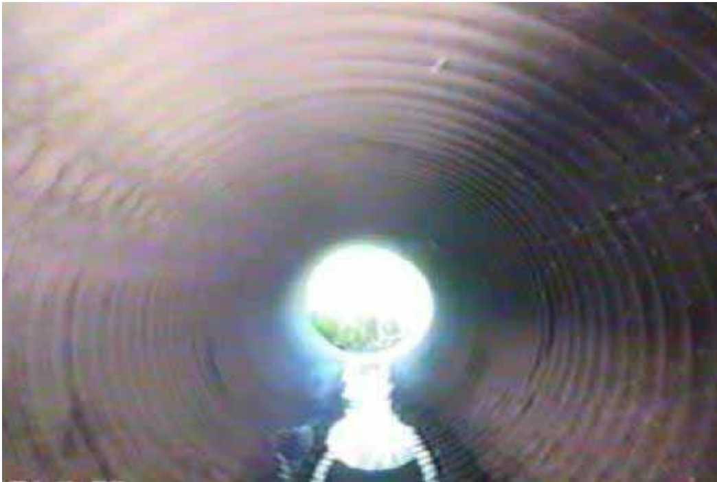
Figure 358 Corrugation growth and excessive deformation (refer to Figure 357-d) failure for Pipeline No. 1 (Site No. 1: Legacy Parkway)
