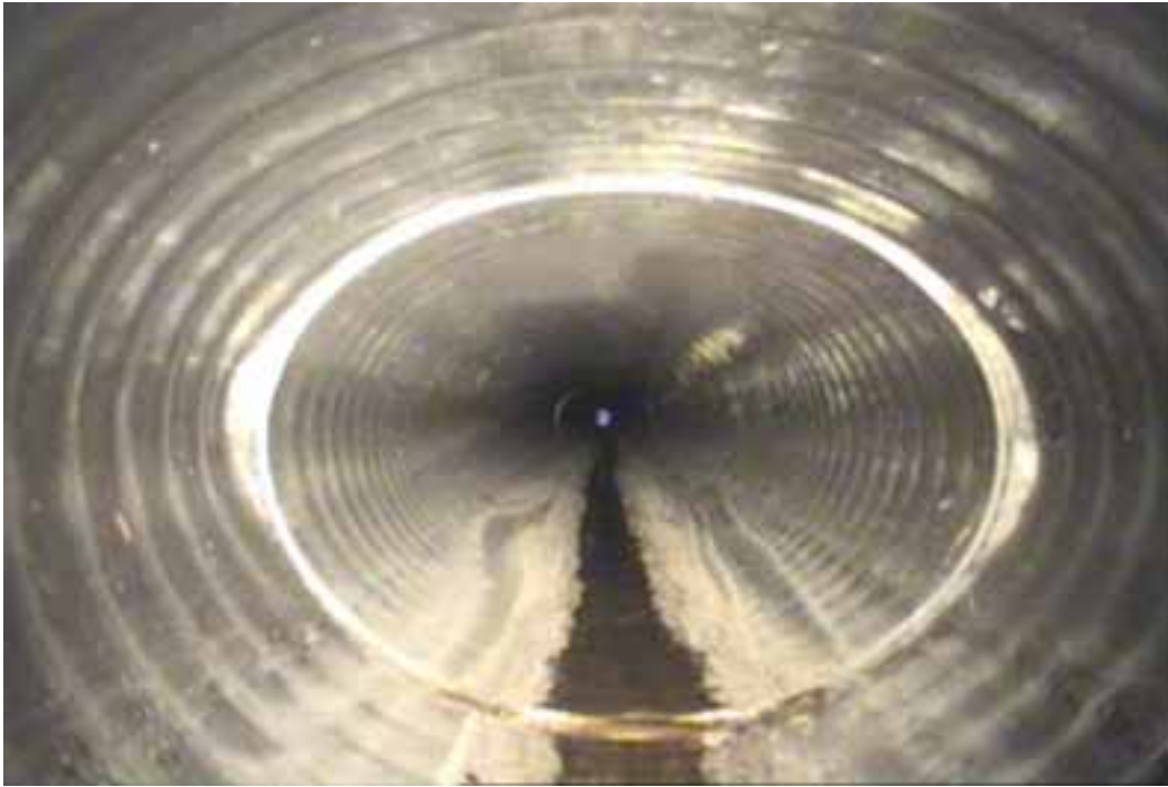
Figure 132 View of excessive deformation and corrugation growth failures for pipeline No. 8 (Site No. 4: Mechanicsville)
