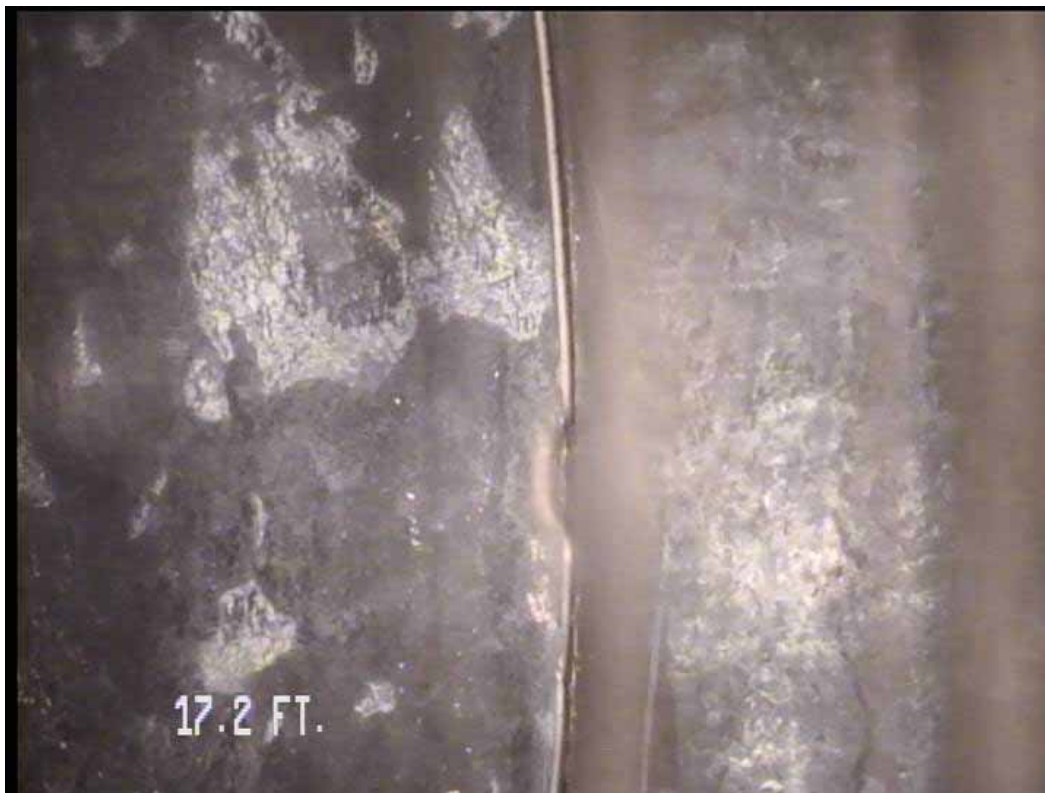
Figure 567 View of buckling failure at the joint for pipeline No. 13 (Site No. 2: Apopka)
