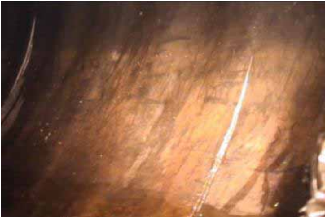
Figure 435 Cracking/fracture failure for Pipeline No. 13 (Site No. 8: Kinross Road)
