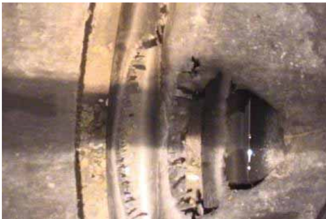
Figure 254 Cracking/fracture failure for Pipeline No. 1 (Site No. 1: Route 101)
