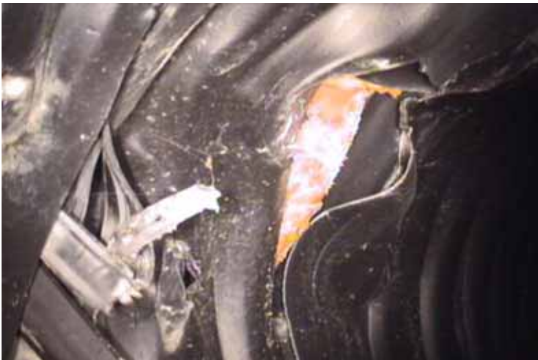
Figure 128 View of cracking/fracture failure for pipeline No. 6 (Site No. 4: Mechanicsville)
