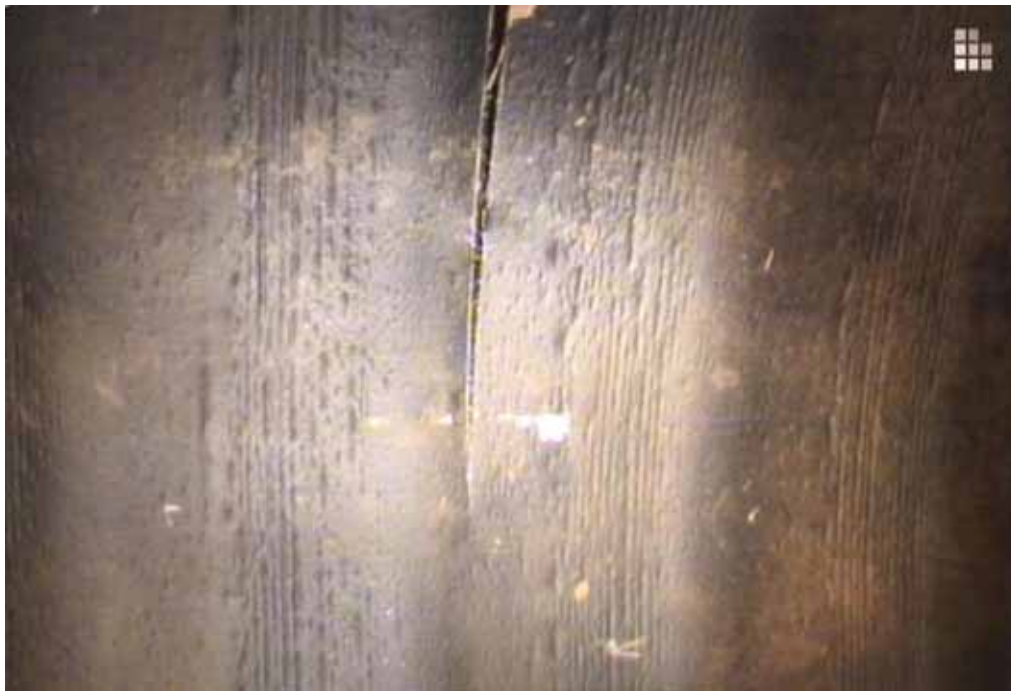
Figure 173 View of cracking/fracture failure for pipeline No. 15 (Site No. 5: McGregor)
