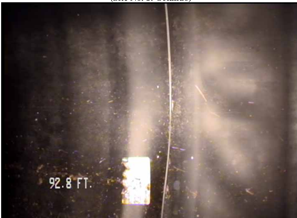
Figure 518 View of the buckling failures for pipeline No. 7 (Site No. 1: Orlando)
