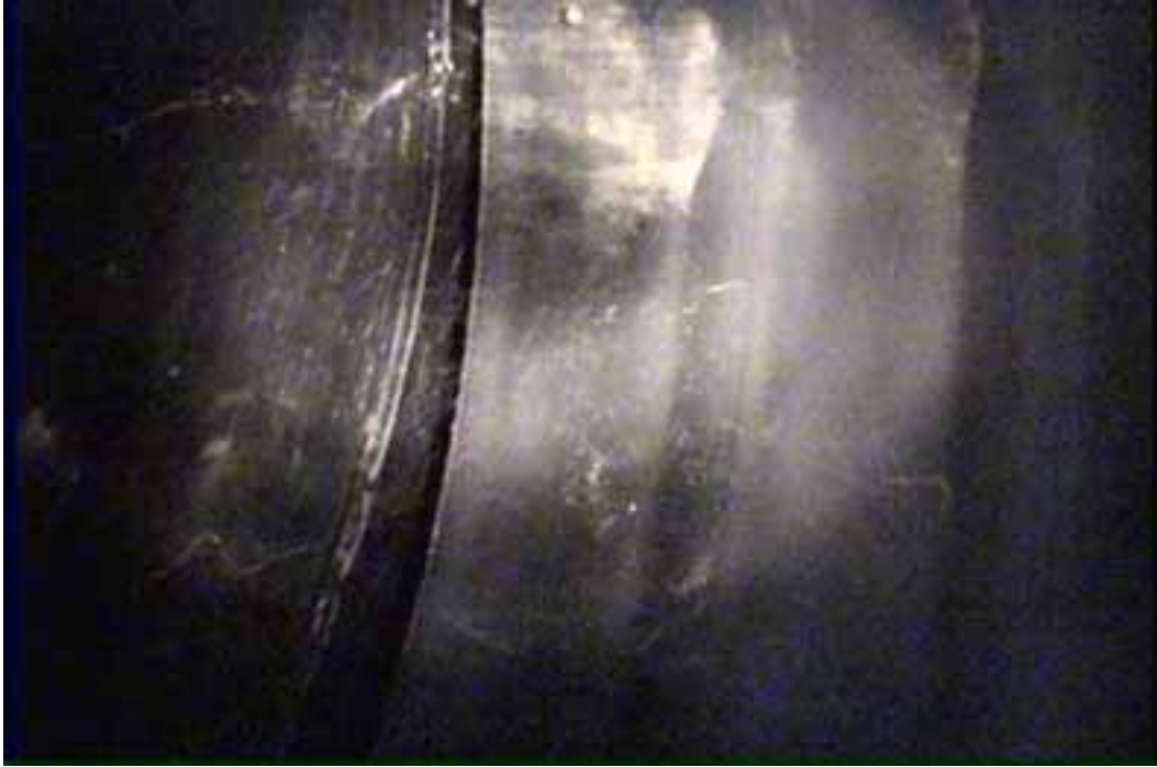
Figure 153 View of joint displacement failure for pipeline No. 18 (Site No. 6: Winchester)
