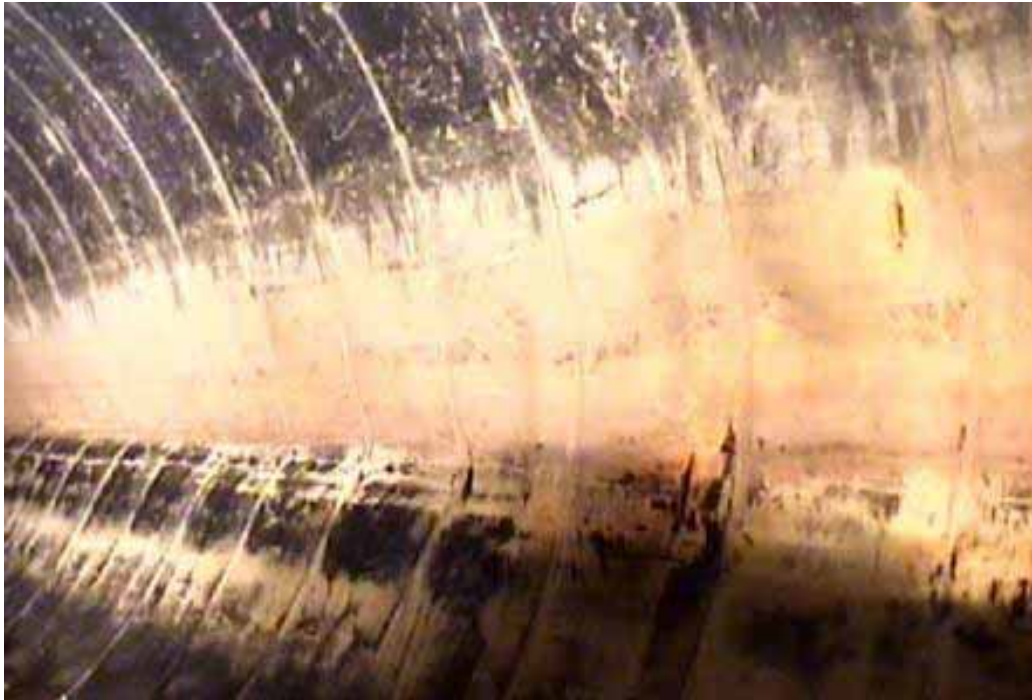
Figure 458 Buckling and corrugation growth failure for Pipeline No. 23 (Site No. 12: 48 th Avenue)
