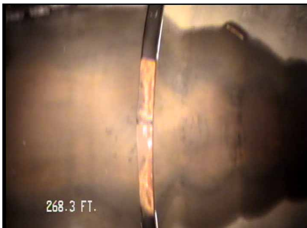
Figure 570 View of the major joint displacement failure for pipeline No. 13 (Site No. 2: Apopka)
