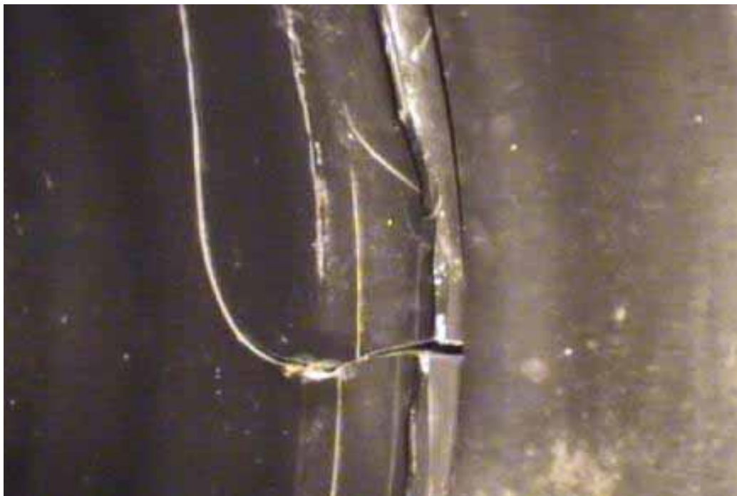
Figure 402 Cracking/fracture and major joint failure for Pipeline No. 5 (Site No. 5: Bad Axe)
