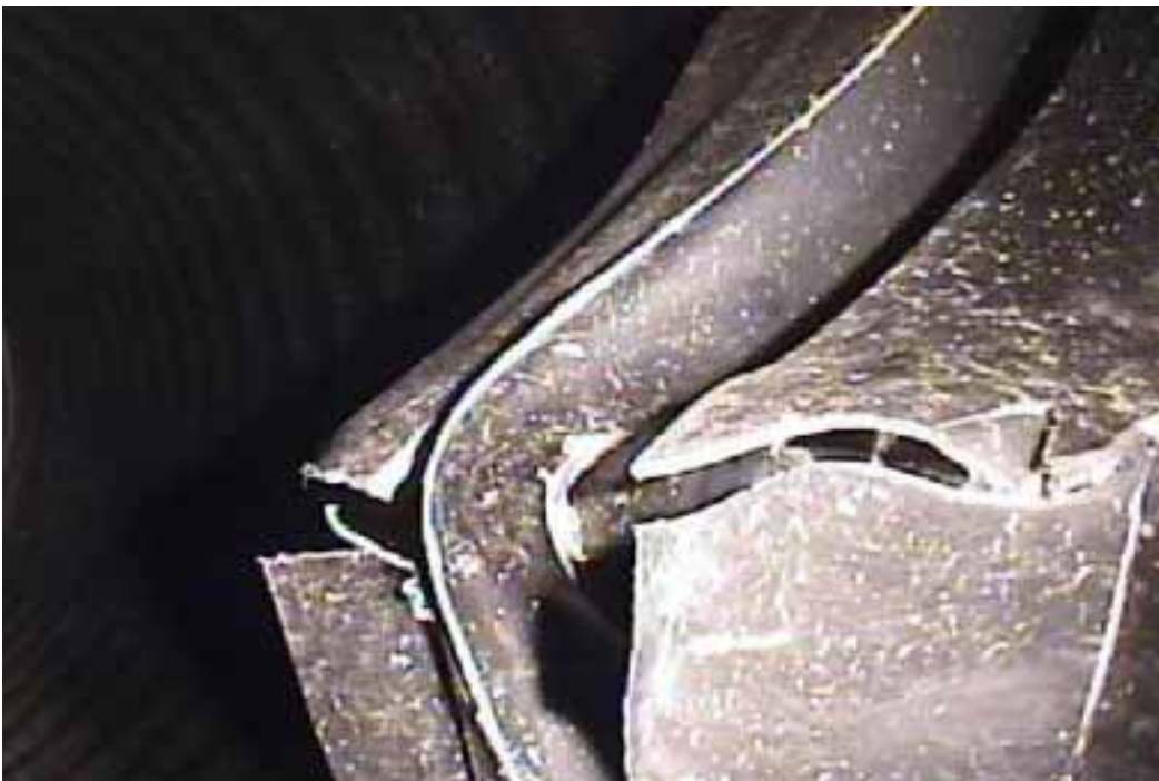
Figure 384 Cracking/fracture and inverse curvature failure from Figure 383 above for Pipeline No. 9 (Site No. 2: Silver Creek Parkway)
