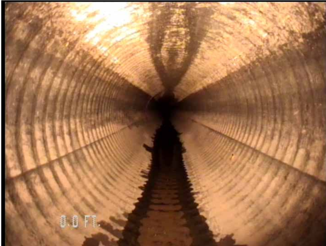
Figure 504 View of the corrugation growth failure for pipeline No. 6 (Site No. 1: Orlando)
