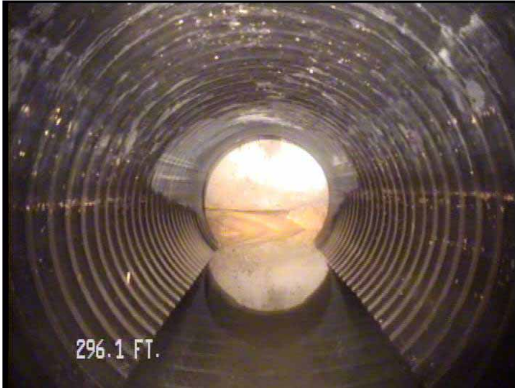
Figure 571 View of the corrugation growth failure at the end for pipeline No. 13 (Site No. 2: Apopka)
