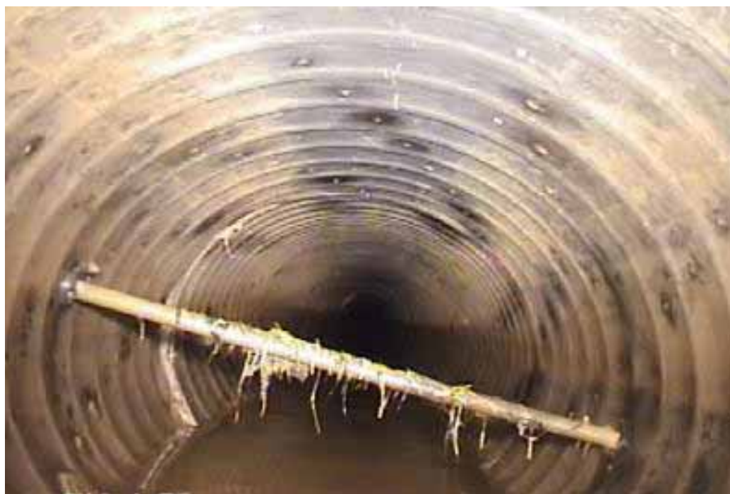
Figure 418 Cracking/fracture and corrugation growth failure for Pipeline No. 7 (Site No. 7: West Island Road)
