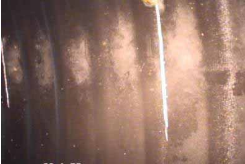
Figure 437 Cracking/fracture and corrugation growth failure for Pipeline No. 13 (Site No. 8: Kinross Road)
