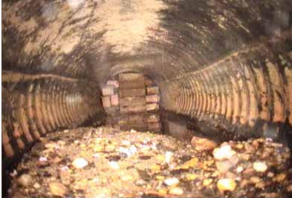
Figure 123 View of corrugation growth failure for pipeline No. 5 (Site No. 3: Spotsylvania County)
