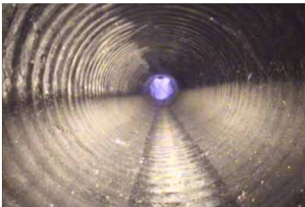
Figure 245 Corrugation growth failure for pipeline No. 11 (Site No. 3: Franklin County – Route FF)
