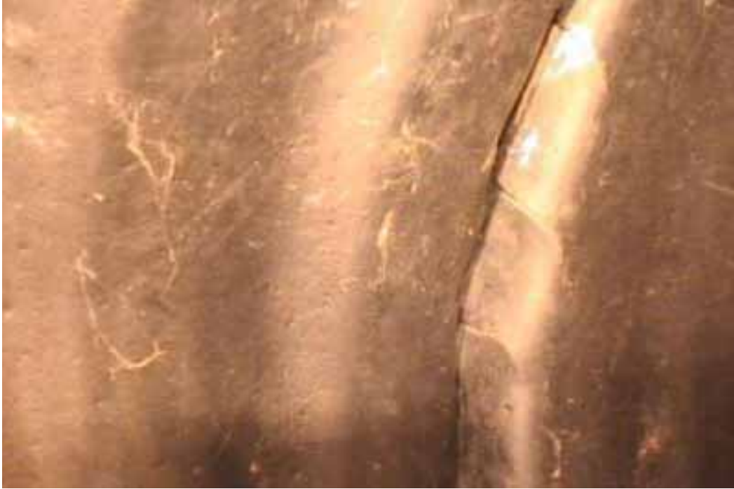
Figure 302 Cracking/fracture failure for Pipeline No. 9 (Site No. 1: Route 101)
