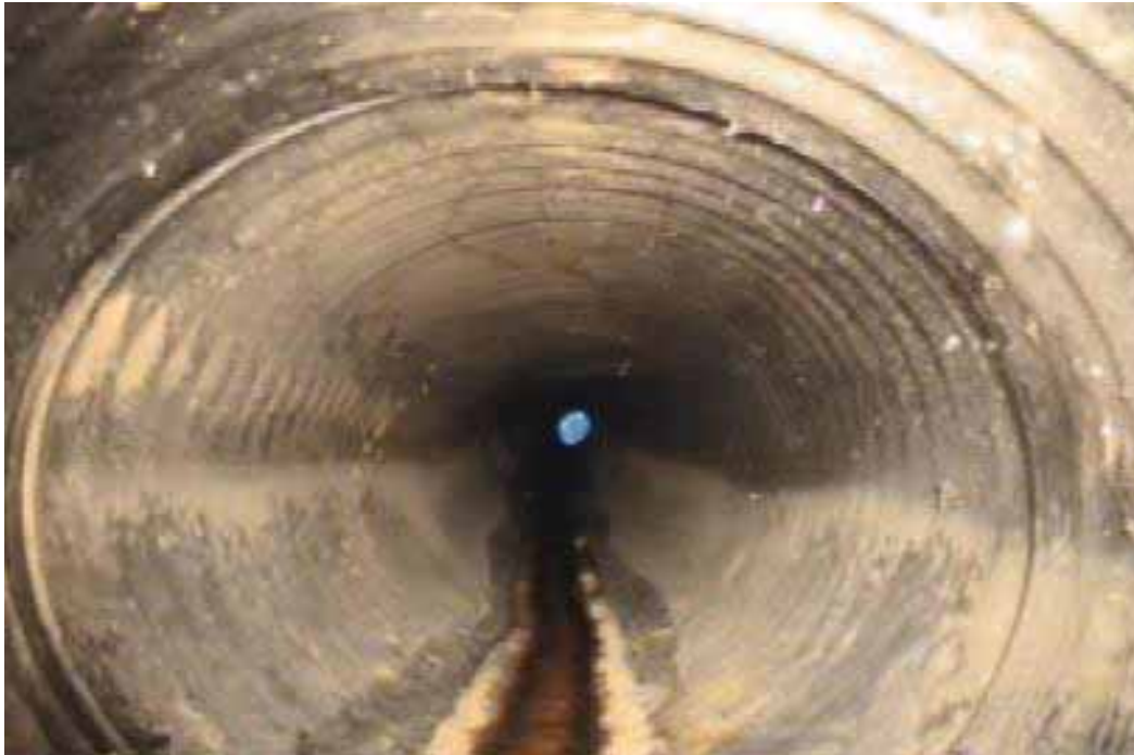
Figure 295 Corrugation growth failure for Pipeline No. 8 (Site No. 1: Route 101)
