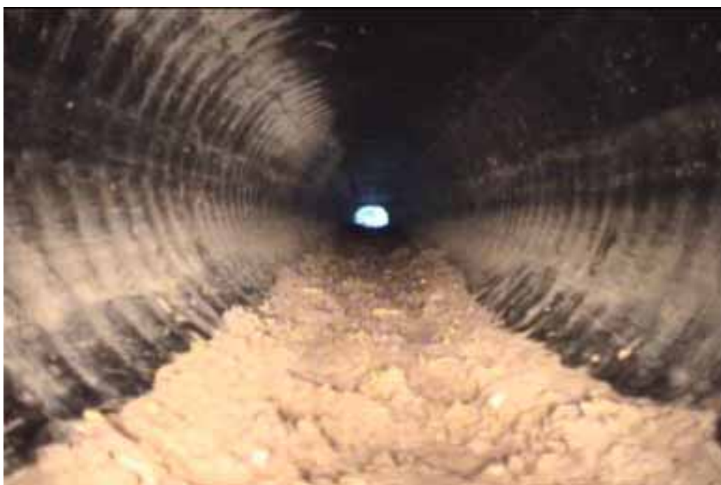
Figure 242 Corrugation growth for pipeline No. 10 (Site No. 3: Franklin County – Route FF)
