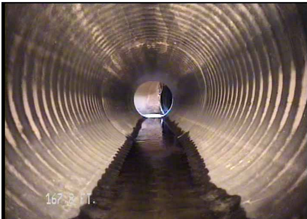
Figure 540 View of corrugation growth failure for pipeline No. 9 (Site No. 1: Orlando)
