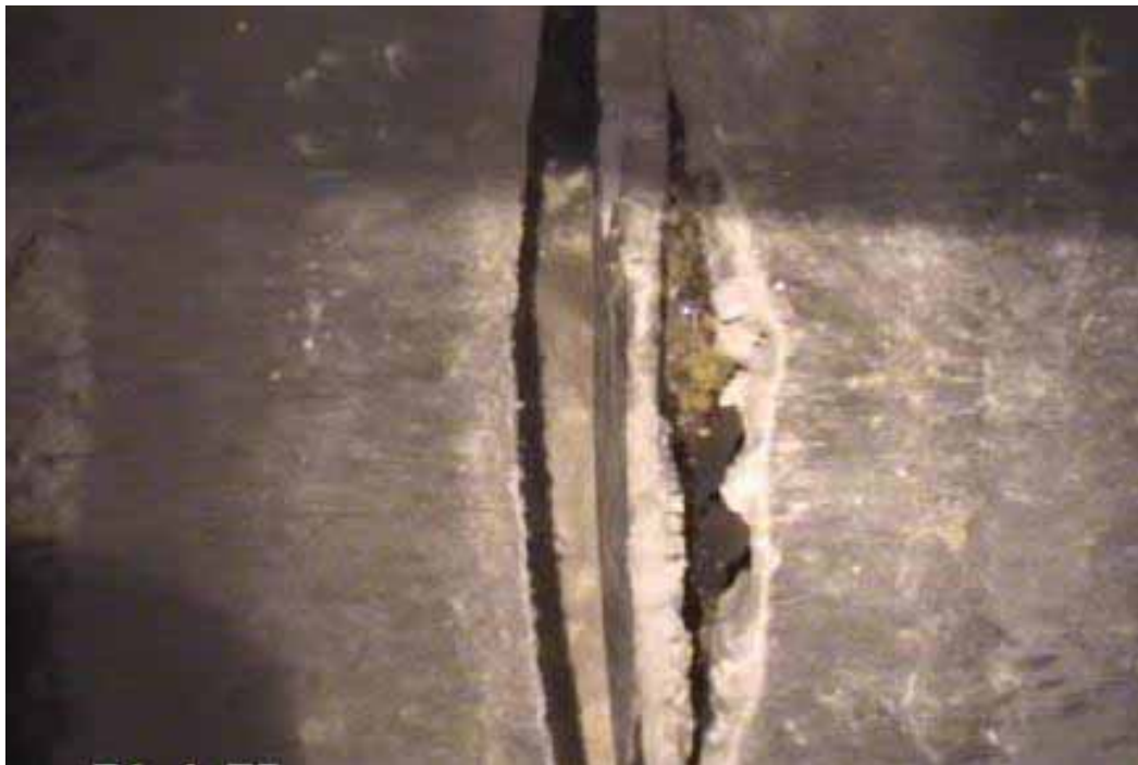
Figure 253 Cracking/fracture failure for Pipeline No. 1 (Site No. 1: Route 101)
