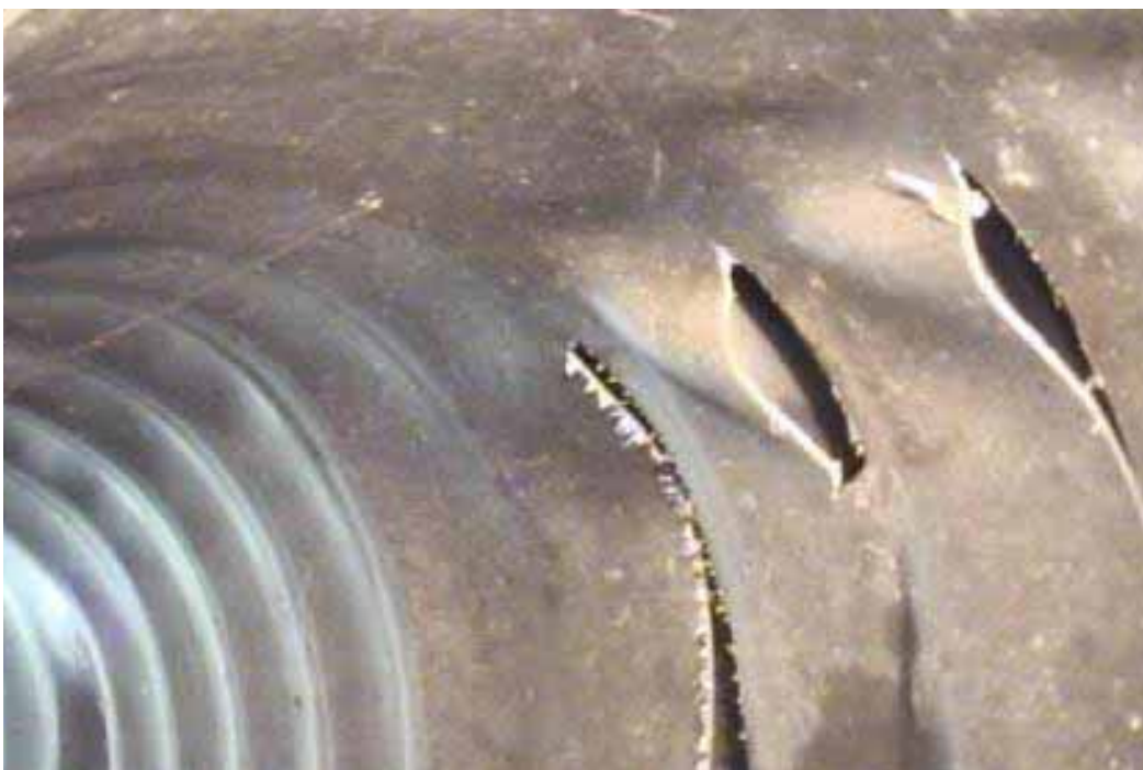
Figure 268 Corrugation growth and cracking/fracture failures for Pipeline No. 2 (Site No. 1: Route 101)
