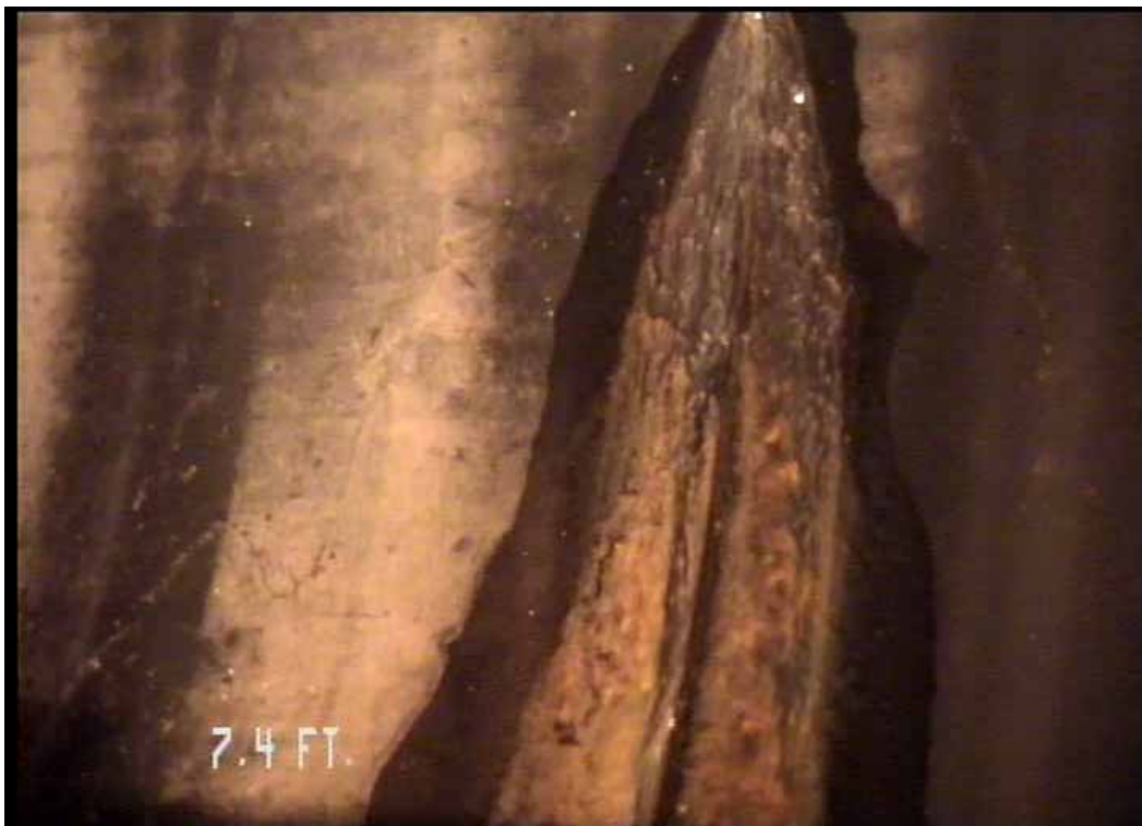
Figure 525 View of cracking/leaking failures for pipeline No. 8 (Site No. 1: Orlando)
