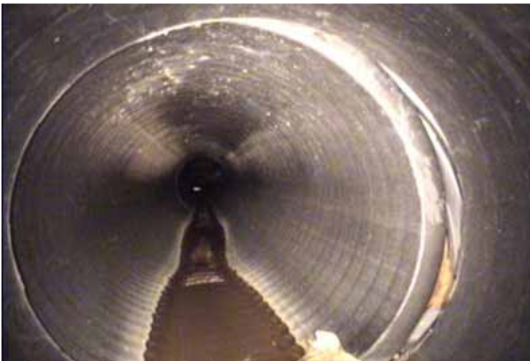
Figure 115 View of cracking/fracture failure for pipeline No. 3 (Site No. 2: Chesterfield – Bandermill)
