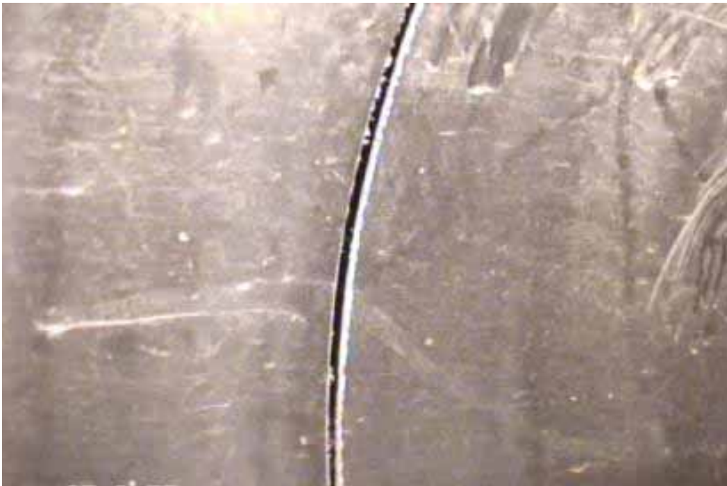
Figure 272 Cracking/fracture failure for Pipeline No. 3 (Site No. 1: Route 101)
