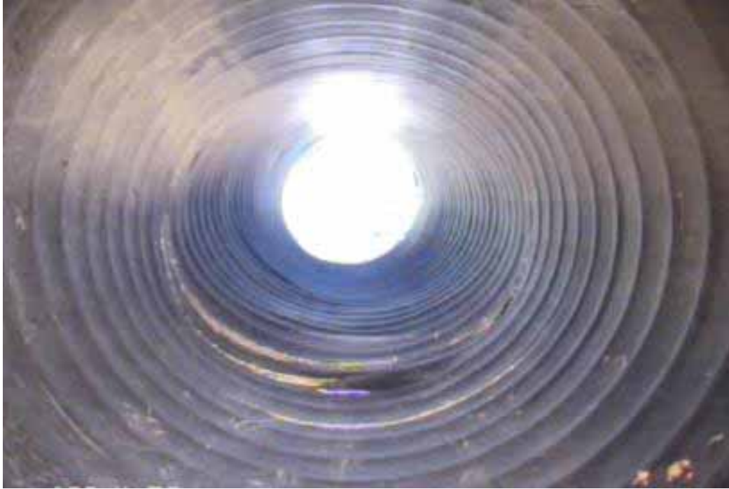
Figure 311 Cracking/fracture and corrugation growth failure for Pipeline No. 10 (Site No. 1: Route 101)
