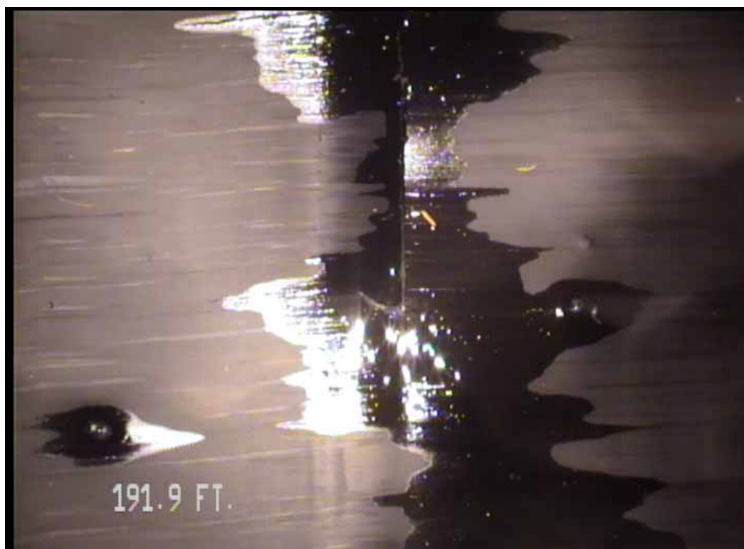
Figure 494 View of the cracking/leaking failures for pipeline No. 3
