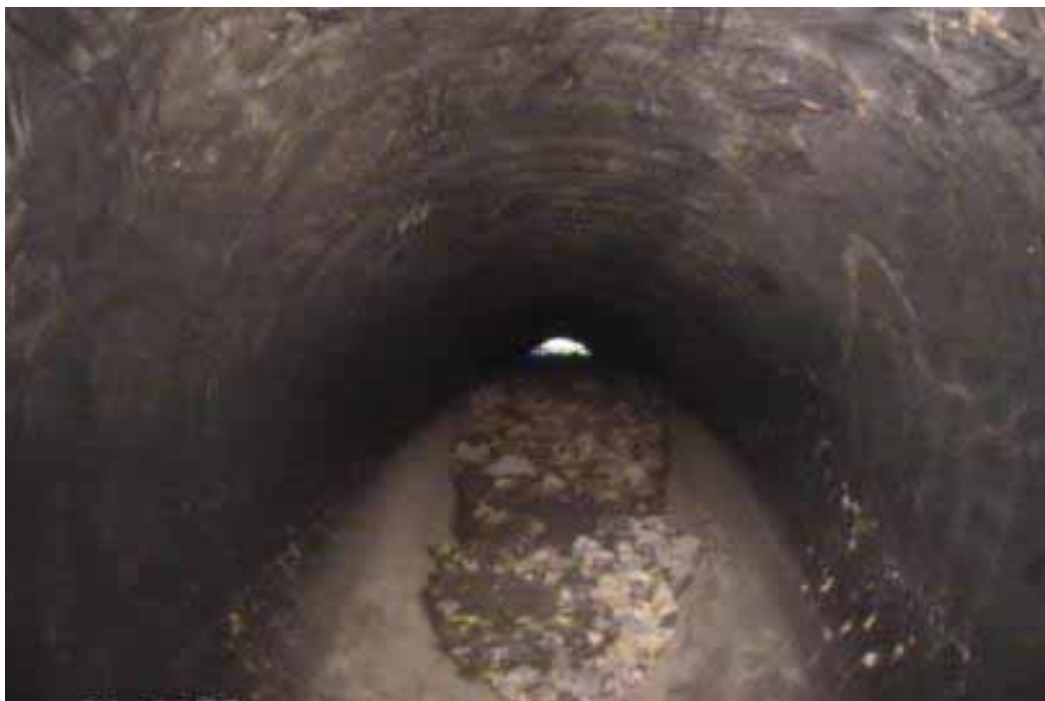
Figure 287 Debris blockage for Pipeline No. 6 (Site No. 1: Route 101)
