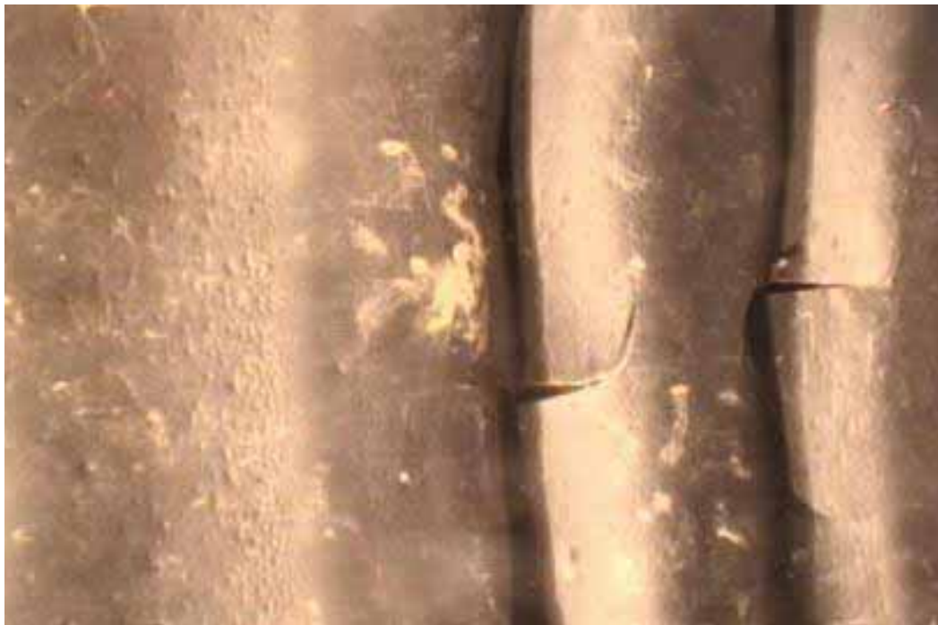
Figure 303 Cracking/fracture failure for Pipeline No. 9 (Site No. 1: Route 101)
