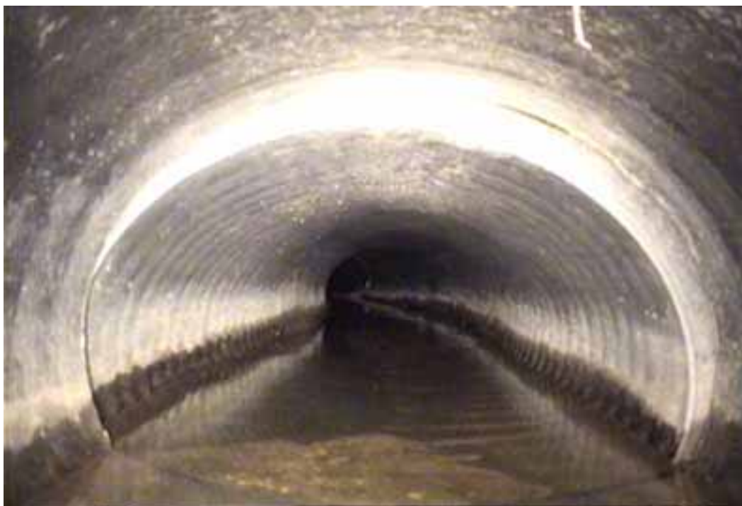
Figure 121 View of joint between two segments of the pipes for pipeline No. 4 (Site No. 3: Spotsylvania County)
