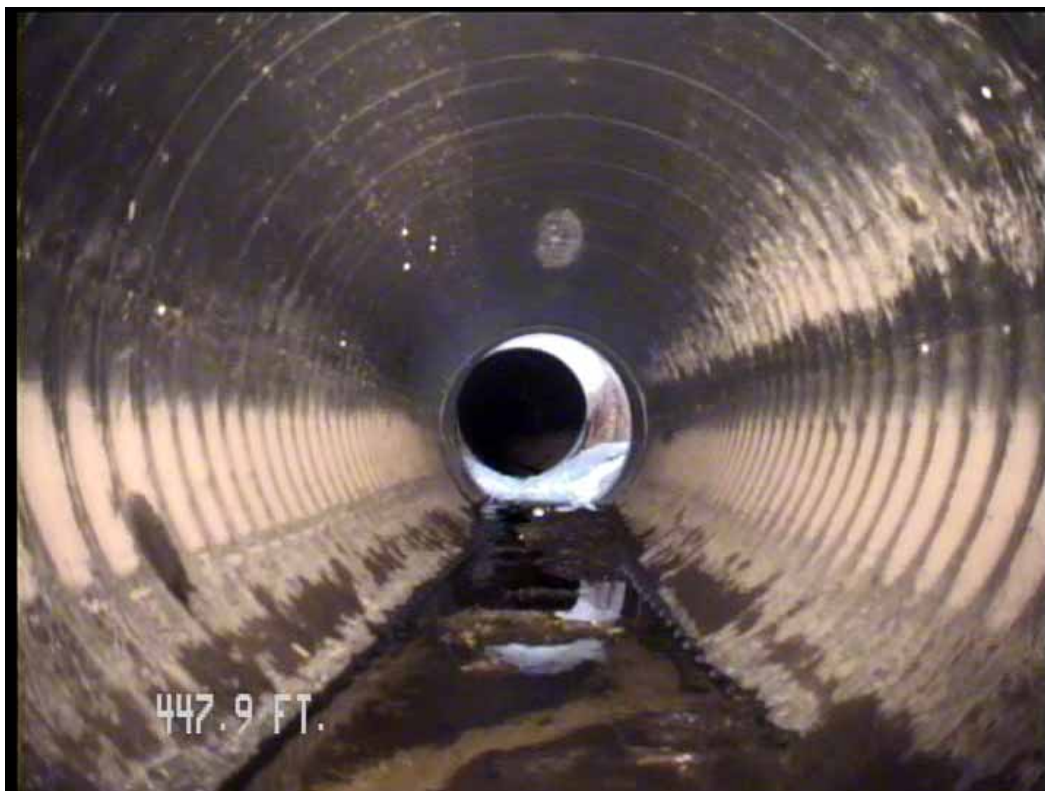
Figure 489 View of the corrugation growth failure for pipeline No. 2 (Site No. 1: Orlando)
