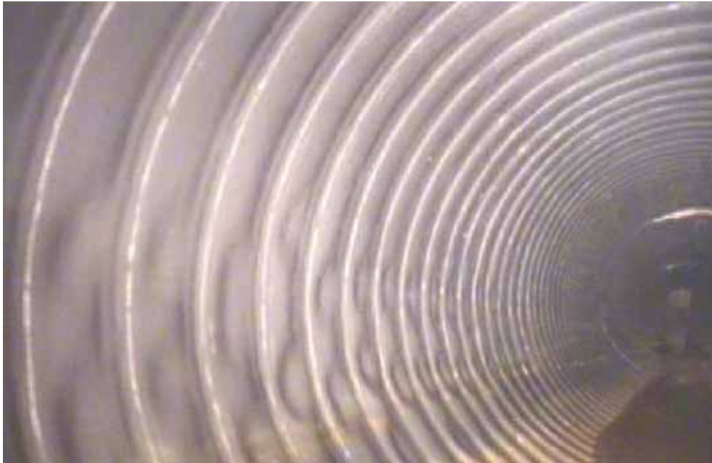
Figure 196 View of corrugation growth and buckling failure for pipeline No. 29 (Site No. 8: Fairmont)
