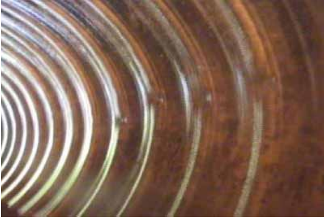
Figure 420 Corrugation growth and buckling failure for Pipeline No. 8 (Site No. 7: West Island Road)
