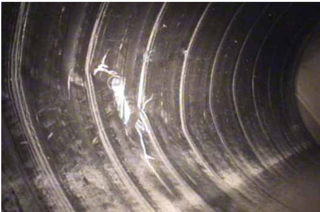
Figure 55 Cracking/fracture and corrugation growth failure for pipeline No. 20 (Segment 2) (Site No. 8: Houston – Fennell)
