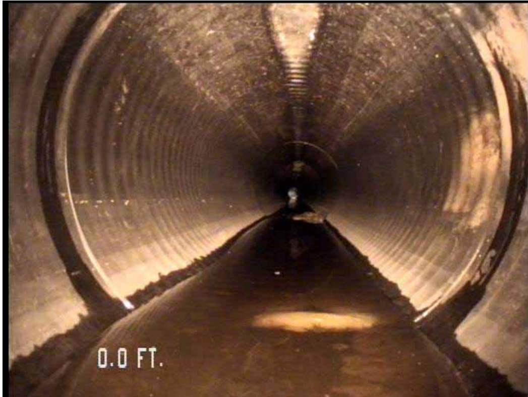
Figure 533 View of the corrugation growth failure at the opening of pipeline No. 9 (Site No. 1: Orlando)
