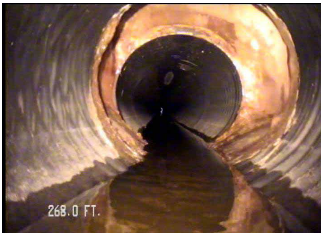
Figure 531 View of the buckling, corrugation growth failures and dip in line and grade for pipeline No. 8 (Site No. 1: Orlando)
