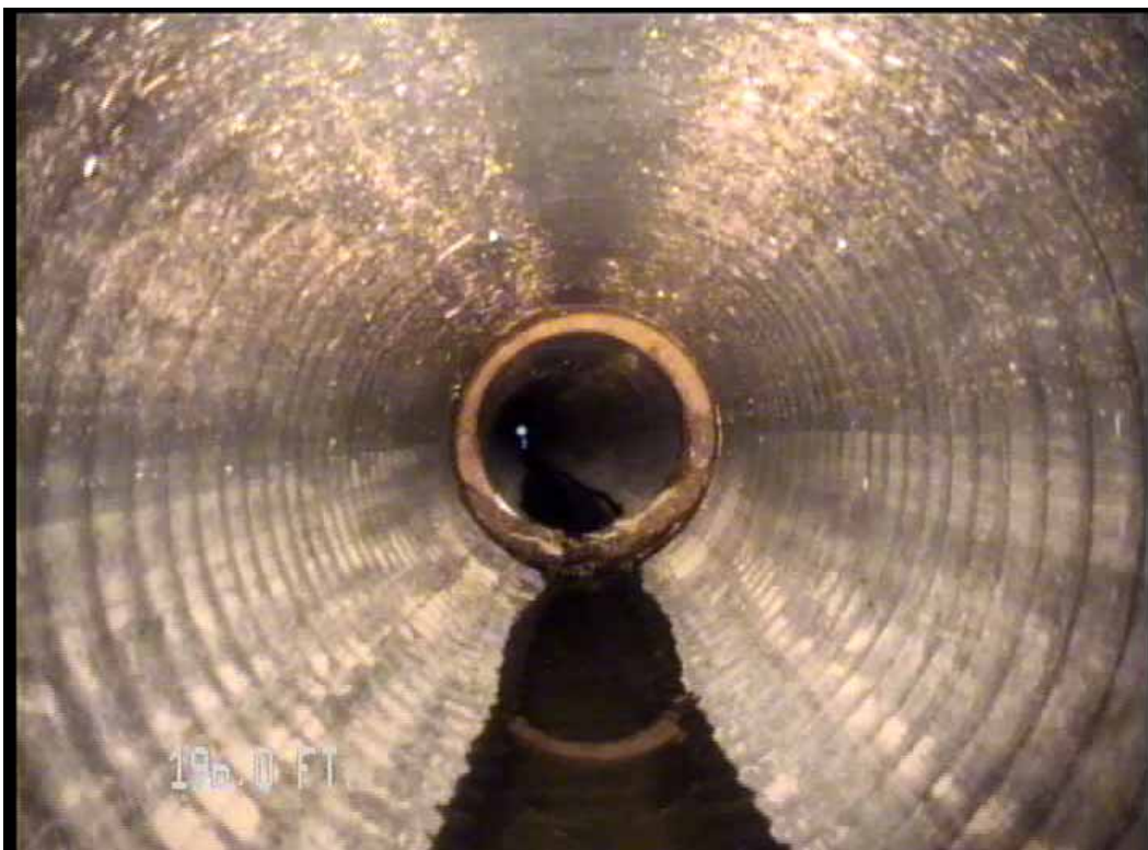
Figure 513 View of the corrugation growth failure for pipeline No. 6 (Site No. 1: Orlando)
