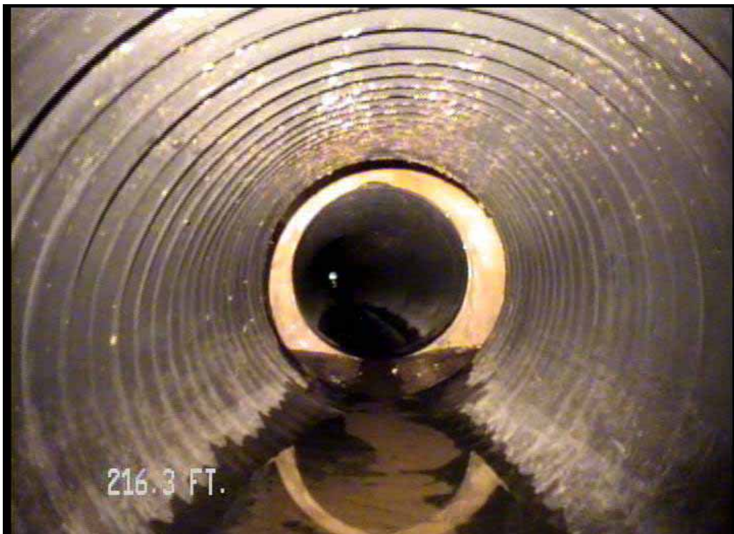
Figure 479 View of excessive deformation and corrugation growth failures for pipeline No. 1 (Site No. 1: Orlando)
