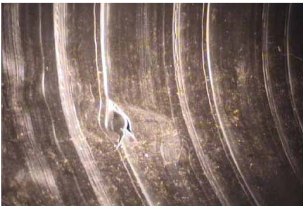
Figure 93 View of buckling and cracking failures for pipeline No. 11 (Site No. 6: Rockingham – Love Ln)
