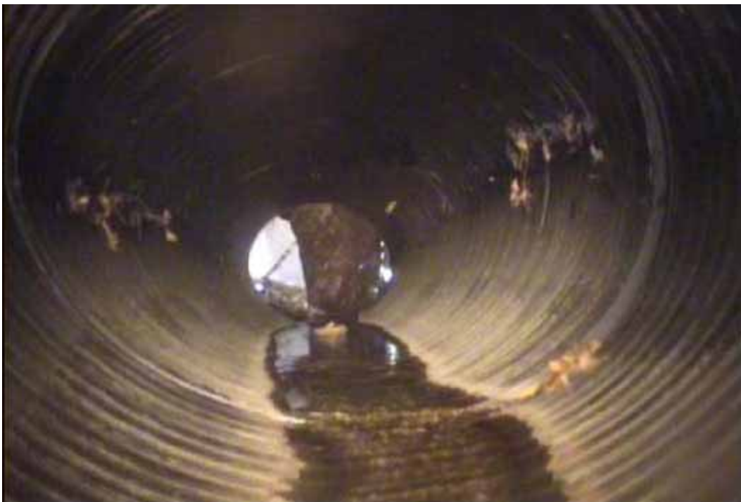
Figure 85 View of excessive deformation failure for pipeline No. 10 (Site No. 6: Rockingham – Love Ln)
