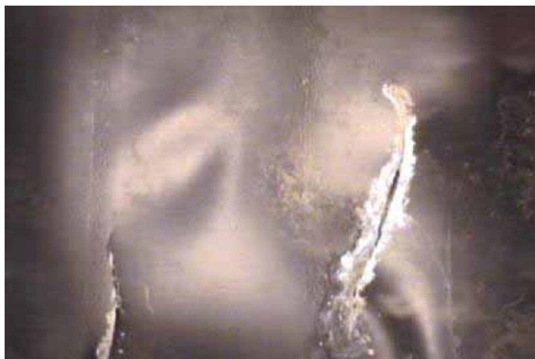
Figure 387 Cracking/fracture and buckling failure for Pipeline No. 10 (Site No. 2: Silver Creek Parkway)
