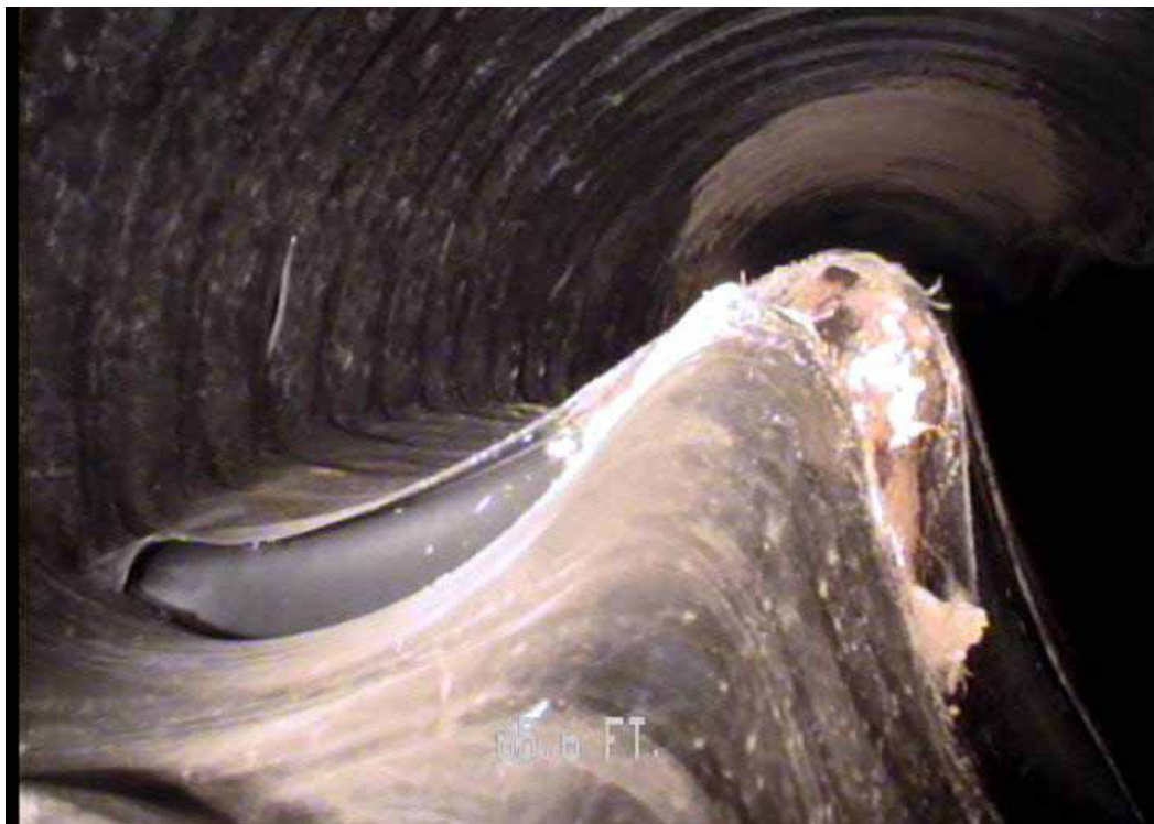
Figure 549 Close view of the inverse curvature/crack/fracture failures for pipeline No. 10 (Site No. 2: Apopka)
