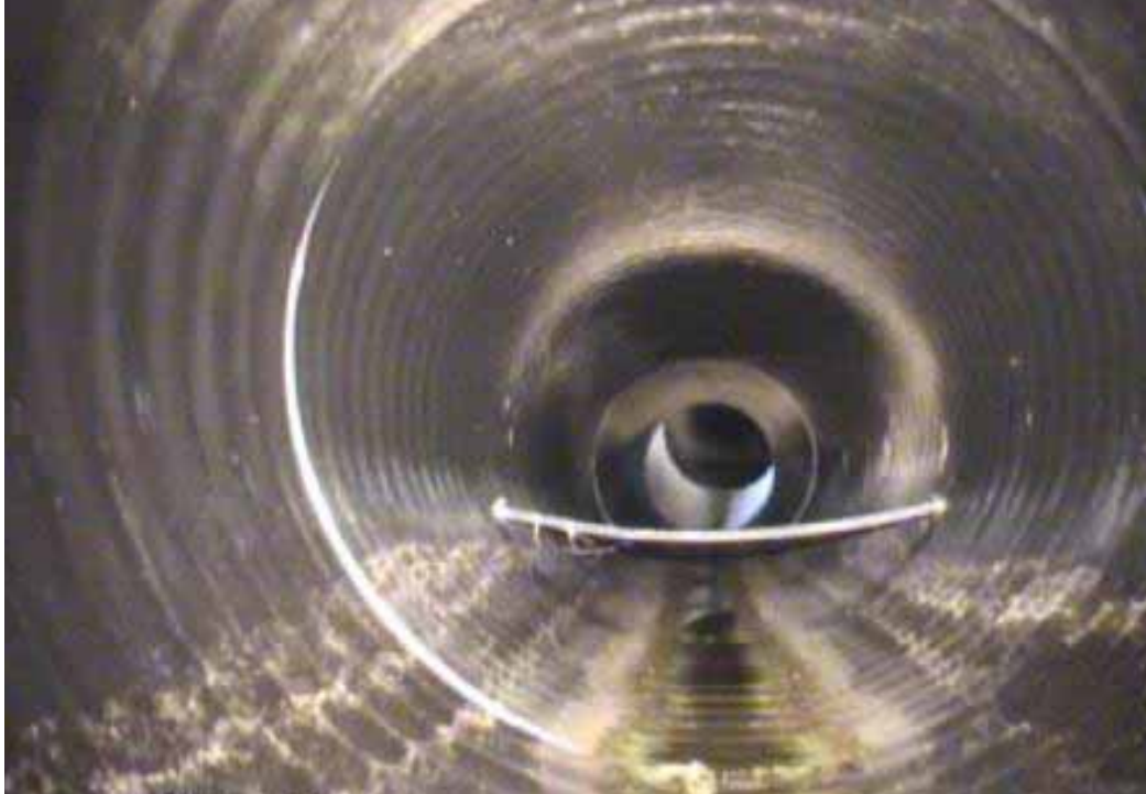
Figure 218 View of corrugation failure and pipe intrusion for pipeline No. 6 (Site No. 1: Lenexa)
