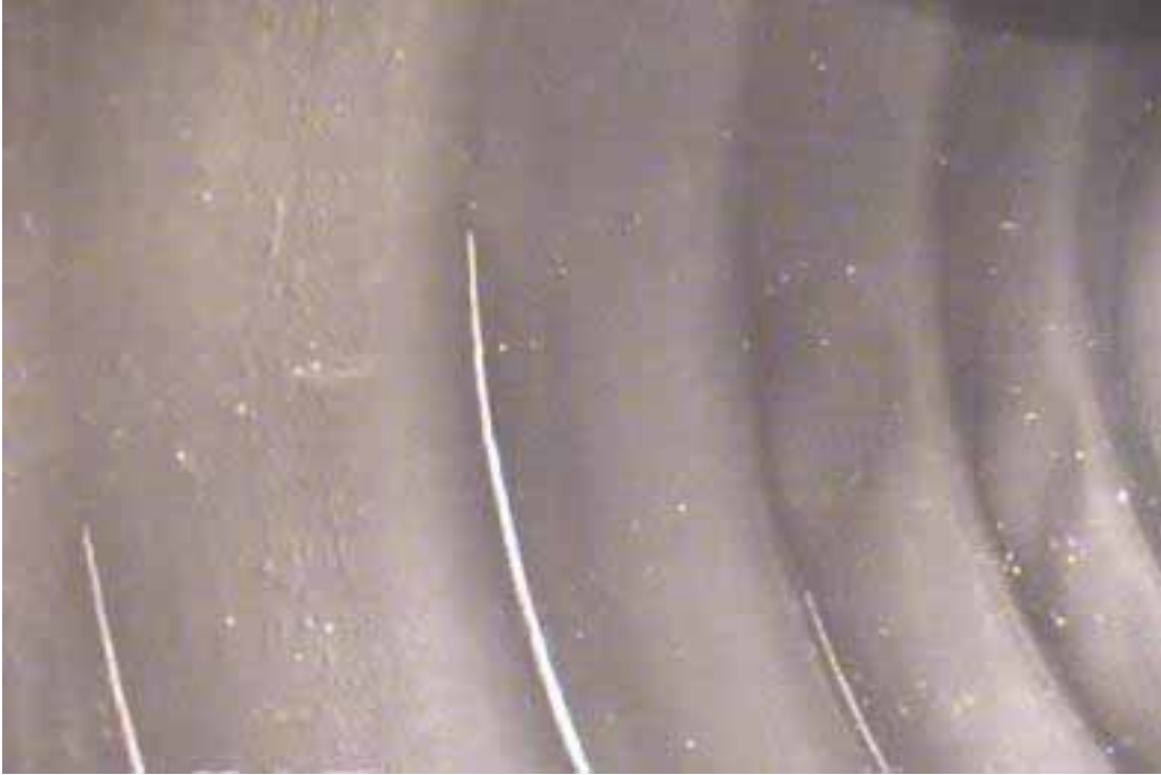
Figure 336 Cracking/fracture and corrugation growth failure for Pipeline No. 22 (Site No. 2: Route 36)
