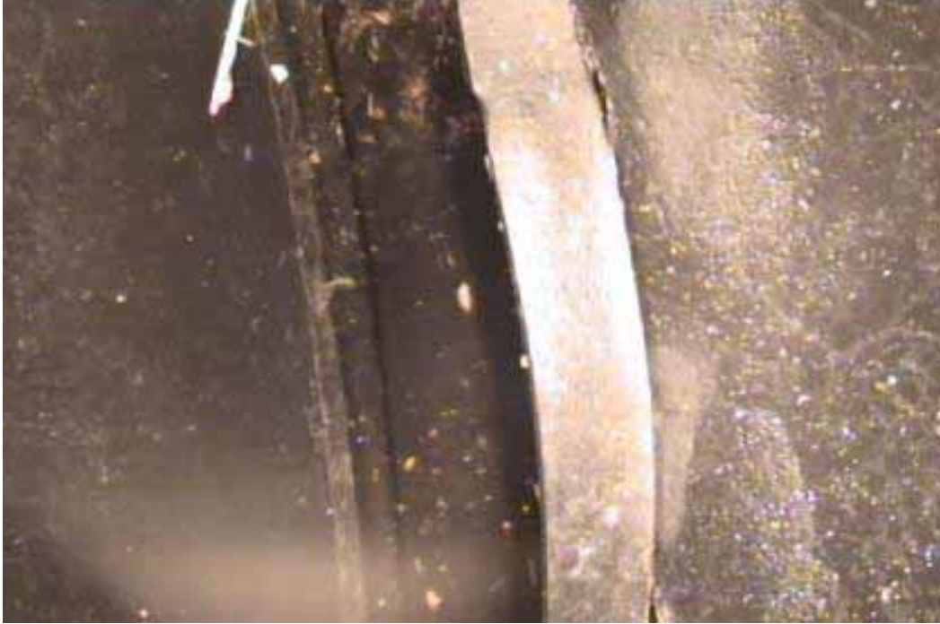
Figure 426 Cracking/fracture failure for Pipeline No. 9 (Site No. 8: Kinross Road)
