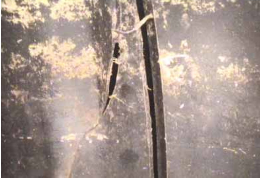
Figure 169 View of cracking/fracture failure for pipeline No. 9 (Site No. 3: Blaine - Xylite)
