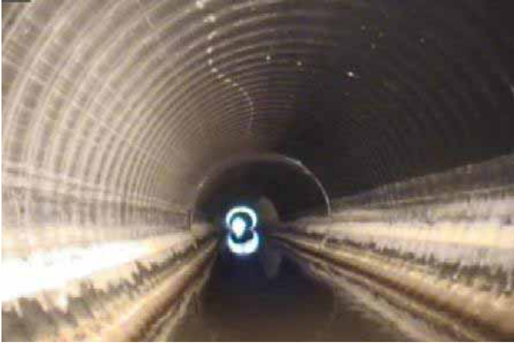
Figure 375 Excessive deformation failure (refer to Figure 374-d) for Pipeline No. 8 (Site No. 1: Legacy Parkway)
