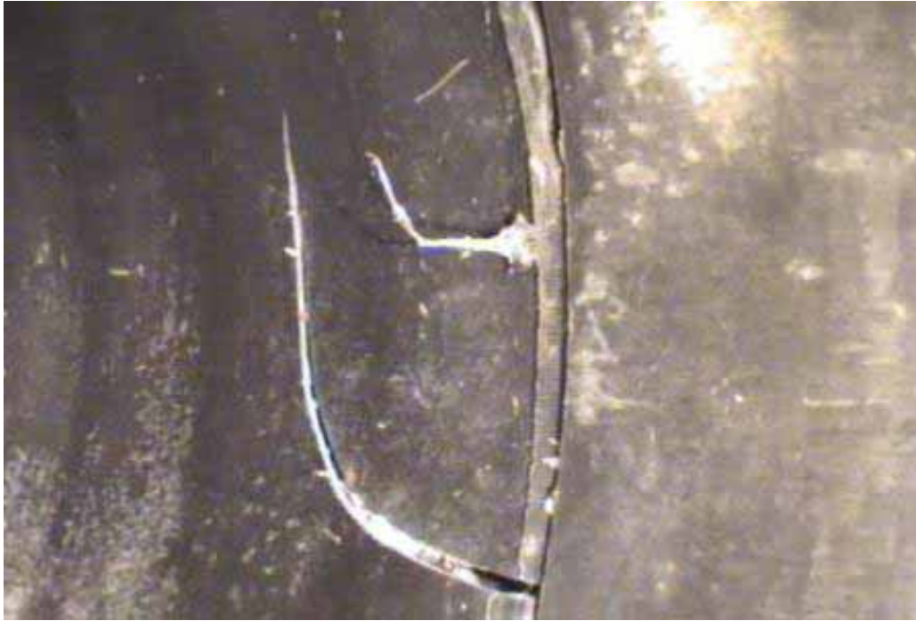
Figure 401 Cracking/fracture and major joint failure for Pipeline No. 5 (Site No. 5: Bad Axe)
