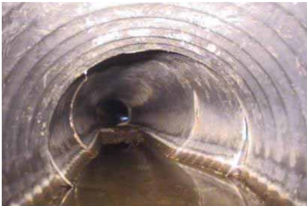
Figure 265 Corrugation growth and excessive deformation failures for Pipeline No. 2 (Site No. 1: Route 101)
