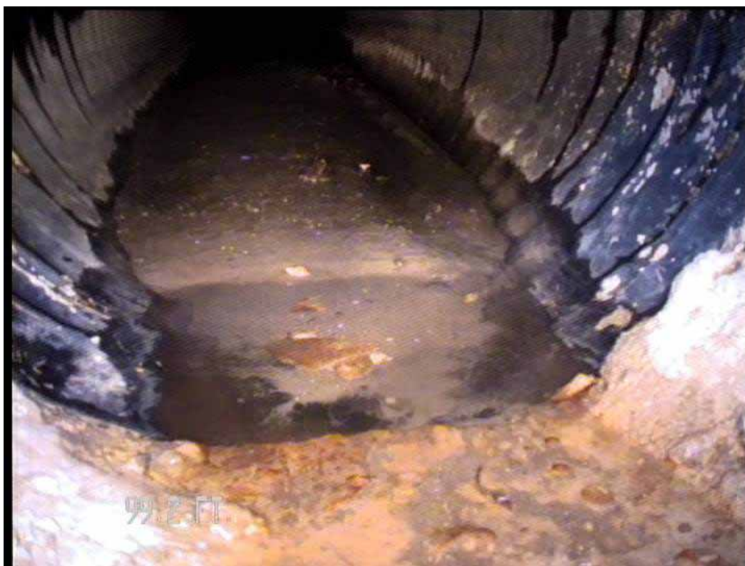
Figure 580 View of the corrugation growth failure at the opening for pipeline No. 15 (Site No. 2: Apopka)
