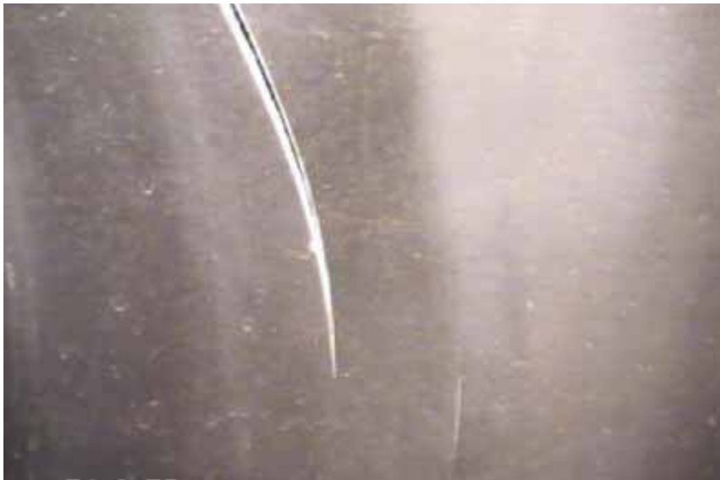
Figure 273 Cracking/fracture failure for Pipeline No. 3 (Site No. 1: Route 101)
