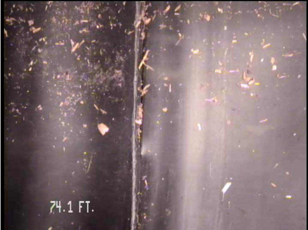
Figure 506 View of the minor joint displacement failure for pipeline No. 6 (Site No. 1: Orlando)
