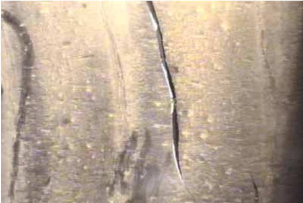
Figure 307 Cracking/fracture failure for Pipeline No. 10 (Site No. 1: Route 101)
