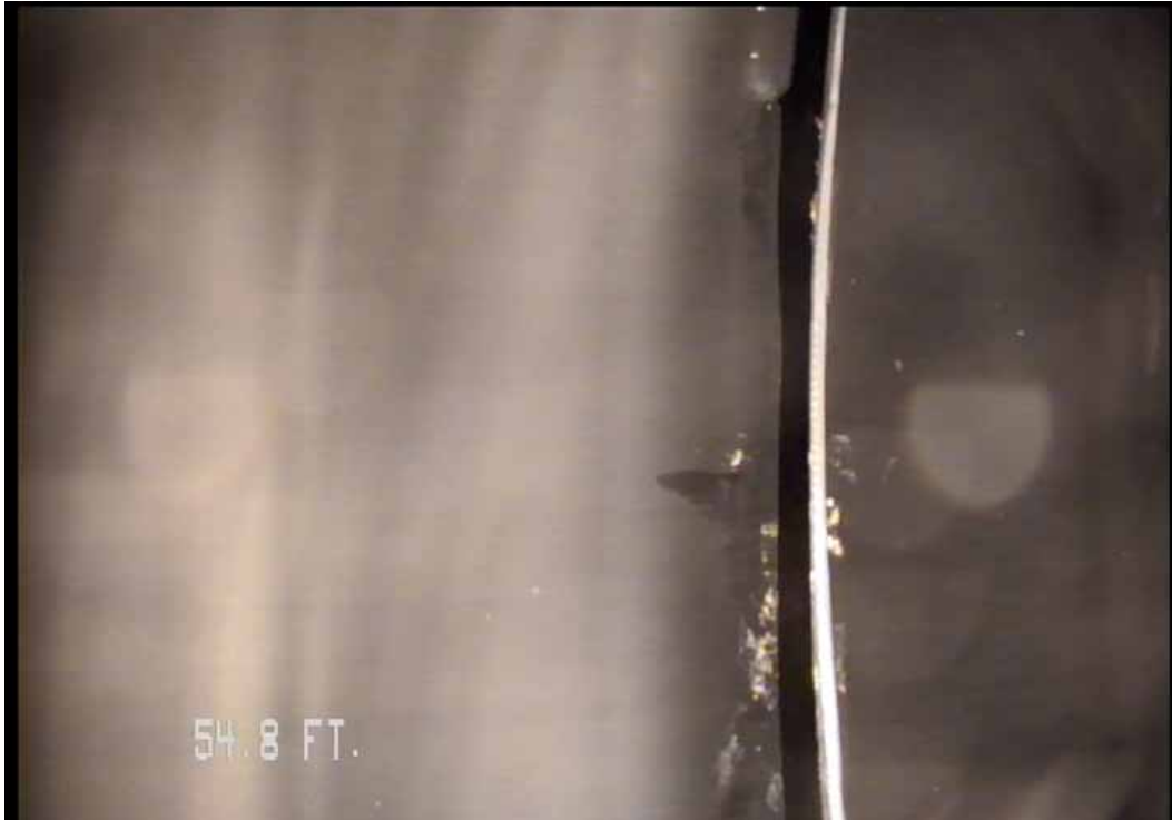
Figure 478 View of the major joint displacement failure for pipeline No. 1 (Site No. 1: Orlando)
