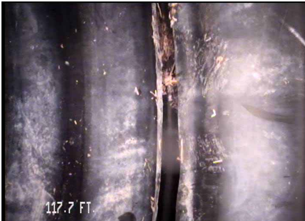
Figure 582 View of major joint displacement failure of pipeline No. 15 (Site No. 2: Apopka)
