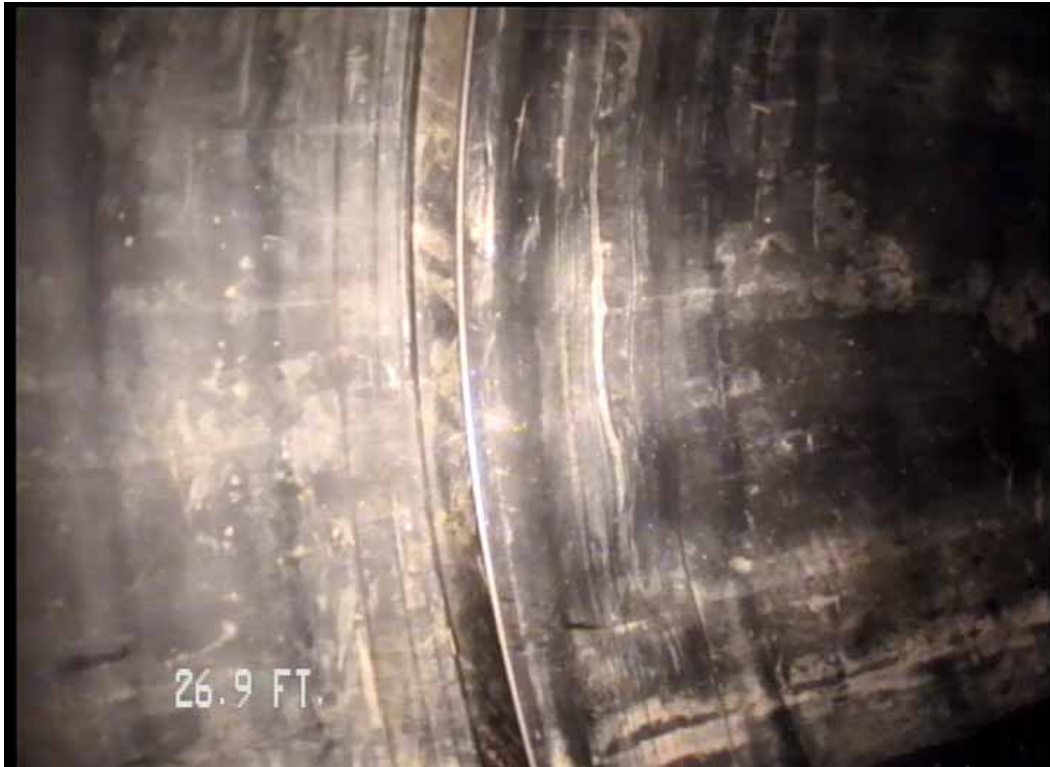
Figure 526 View of major joint displacement and buckling failures for pipeline No. 8 (Site No. 1: Orlando)
