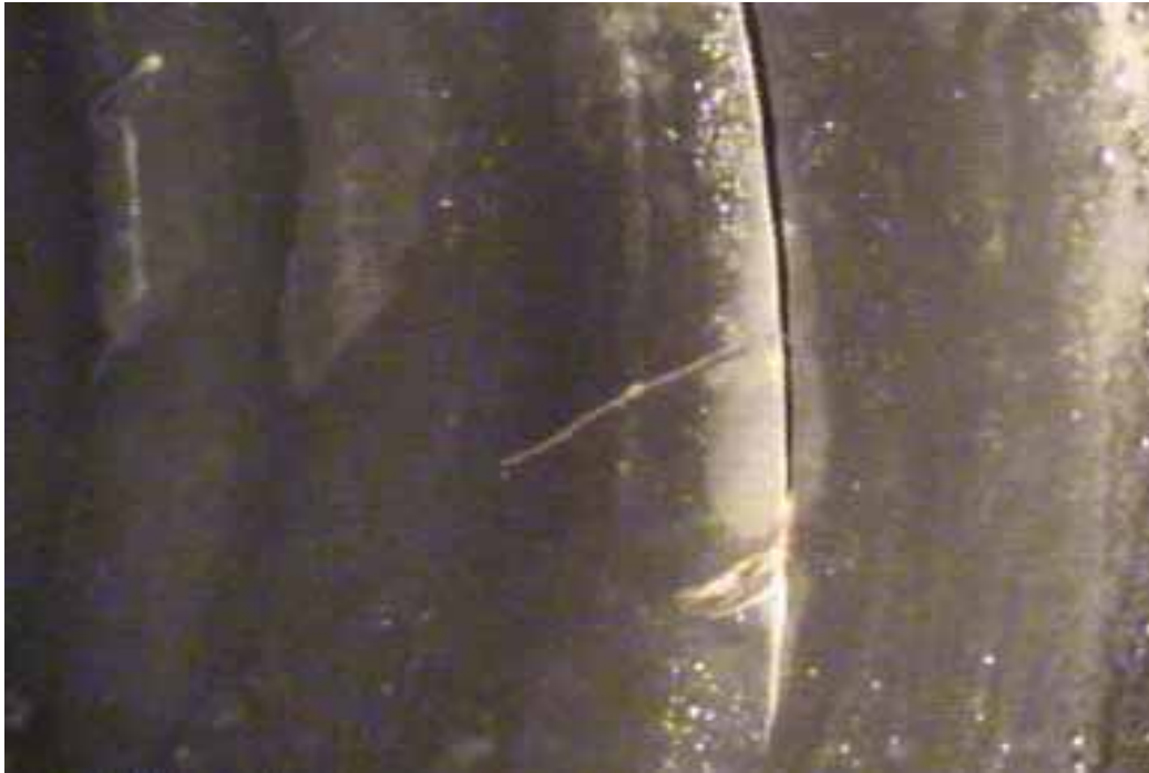
Figure 403 Cracking/fracture and major joint failure for Pipeline No. 5 (Site No. 5: Bad Axe)
