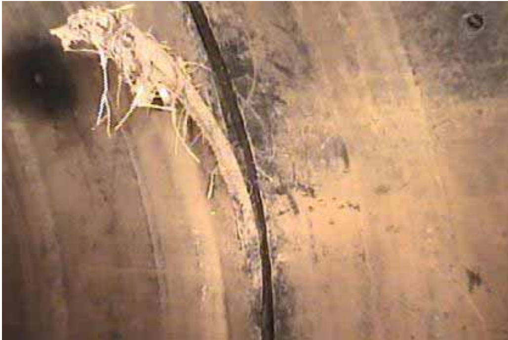
Figure 415 Cracking/fracture and major joint displacement failure for Pipeline No. 7 (Site No. 7: West Island Road)
