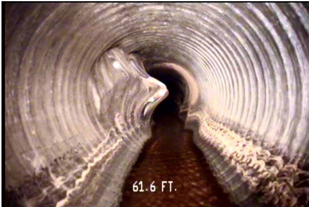
Figure 548 View of the inverse curvature failure for pipeline No. 10 (Site No. 2: Apopka)
