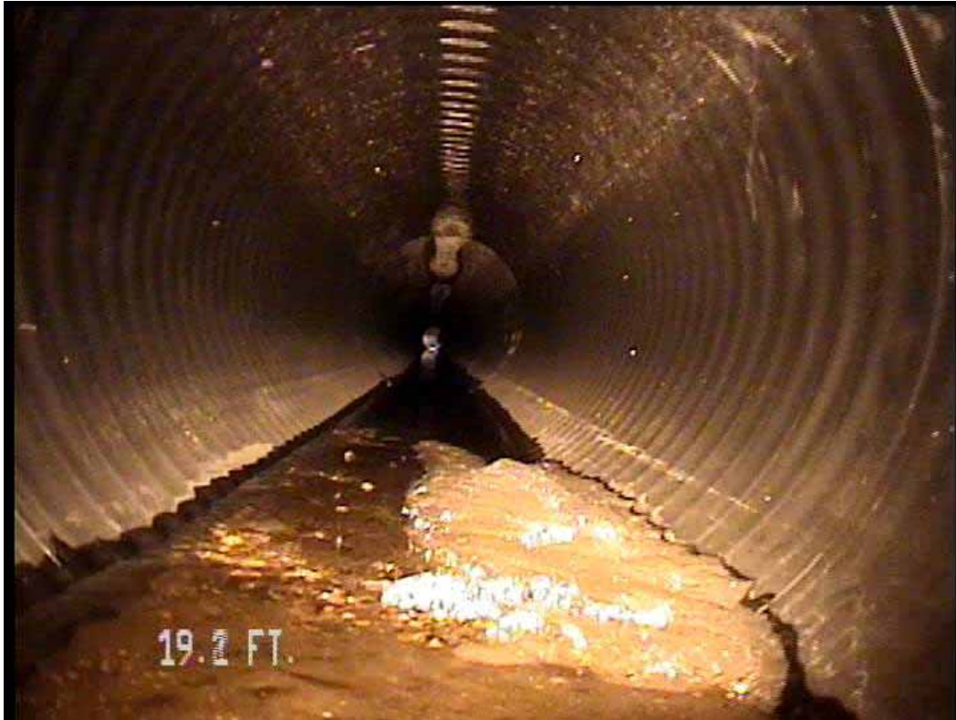
Figure 535 View of the corrugation growth for pipeline No. 9 (Site No. 1: Orlando)
