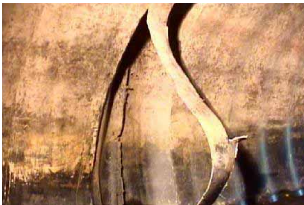
Figure 457 Cracking/fracture, major joint displacement, and corrugation growth failure for Pipeline No. 23 (Site No. 12: 48 th Avenue)
