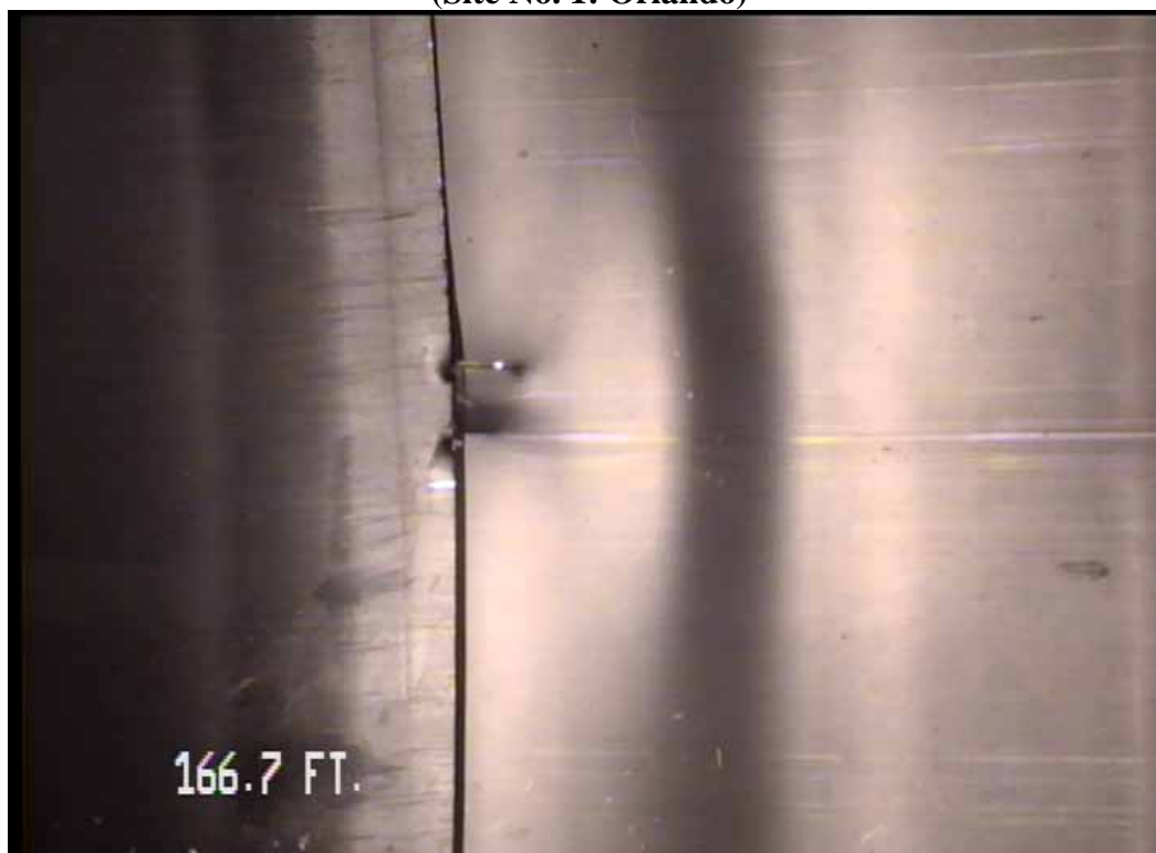
Figure 493 View of the cracking and buckling failures for pipeline No. 3 (Site No. 1: Orlando)
