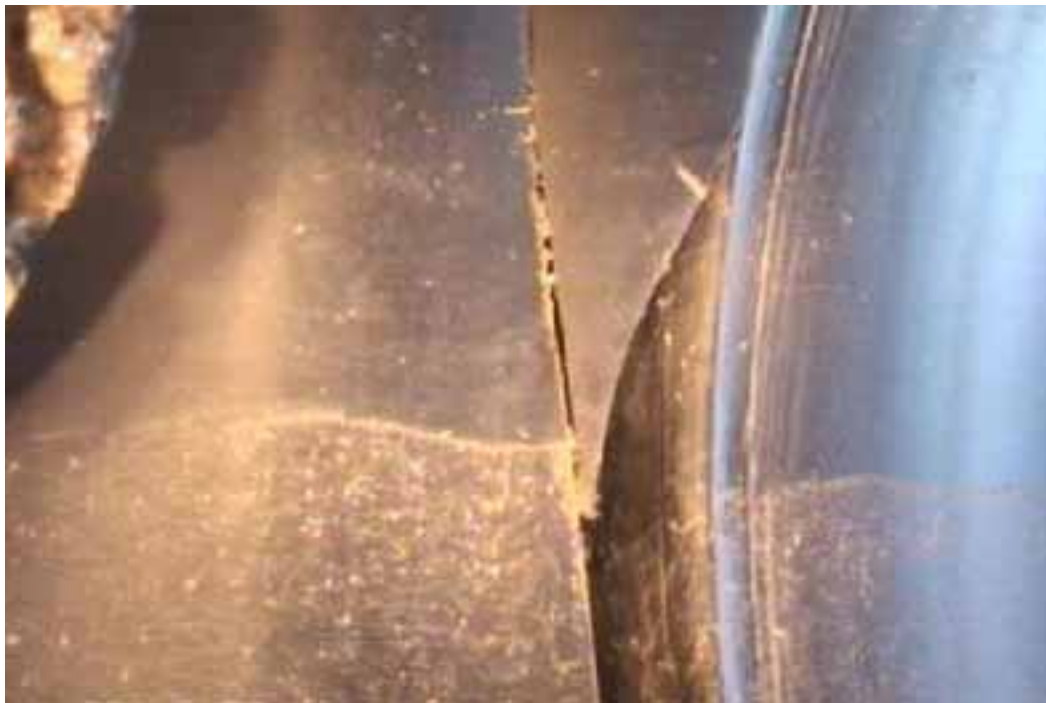
Figure 388 Cracking/fracture and joint displacement failure for Pipeline No. 10 (Site No. 2: Silver Creek Parkway)
