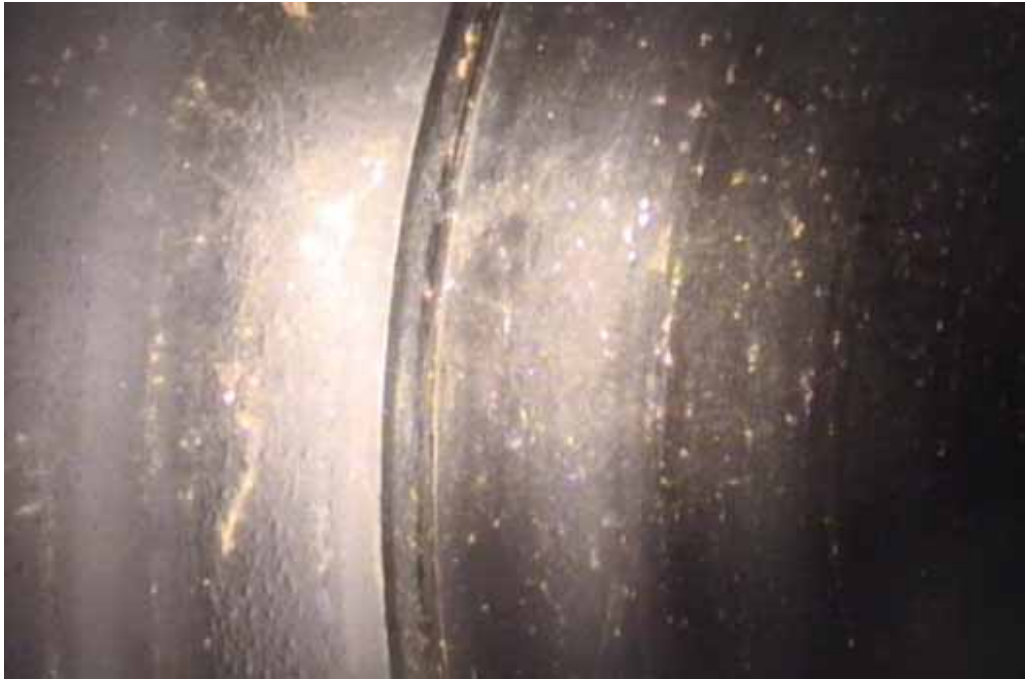
Figure 78 View of joint displacement failure for pipeline No. 9 (Site No. 5: Hickory – Oxford School Rd)
