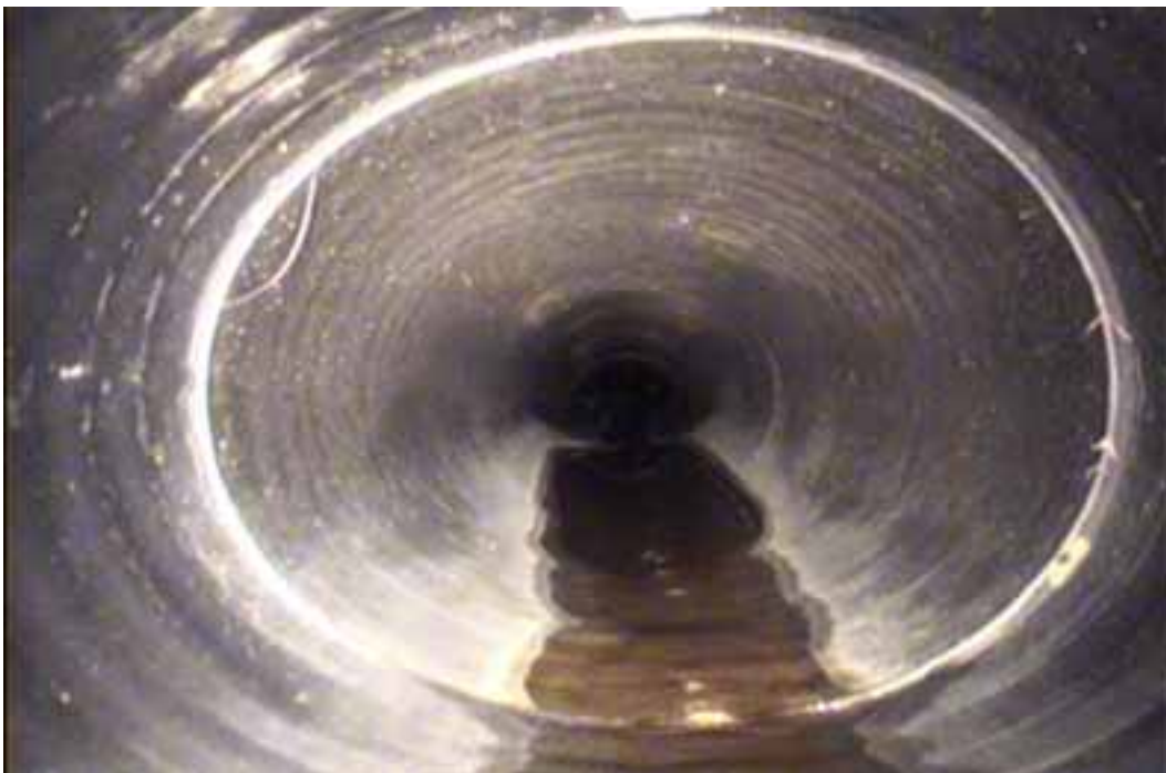
Figure 119 View of excessive deformation failure for pipeline No. 4 (Site No. 3: Spotsylvania County)
