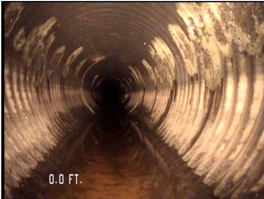
Figure 482 View of the corrugation growth failure for pipeline No. 2 (Site No. 1: Orlando)
