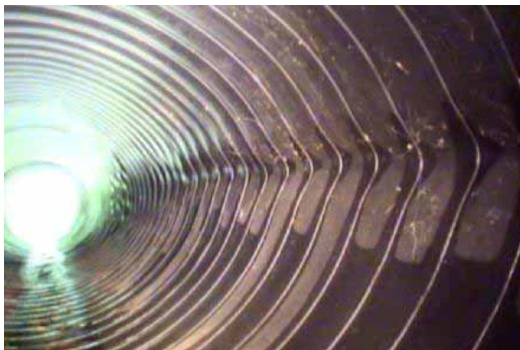
Figure 448 Buckling and corrugation growth failure for Pipeline No. 21 (Site No. 11: Houghton County-North Laird Heights)
