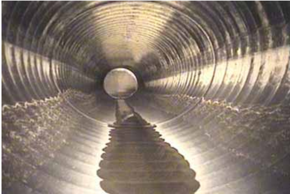
Figure 130 View of excessive deformation and corrugation growth failures for pipeline No. 7 (Site No. 4: Mechanicsville)
