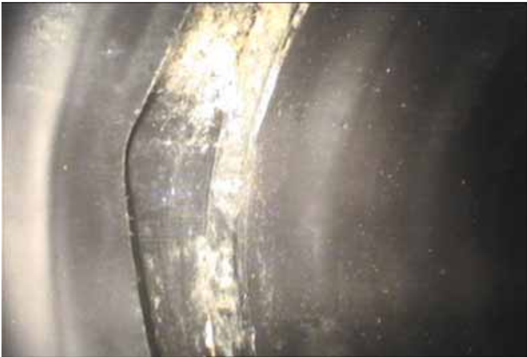
Figure 133 View of deformation of the pipe for pipeline No. 8 (Site No. 4: Mechanicsville)
