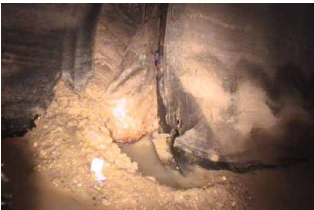
Figure 44 Major joint displacement failure for pipeline No. 19 (Segment 1) (Site No. 8: Houston – Fennell)
