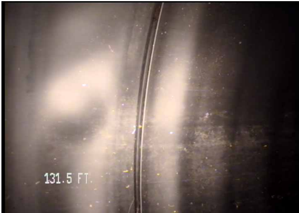
Figure 519 View of the minor joint displacement and buckling failures for pipeline No. 7 (Site No. 1: Orlando)
