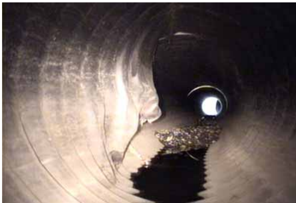
Figure 143 View of cracking/fracture failure for pipeline No. 15 (Site No. 6: Winchester)
