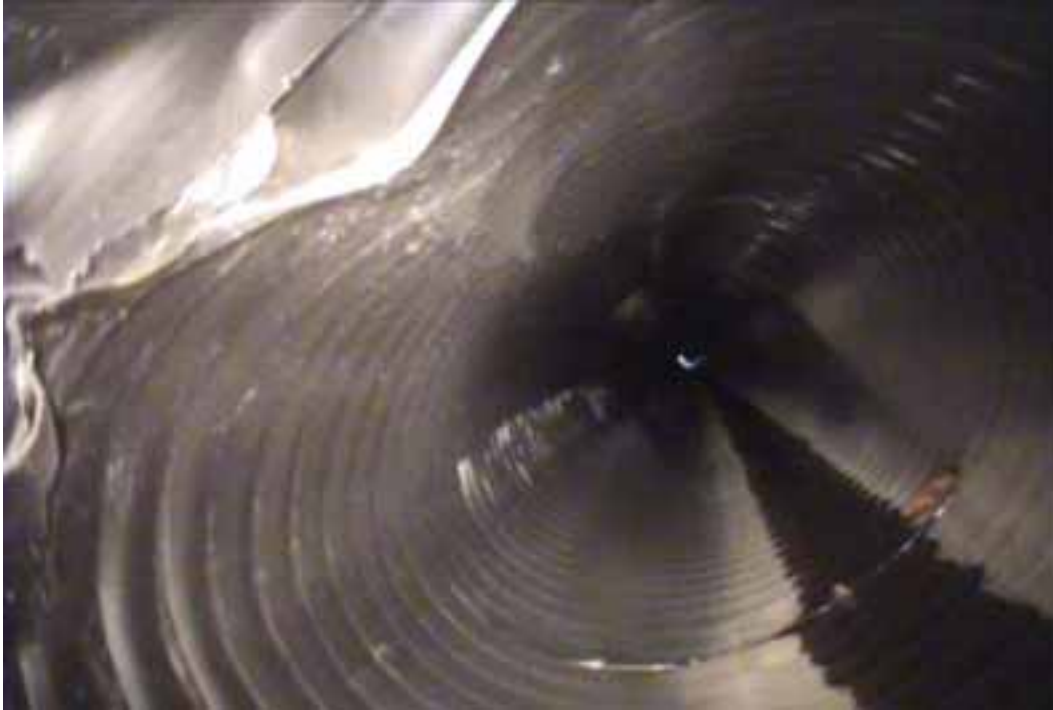
Figure 129 View of cracking/fracture failure for pipeline No. 6 (Site No. 4: Mechanicsville)
