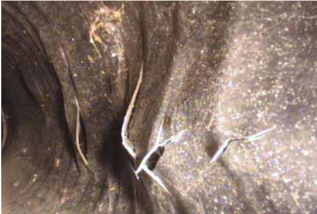
Figure 299 Cracking/fracture, inverse curvature, and corrugation growth failure for Pipeline No. 8 (Site No. 1: Route 101)
