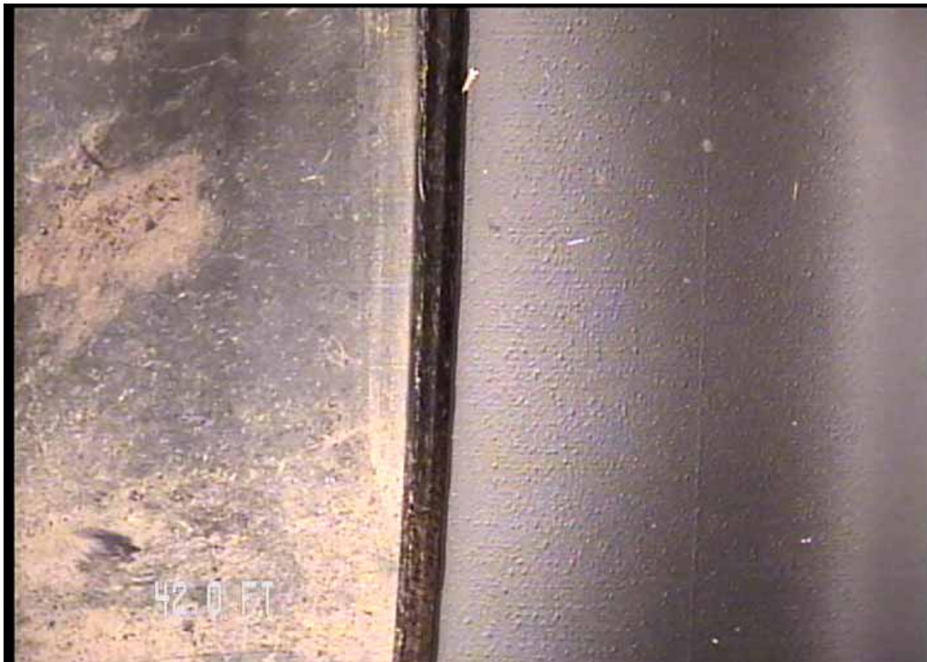
Figure 537 View of the major joint displacement failure for pipeline No. 9 (Site No. 1: Orlando)
