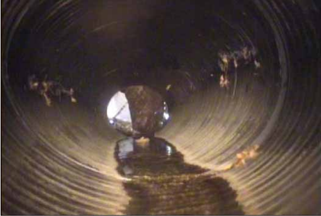
Figure 90 View of excessive deformation failure for pipeline No. 11 (Site No. 6: Rockingham – Love Ln)
