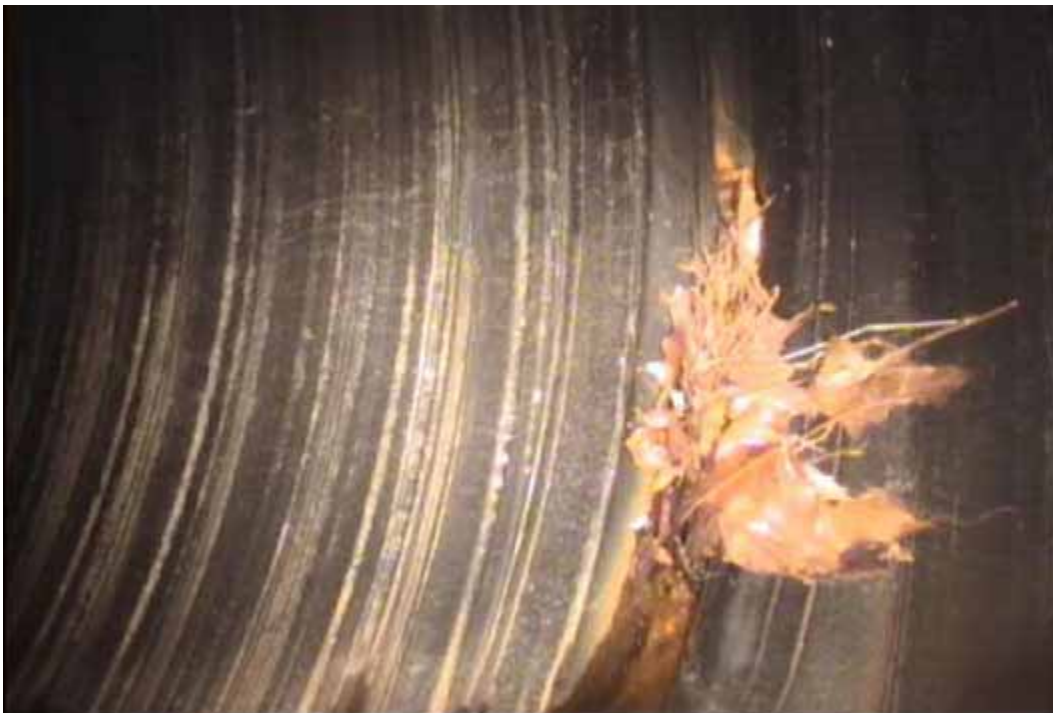
Figure 83 View of major joint displacement failure for pipeline No. 10 (Site No. 6: Rockingham – Love Ln)
