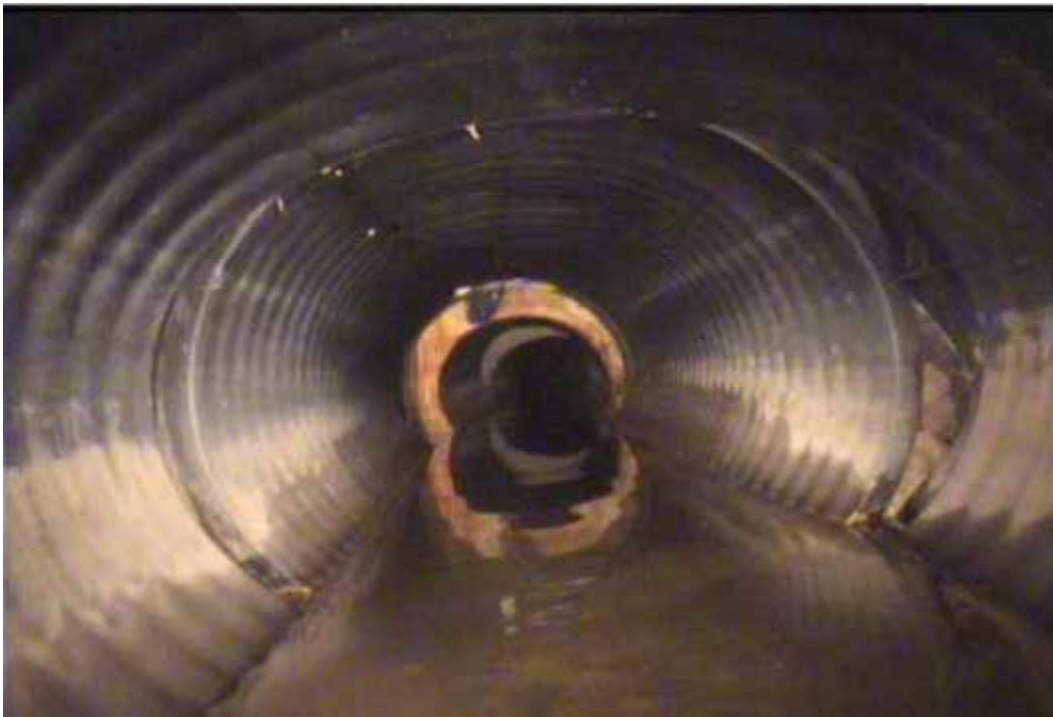
Figure 48 Major joint displacement and excessive deformation failures for pipeline No. 19 (Segment 2) (Site No. 8: Houston – Fennell)
