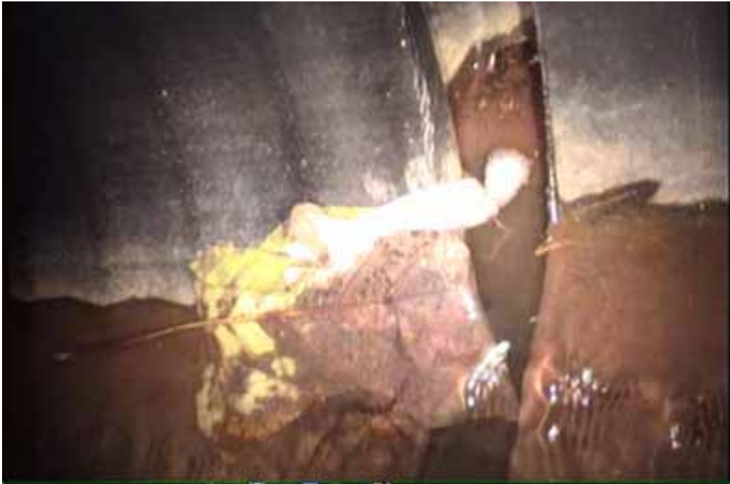
Figure 114 View of major joint displacement failure for pipeline No. 3 (Site No. 2: Chesterfield – Bandermill)
