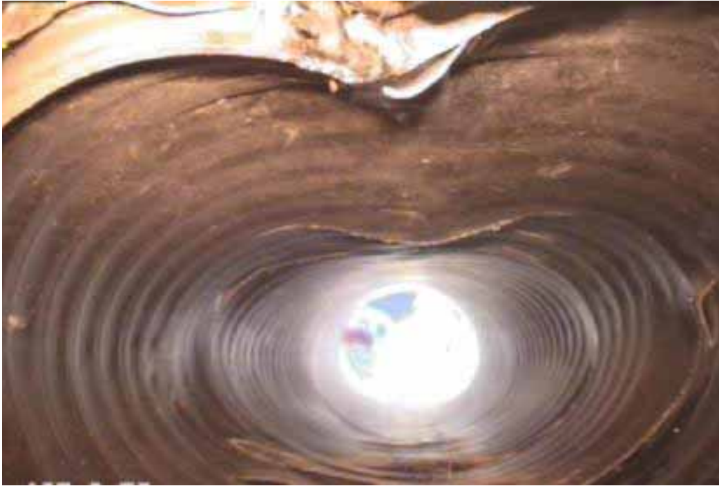
Figure 269 Inverse curvature, cracking/fracture, excessive deformation, and corrugation growth failures for Pipeline No. 2 (Site No. 1: Route 101)
