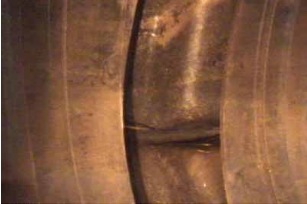
Figure 424 Joint displacement failure for Pipeline No. 8 (Site No. 7: West Island Road)
