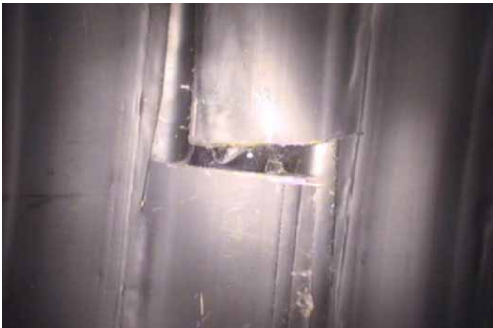
Figure 191 View of cracking/fracture failure for pipeline No. 27 (Site No. 8: Fairmont)
