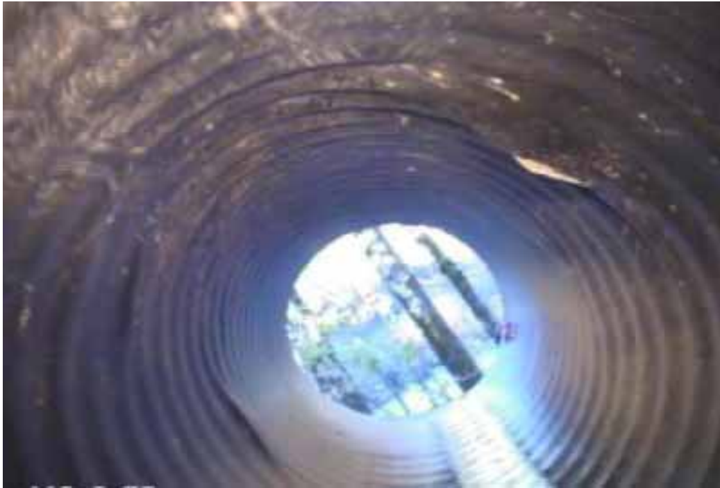
Figure 304 Cracking/fracture, inverse curvature, and corrugation growth failure for Pipeline No. 9 (Site No. 1: Route 101)
