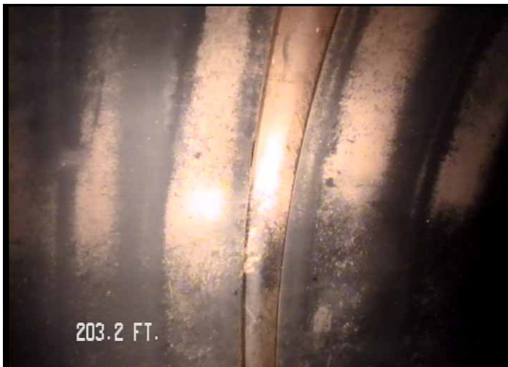
Figure 530 View of major joint displacement for pipeline No. 8 (Site No. 1: Orlando)
