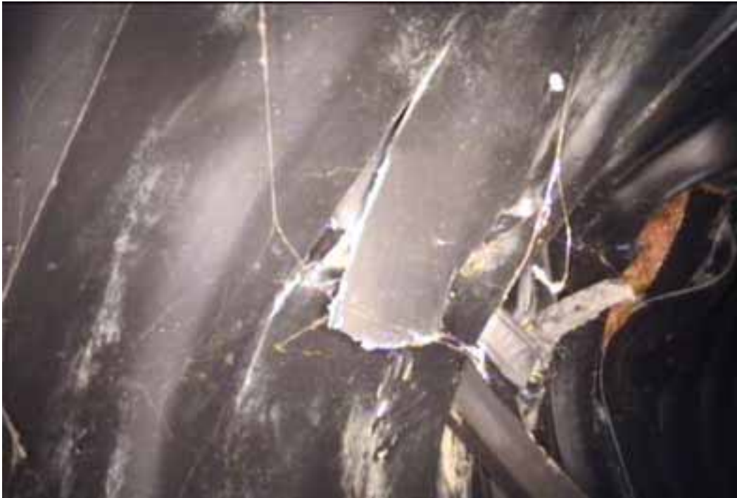
Figure 127 View of cracking/fracture failure for pipeline No. 6 (Site No. 4: Mechanicsville)
