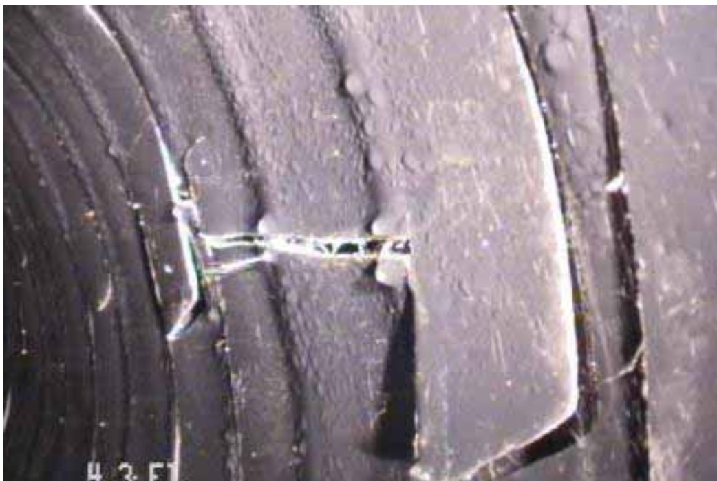
Figure 341 Cracking/fracture and corrugation growth failure for Pipeline No. 23 (Site No. 2: Route 36)
