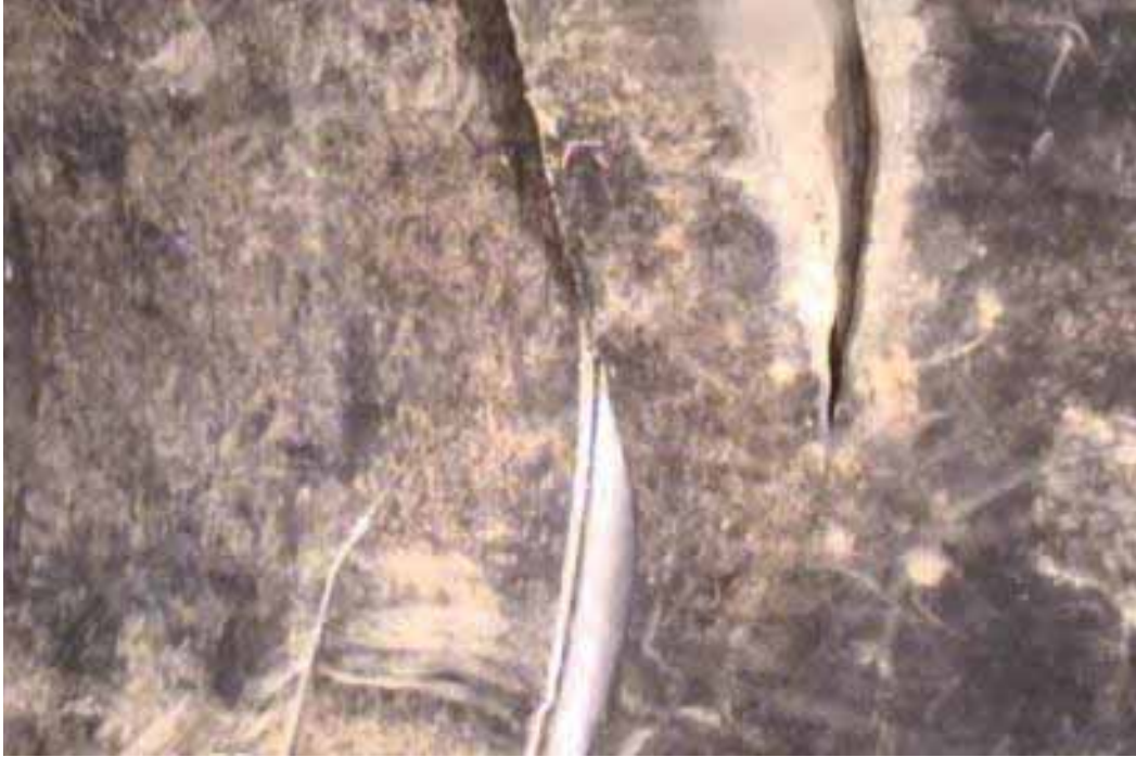
Figure 322 Cracking/fracture failure for Pipeline No. 16 (Site No. 2: Route 36)
