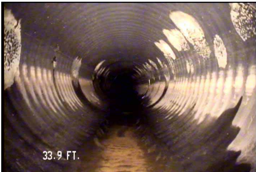
Figure 485 View of the corrugation growth failure for pipeline No. 2 (Site No. 1: Orlando)
