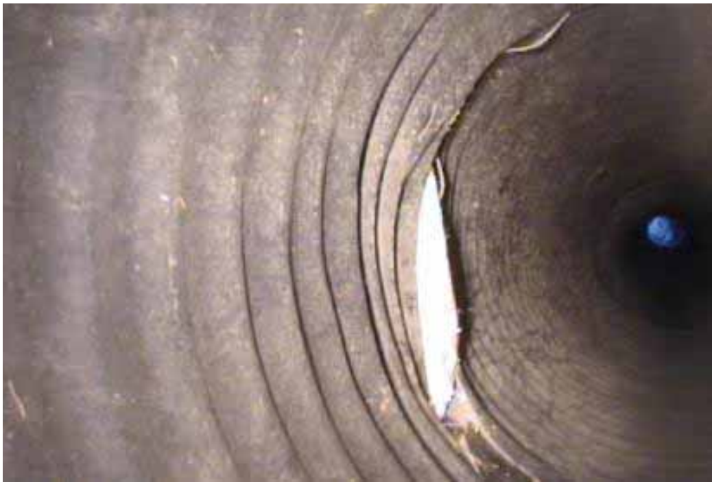
Figure 289 Cracking/fracture and corrugation growth failures for Pipeline No. 7 (Site No. 1: Route 101)
