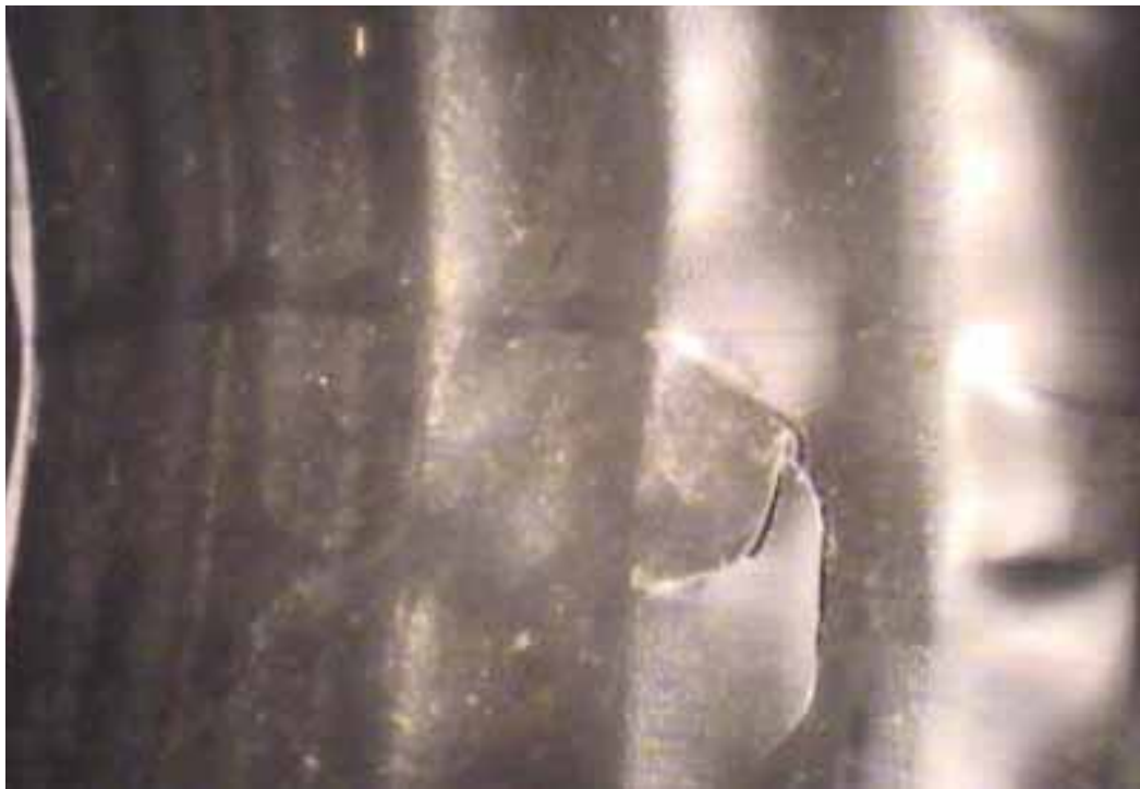
Figure 208 View of the cracking failure for pipeline No. 2 (Site No. 1: Lenexa)
