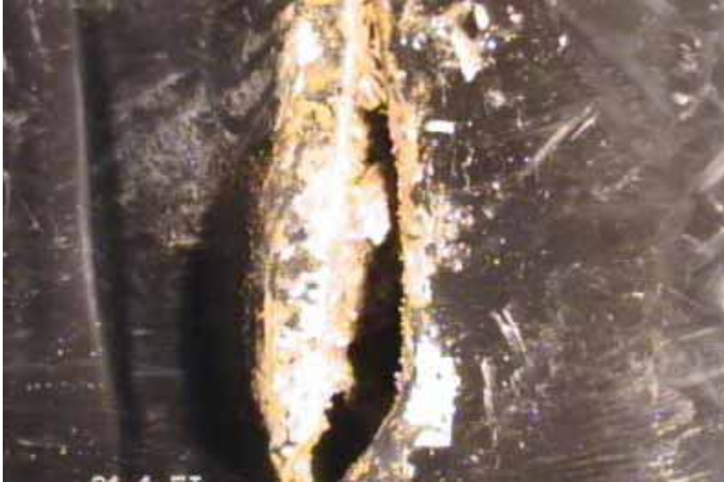
Figure 317 Cracking/fracture failure for Pipeline No. 12 (Site No. 1: Route 101)
