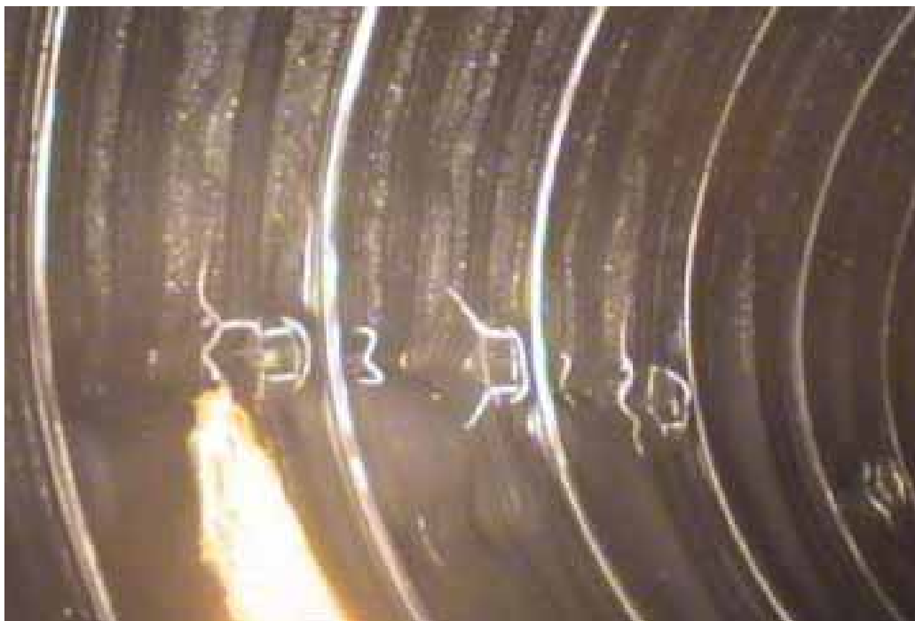
Figure 396 Cracking/fracture, corrugation growth, and buckling failure for Pipeline No. 4 (Site No. 4: Horton)
