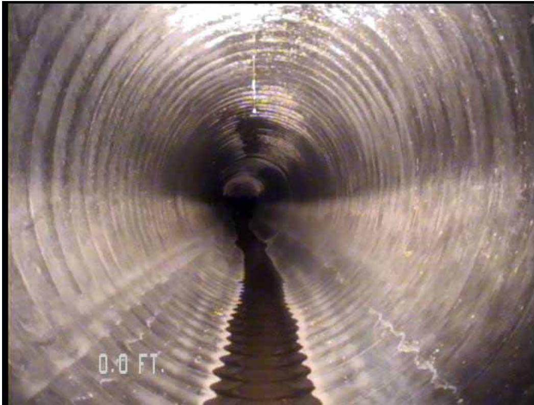
Figure 566 View of the corrugation growth failure at the opening for pipeline No. 13 (Site No. 2: Apopka)
