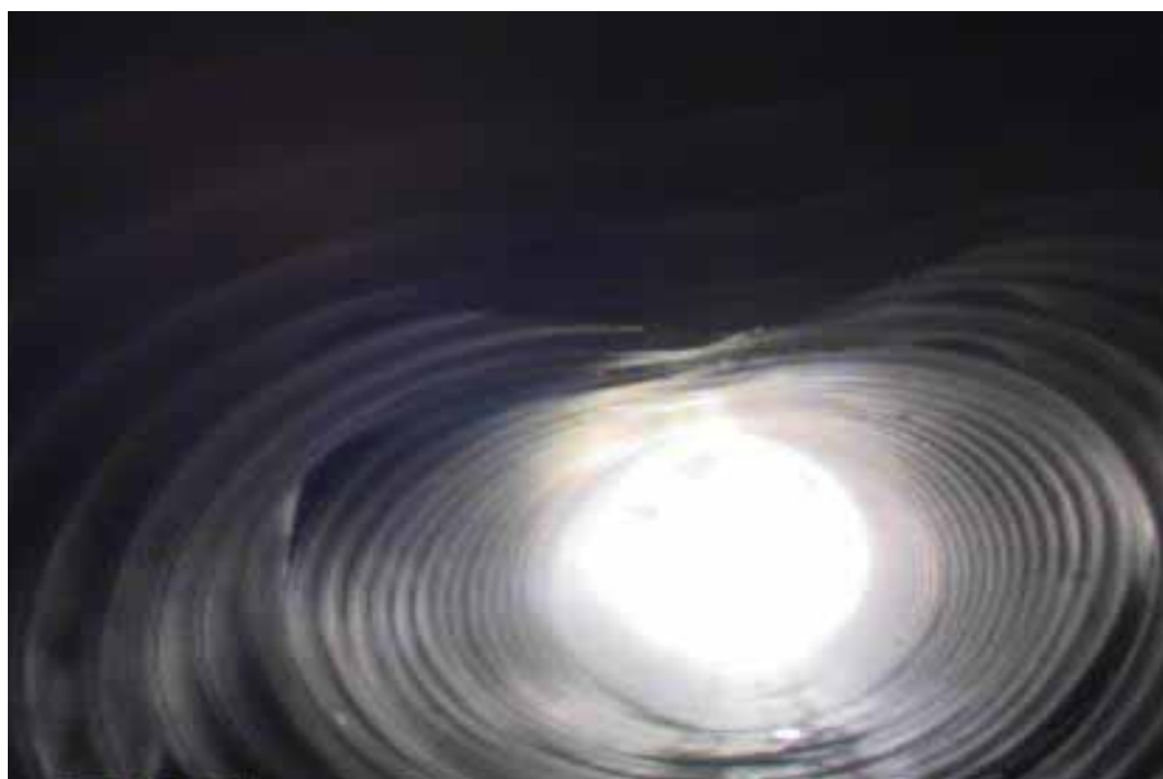
Figure 266 Corrugation growth, excessive deformation, cracking/fracture, and inverse curvature failures for Pipeline No. 2 (Site No. 1: Route 101)
