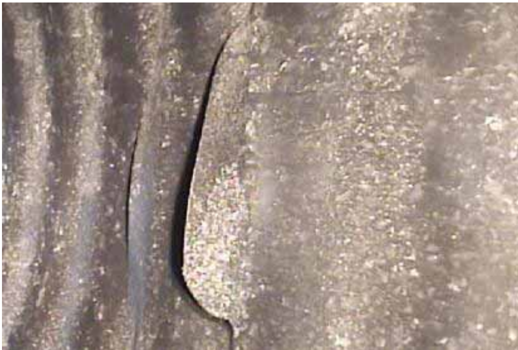
Figure 378 Cracking/fracture failure for Pipeline No. 9 (Site No. 2: Silver Creek Parkway)
