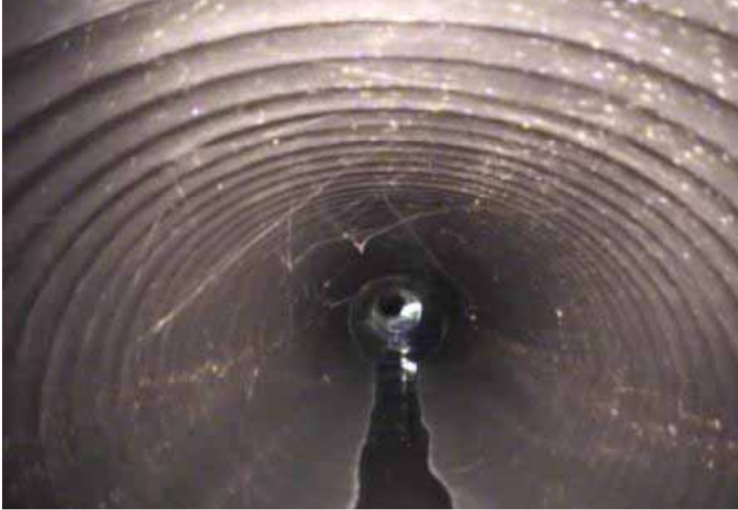
Figure 221 View of the corrugation growth failure for pipeline No. 7 (Site No. 2: Wichita)
