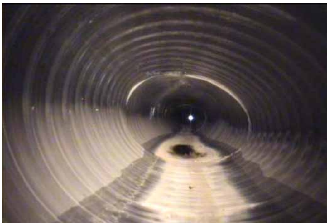
Figure 25 Excessive deformation and corrugation growth failure modes for pipeline No. 1 (Site No. 1: San Antonio - HW 1604 and 1560)
