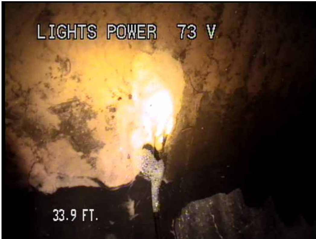
Figure 484 View of the leaking at the joint for pipeline No. 2 (Site No. 1: Orlando)
