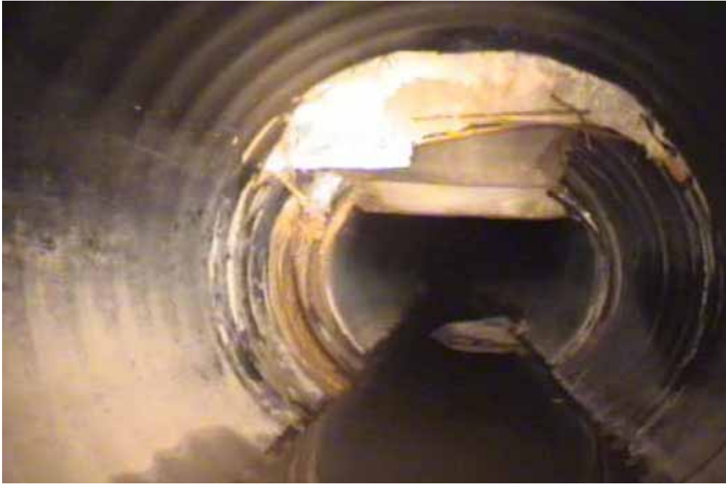
Figure 47 Major joint displacement, major cracking/fracture and inverse curvature failures for pipeline No. 19 (Segment 2) (Site No. 8: Houston – Fennell)
