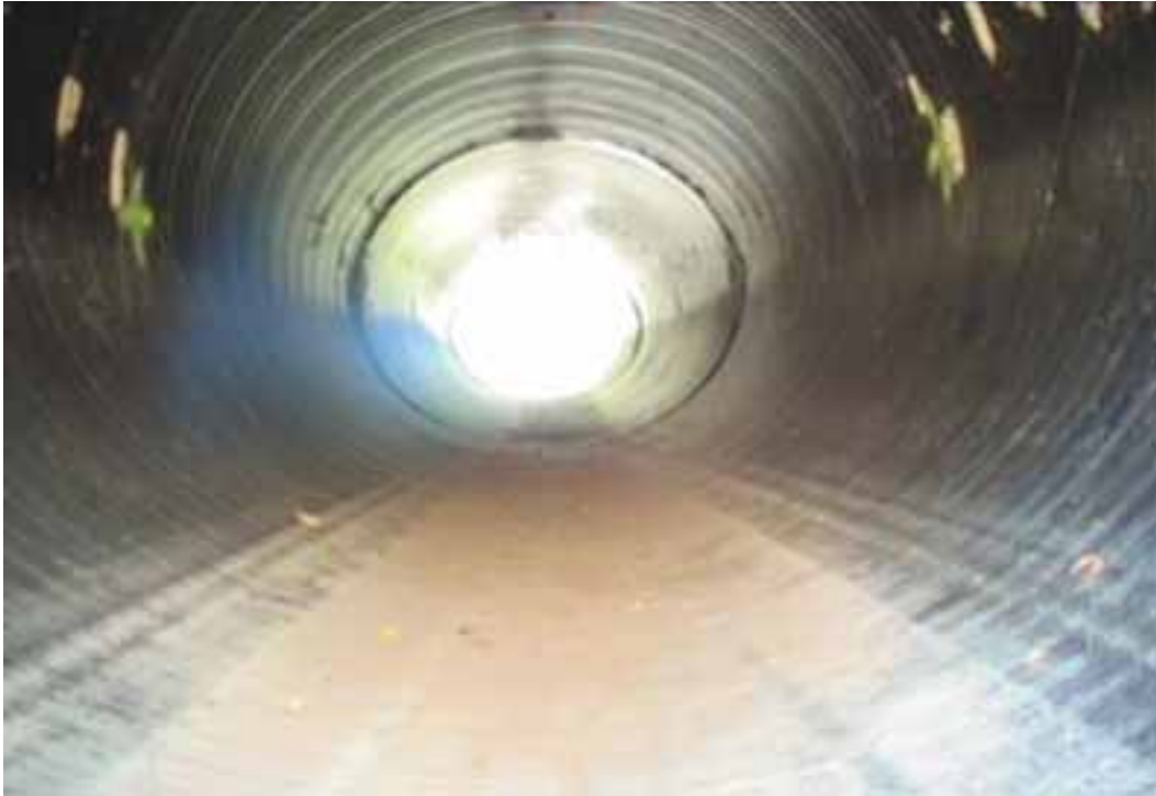
Figure 232 Corrugation growth for pipeline No. 4 (Site No. 2: St Claire County – Route B)
