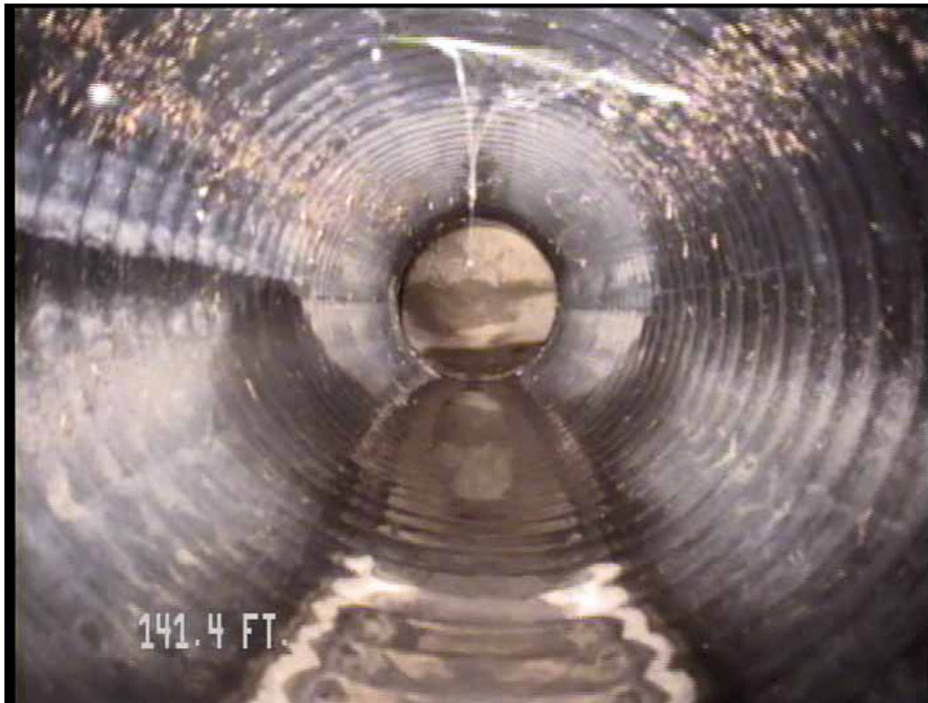
Figure 584 View of corrugation growth failure at the end for pipeline No. 15 (Site No. 2: Apopka)
