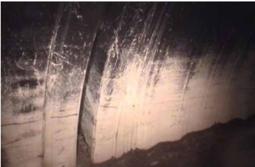
Figure 72 View of major joint displacement failures for pipeline No. 7 (Site No. 4: Wendell – Huntzell Main Drive)
