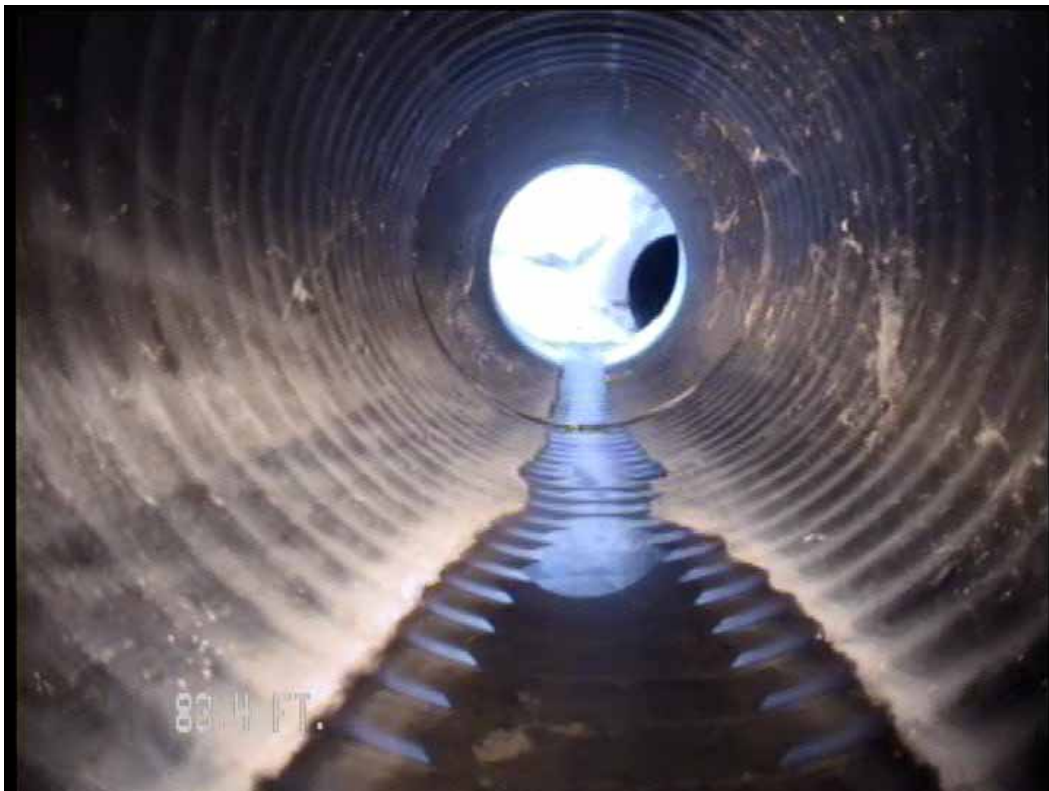
Figure 578 View of the corrugation growth failure at the end for pipeline No. 14 (Site No. 2: Apopka)
