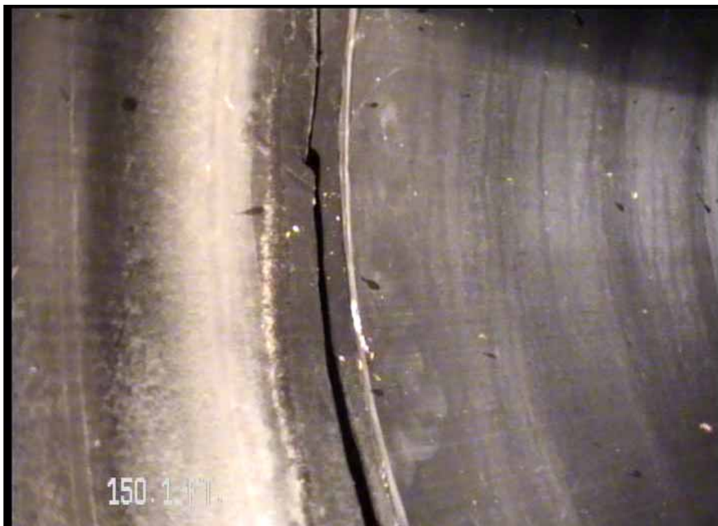
Figure 559 View of the major joint displacement failure for pipeline No. 11 (Site No. 2: Apopka)
