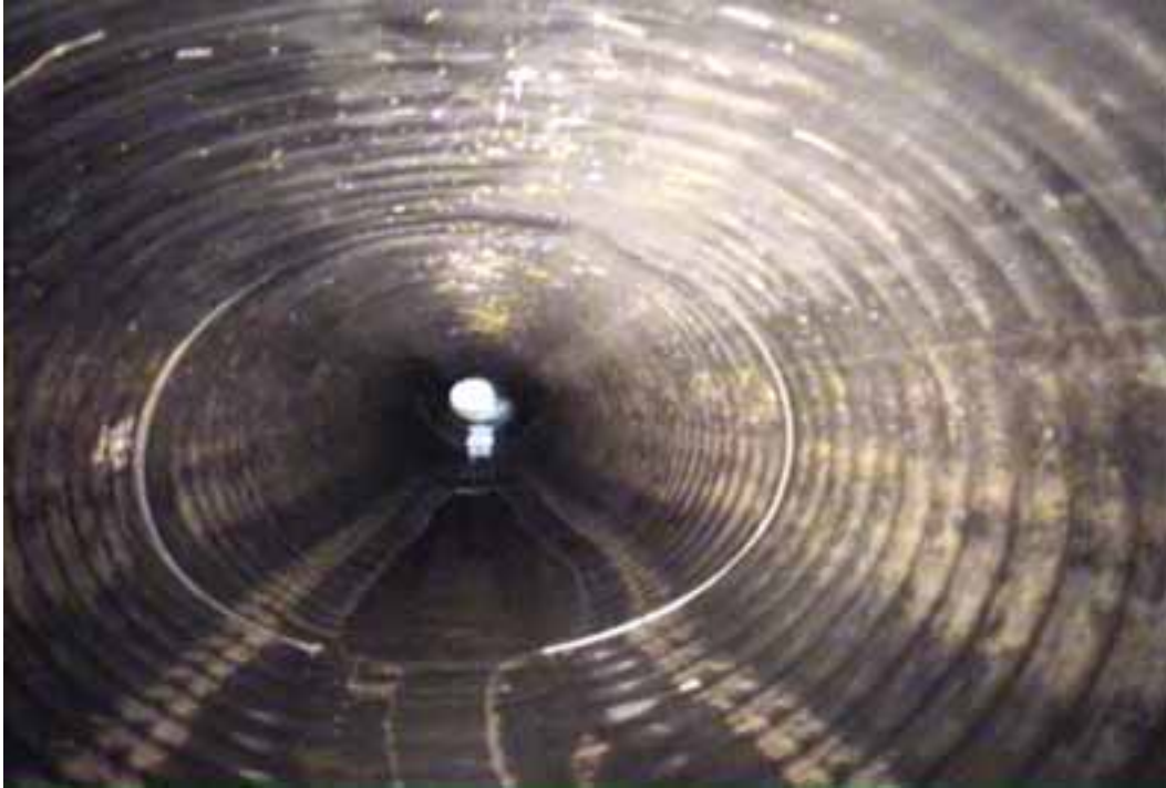
Figure 140 View of excessive deformation failure for pipeline No. 12 (Site No. 5: Staunton)
