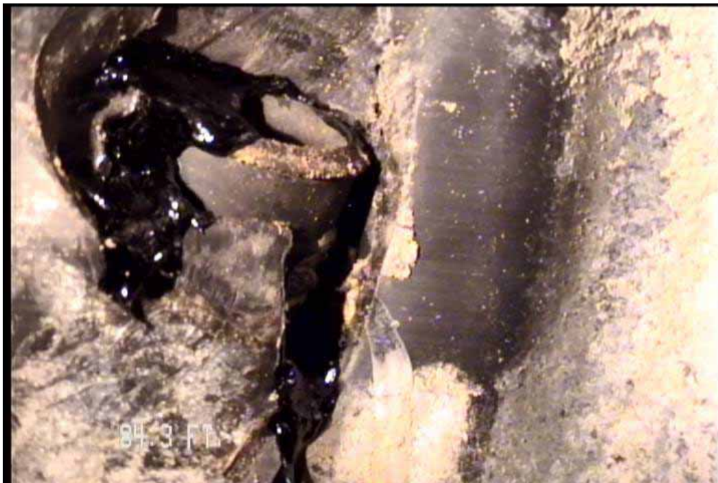
Figure 558 View of cracking/fracture failures for pipeline No. 11 (Site No. 2: Apopka)
