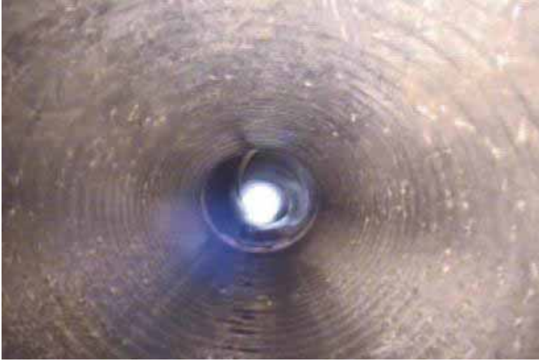
Figure 257 Corrugation growth failure for Pipeline No. 1 (Site No. 1: Route 101)
