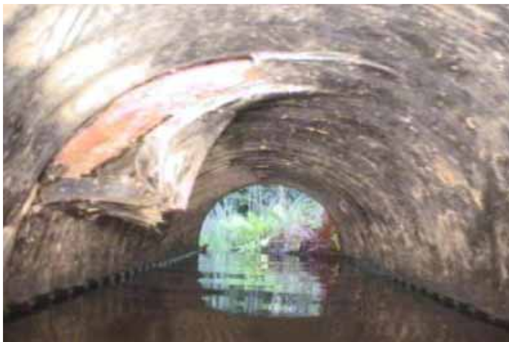
Figure 328 Cracking/fracture and corrugation growth failure for Pipeline No. 20 (Site No. 2: Route 36)
