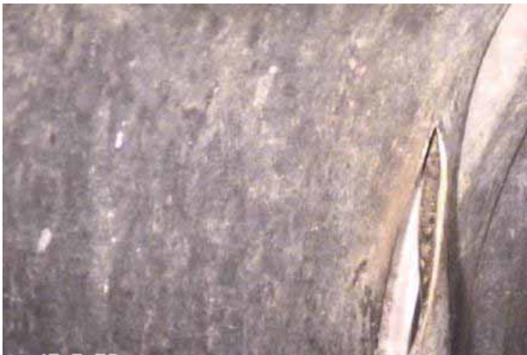
Figure 259 Cracking/fracture failure for Pipeline No. 2 (Site No. 1: Route 101)
