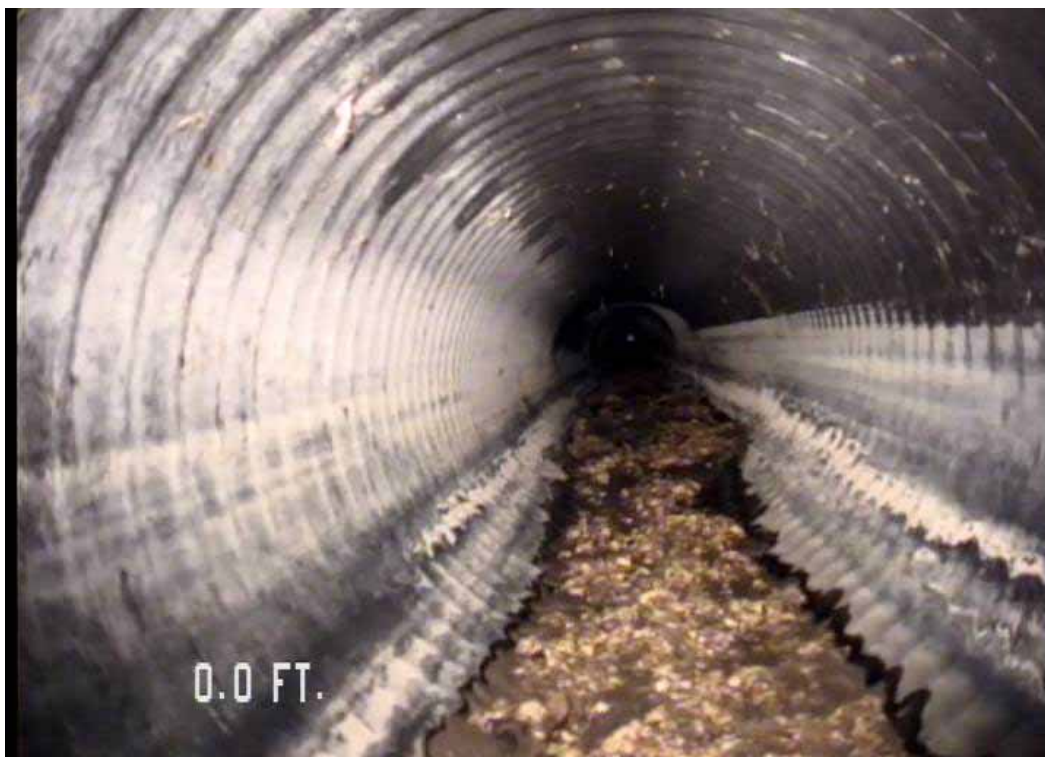
Figure 551 View of the corrugation growth failure at the opening for pipeline No. 11 (Site No. 2: Apopka)
