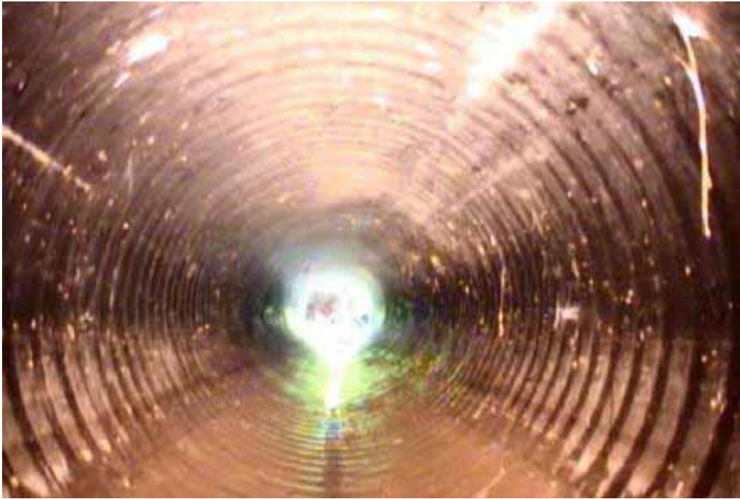
Figure 441 Corrugation growth failure for Pipeline No. 16 (Site No. 9: Driveway off Main St. L’Anse)
