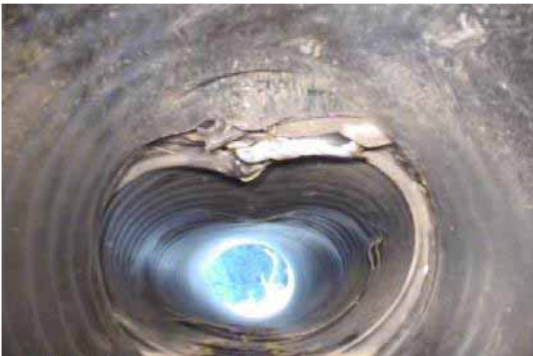
Figure 262 Cracking/fracture, inverse curvature, and excessive deformation failures for Pipeline No. 2 (Site No. 1: Route 101)
