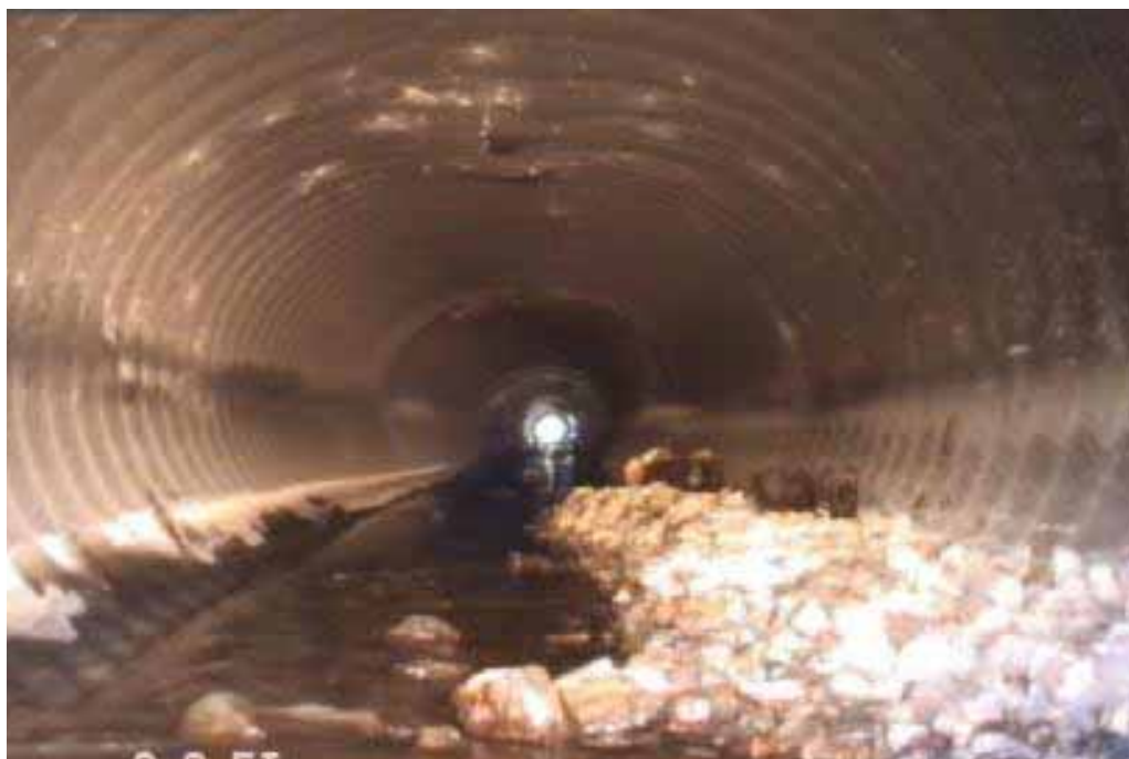
Figure 368 Corrugation growth, cracking/fracture, and inverse curvature failure and debris for Pipeline No. 6 (Site No. 1: Legacy Parkway)
