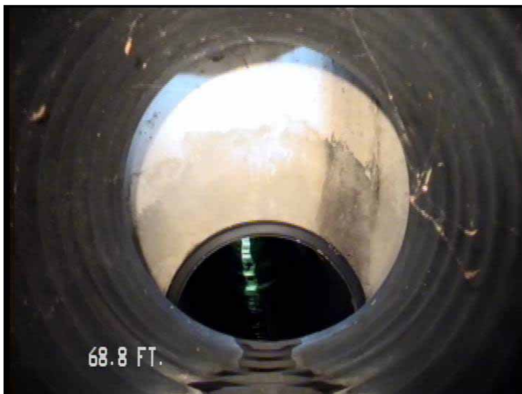
Figure 565 View of the corrugation growth failure at the end for pipeline No. 12 (Site No. 2: Apopka)
