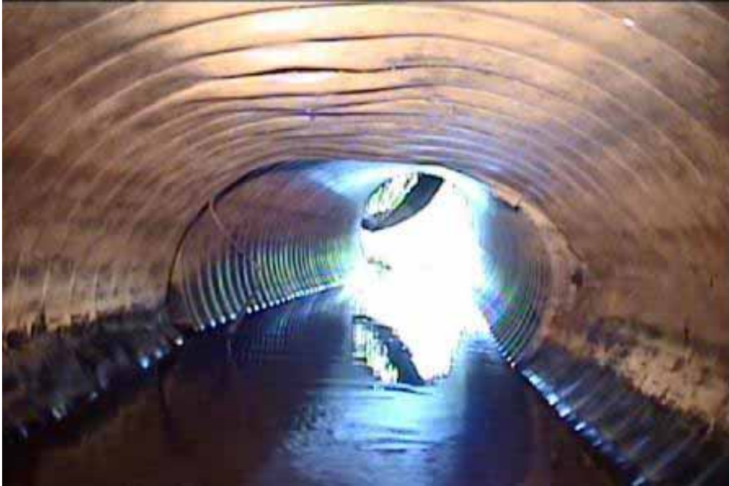
Figure 460 Excessive deformation, inverse curvature, and corrugation growth failure for Pipeline No. 23 (Site No. 12: 48 th Avenue)
