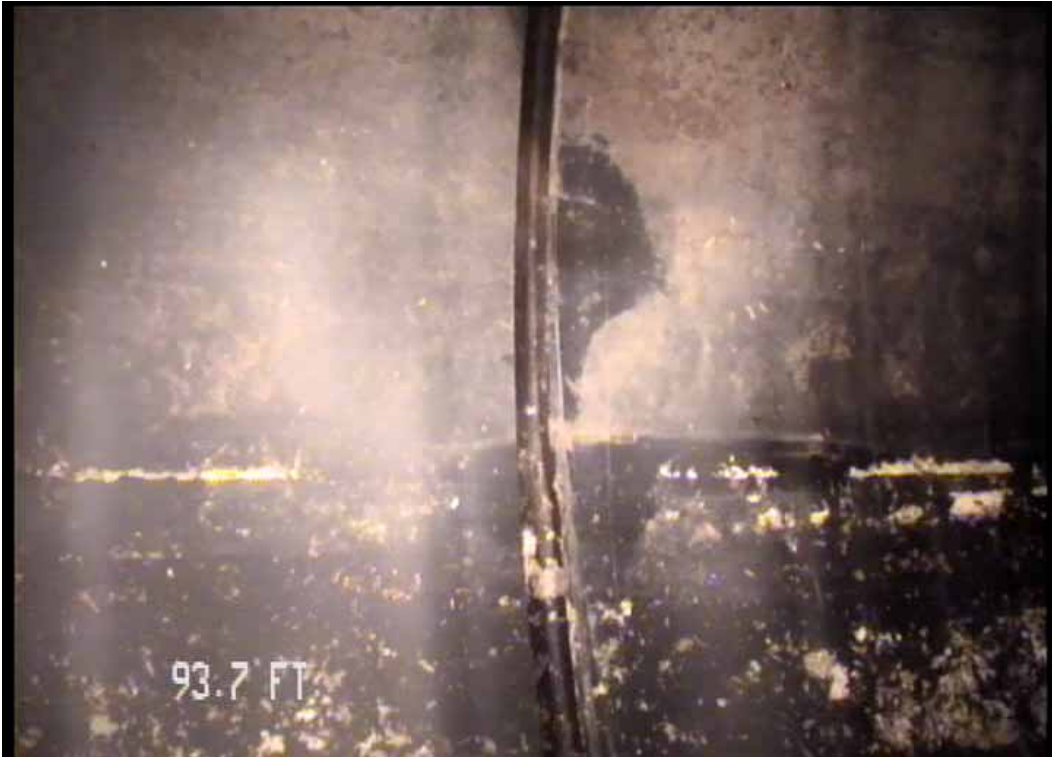
Figure 507 View of the major joint displacement failure for pipeline No. 6
