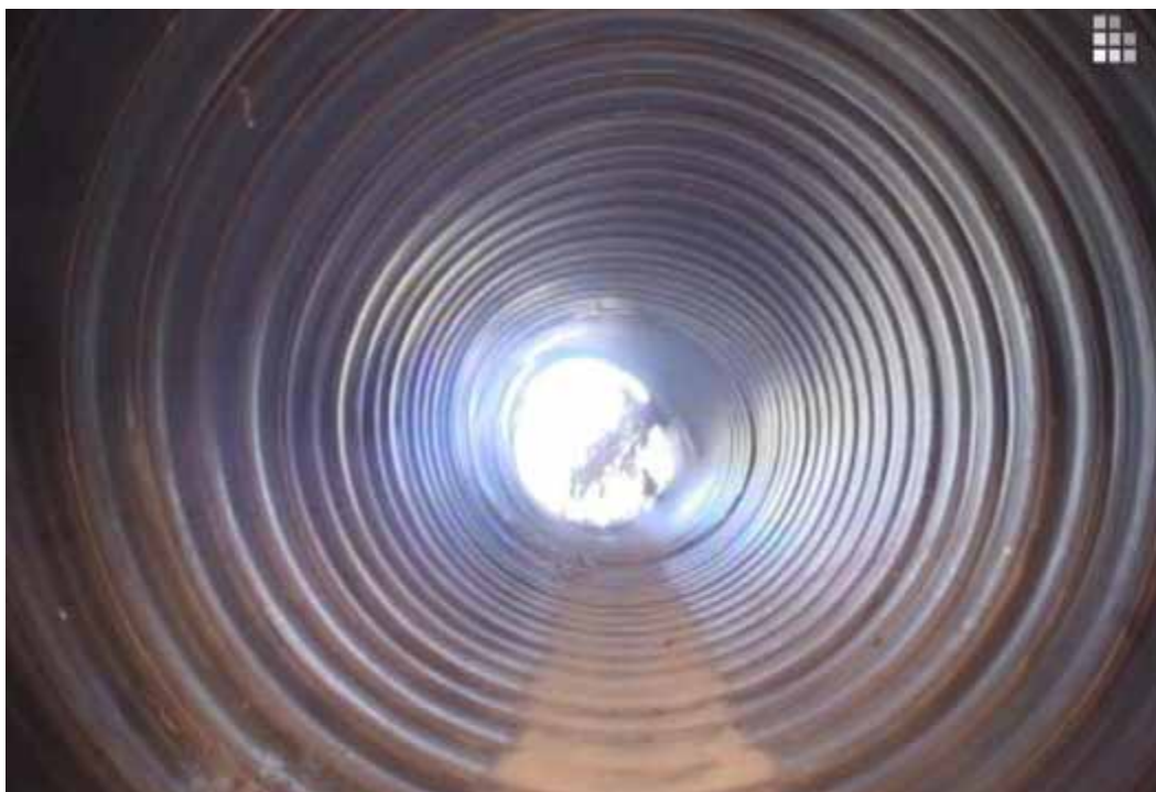
Figure 30 Corrugation growth and excessive deformation failures for pipeline No. 3 (Site No. 1: San Antonio - HW 1604 and 1560)
