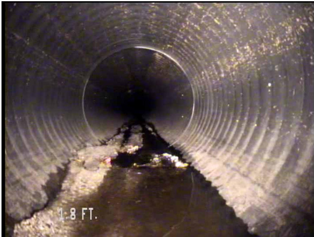
Figure 491 View of the corrugation growth failure for pipeline No. 3 (Site No. 1: Orlando)
