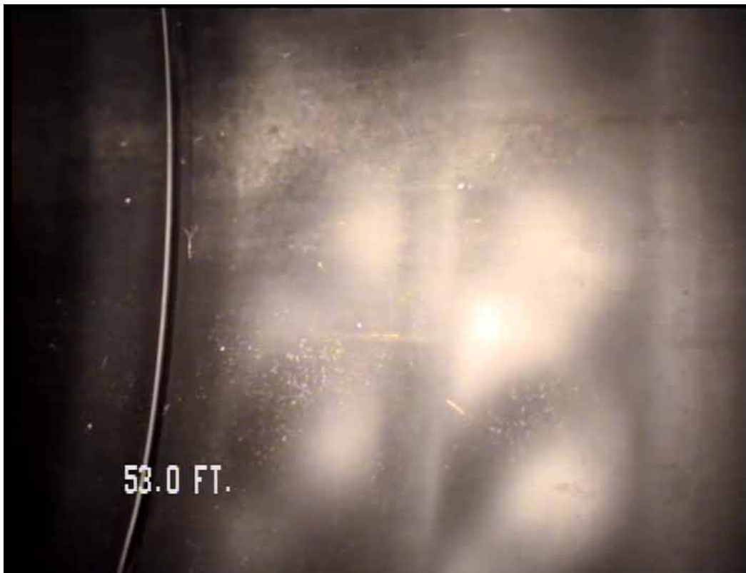
Figure 517 View of the minor joint displacement and buckling failure for pipeline No. 7 (Site No. 1: Orlando)
