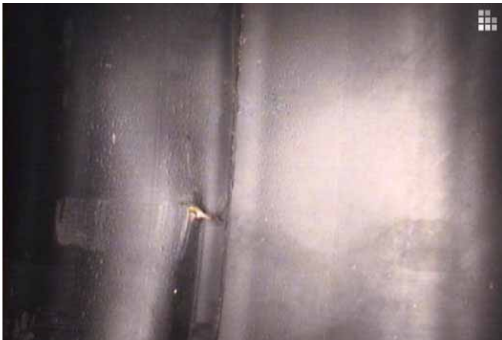
Figure 170 View of cracking failure for pipeline No. 12 (Site No. 3: Blaine - Xylite)
