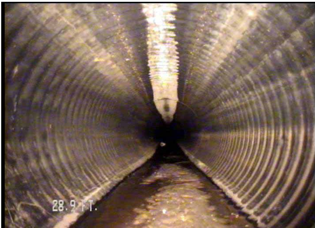
Figure 527 View of corrugation growth failure for pipeline No. 8 (Site No. 1: Orlando)
