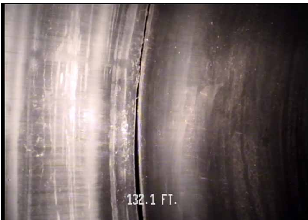
Figure 545 View of minor joint displacement for pipeline No. 10 (Site No. 2: Apopka)
