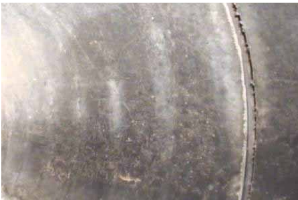
Figure 260 Cracking/fracture failure for Pipeline No. 2 (Site No. 1: Route 101)
