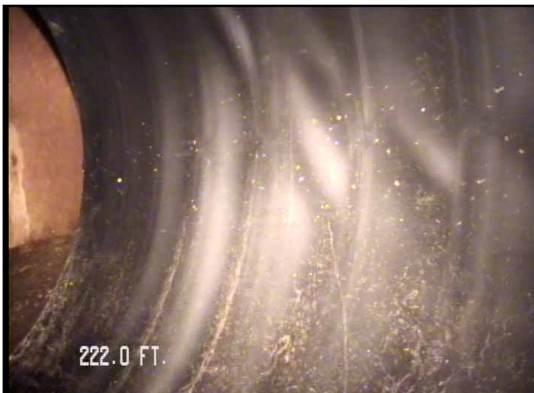
Figure 498 View of the buckling failure for pipeline No. 3 (Site No. 1: Orlando)
