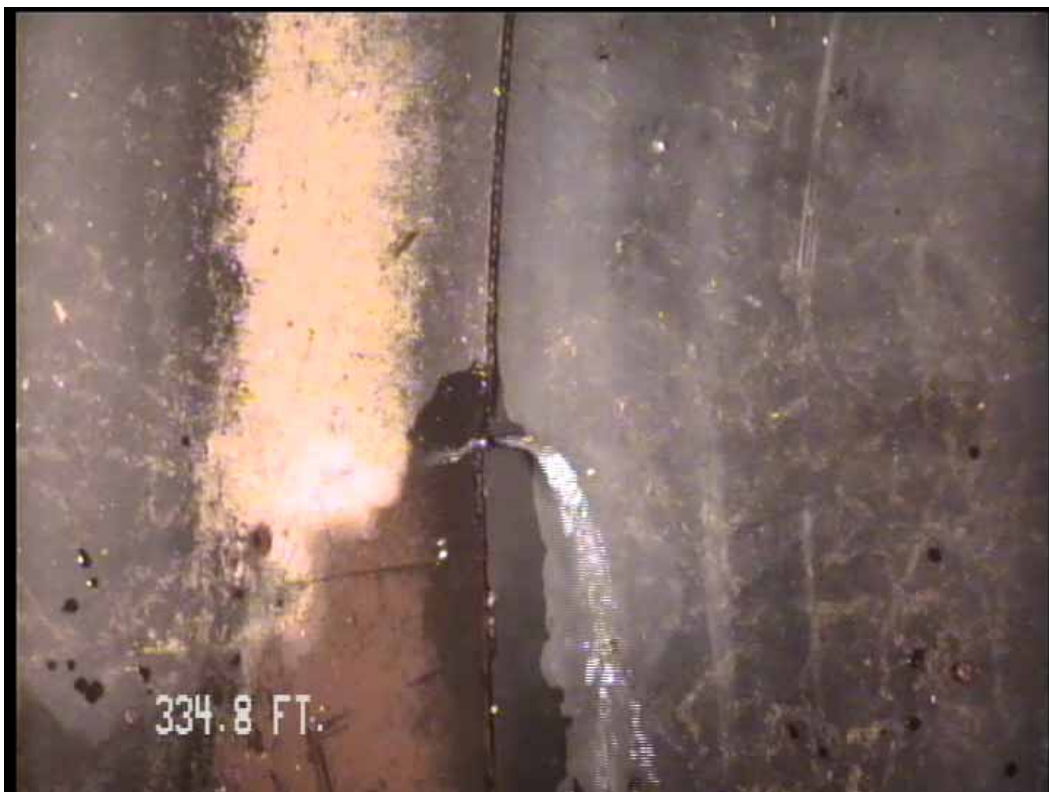
Figure 500 View of the leaking at the joint for pipeline No. 3 (Site No. 1: Orlando)
