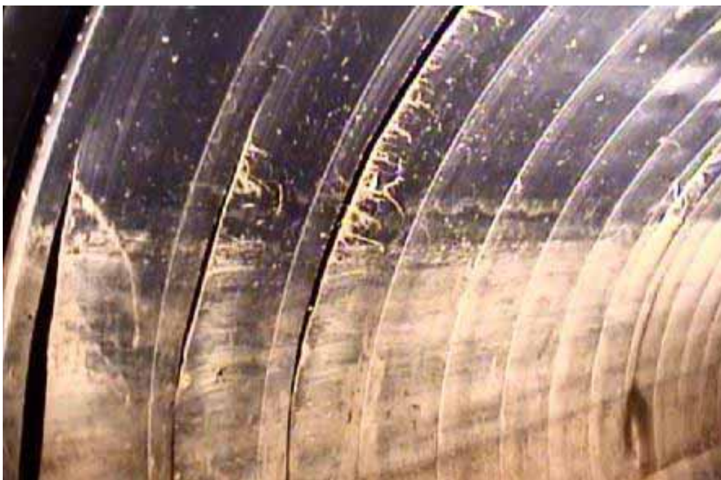
Figure 455 Buckling and corrugation growth failure for Pipeline No. 23 (Site No. 12: 48 th Avenue)
