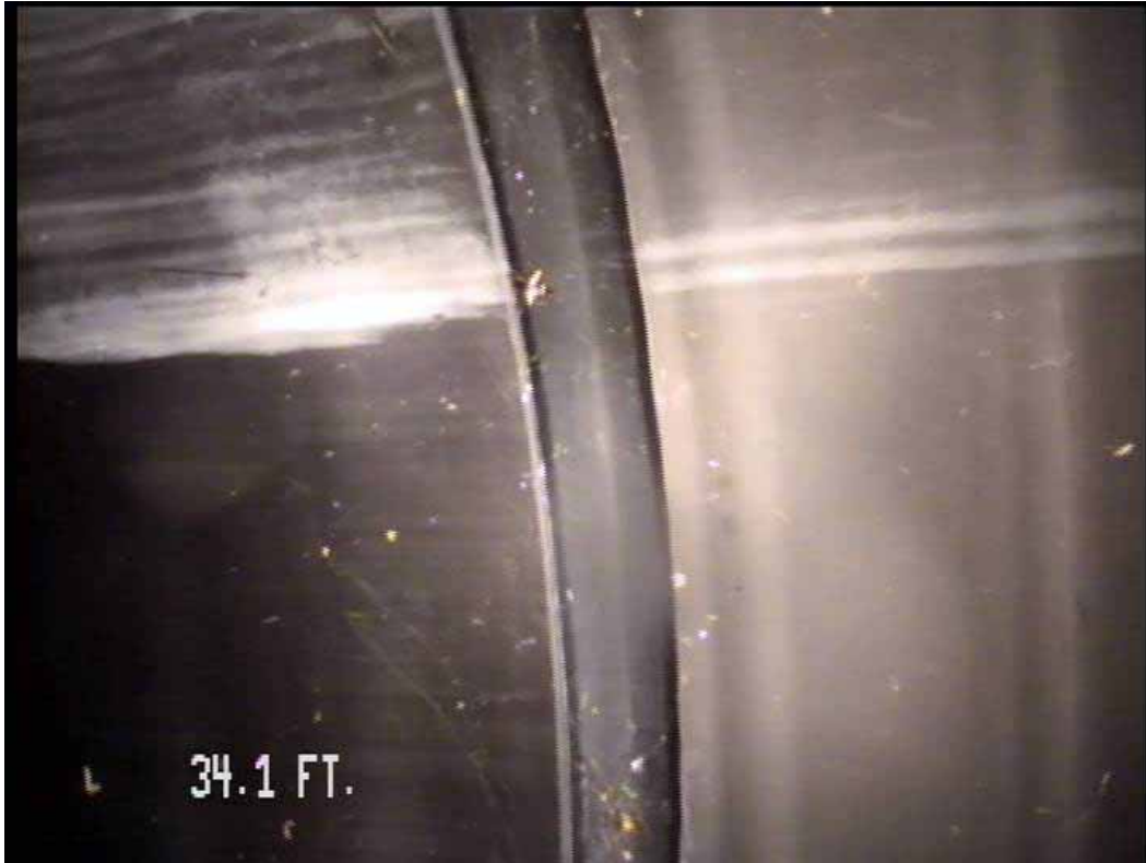
Figure 575 View of the major joint displacement failure for pipeline No. 14 (Site No. 2: Apopka)
