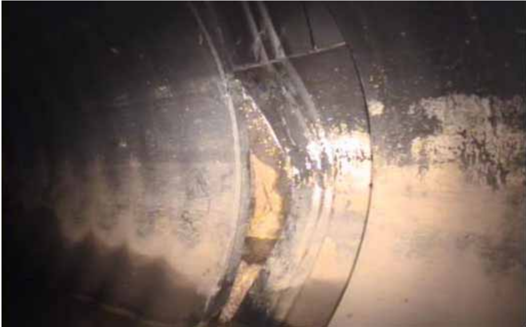
Figure 49 Major joint displacement, minor cracking/fracture and inverse curvature failures for pipeline No. 19 (Segment 2) (Site No. 8: Houston – Fennell)
