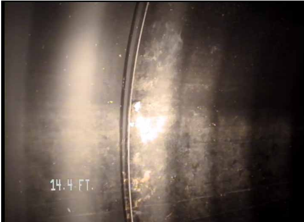
Figure 515 View of the minor joint displacement failure for pipeline No. 7 (Site No. 1: Orlando)
