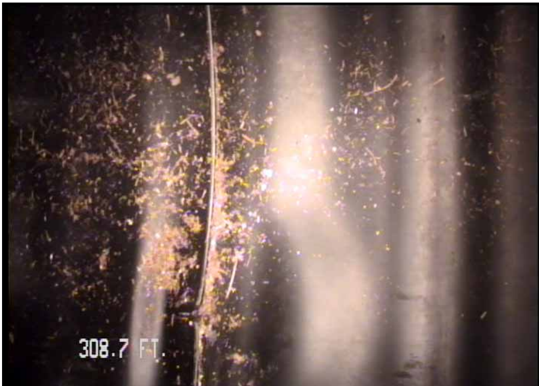
Figure 522 View of the buckling/cracking failures at the joint for pipeline No. 7 (Site No. 1: Orlando)
