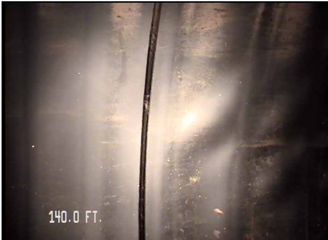
Figure 539 View of the minor joint displacement and buckling failures for pipeline No. 9 (Site No. 1: Orlando)
