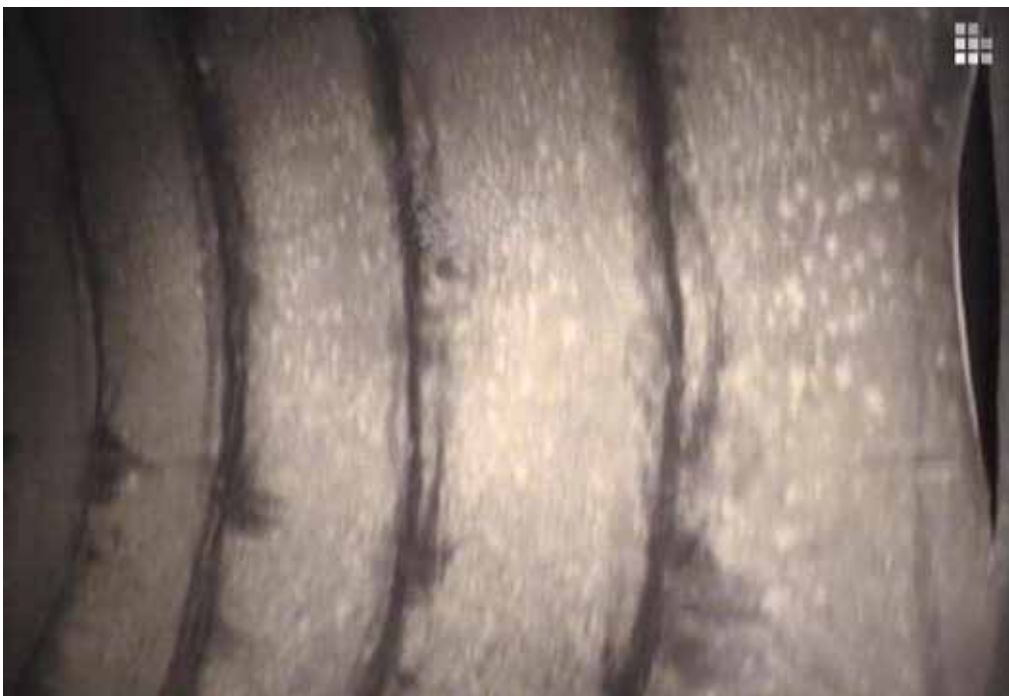
Figure 202 View of cracking/fracture failure for pipeline No. 31 (Site No. 9: Rochester)
