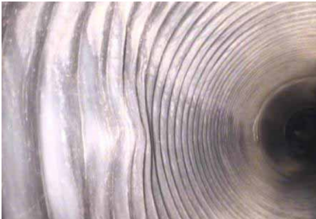
Figure 212 View of inverse curvature failure for pipeline No. 4 (Site No. 1: Lenexa)
