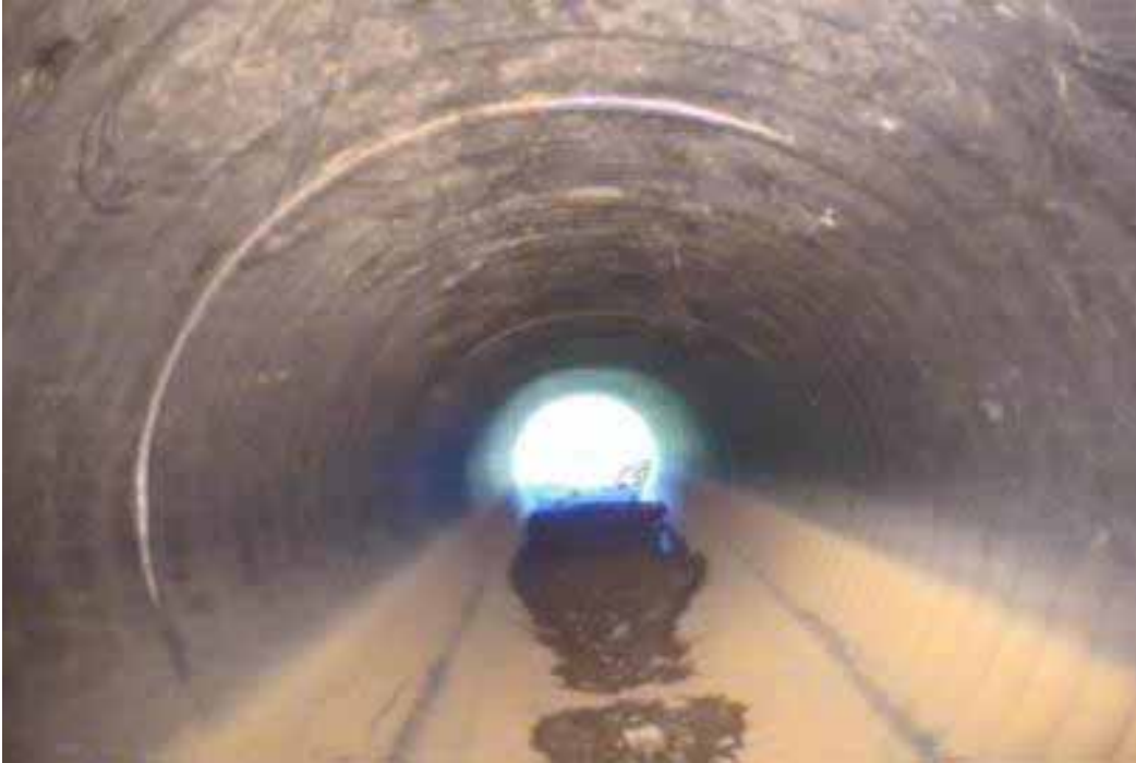
Figure 283 Cracking/fracture and corrugation growth failure for Pipeline No. 5 (Site No. 1: Route 101)
