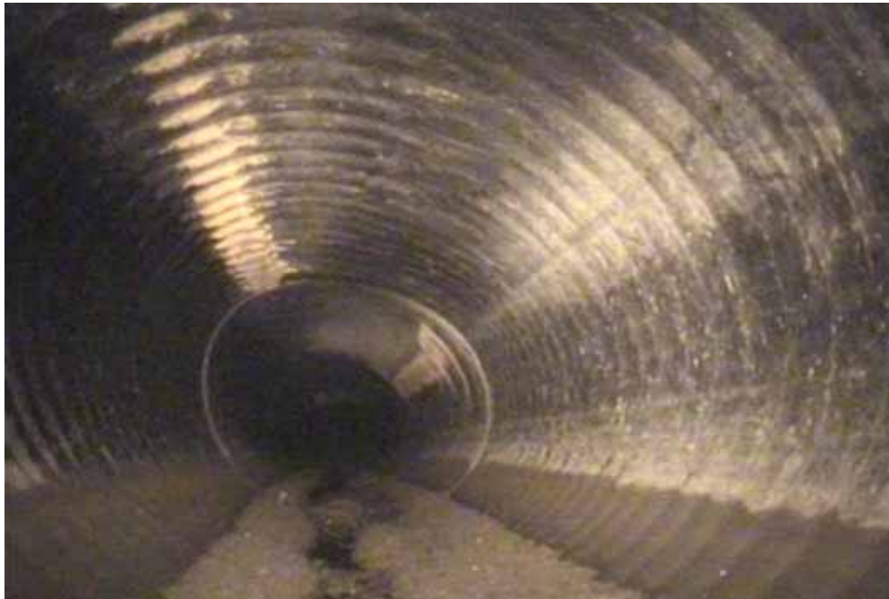
Figure 108 View of the corrugation growth failure for pipeline No. 1 (Site No. 1: Chesterfield - Commonwealth Pkwy)
