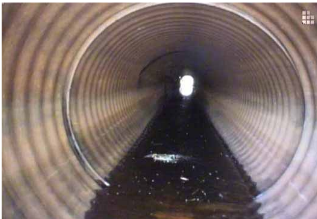
Figure 174 View of corrugation growth and excessive deformation failures for pipeline No. 15 (Site No. 5: McGregor)
