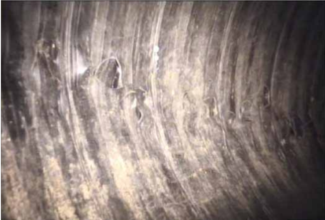
Figure 104 View of buckling and cracking failures for pipeline No. 11 (Site No. 6: Rockingham – Love Ln)
