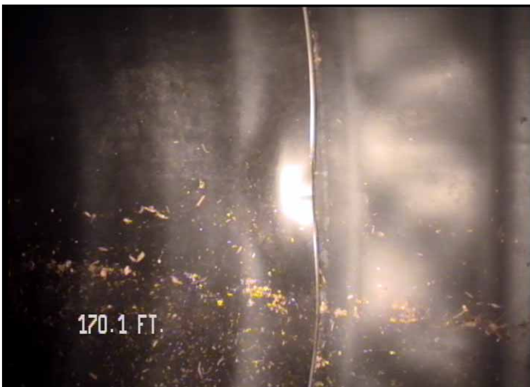
Figure 520 View of the buckling failure at the joint for pipeline No. 7 (Site No. 1: Orlando)
