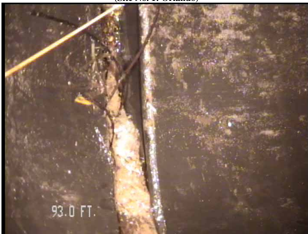
Figure 487 View of the major joint displacement failure for pipeline No. 2 (Site No. 1: Orlando)
