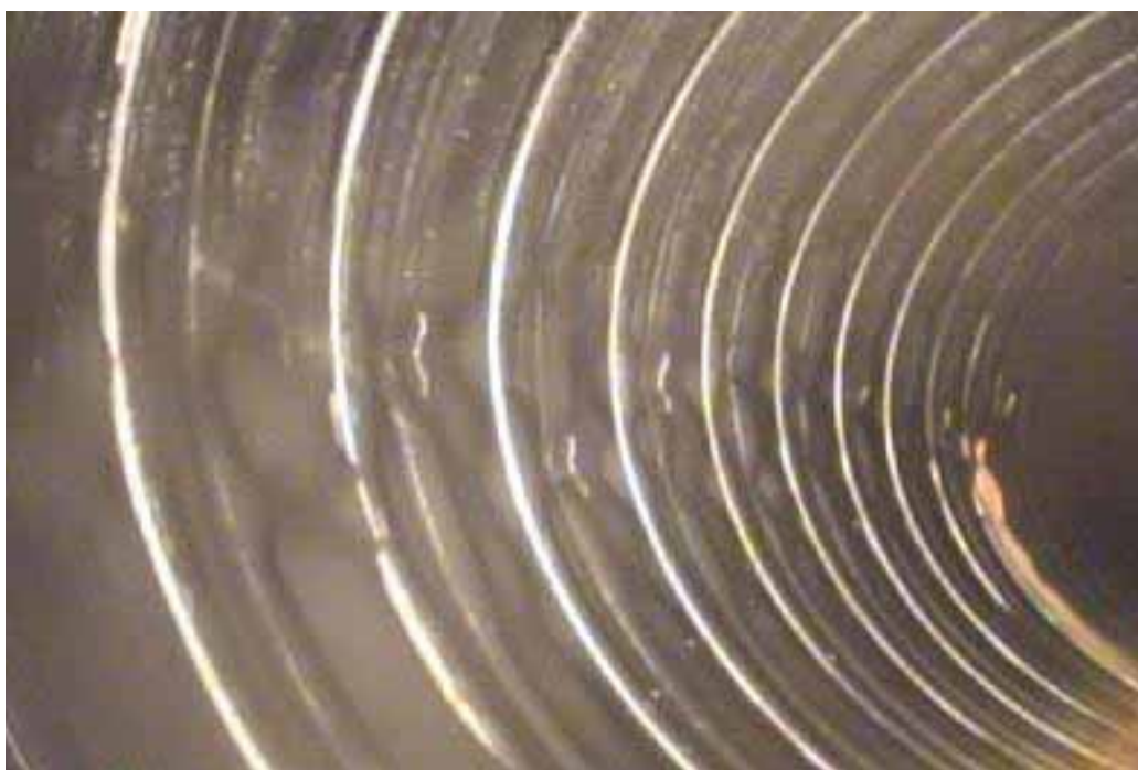
Figure 397 Corrugation growth and buckling failure for Pipeline No. 4 (Site No. 4: Horton Parkway)
