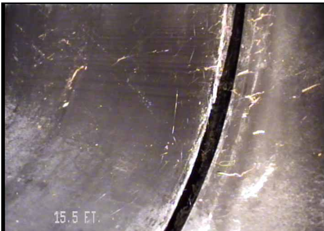
Figure 556 View of the major joint displacement failure for pipeline No. 11 (Site No. 2: Apopka)
