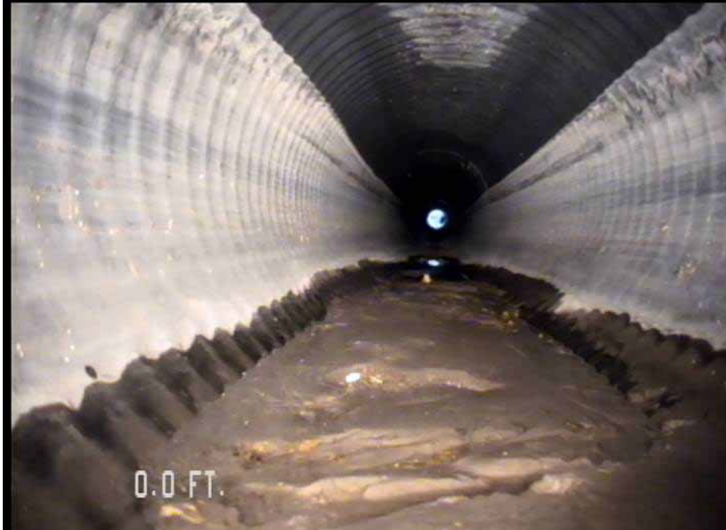
Figure 573 View of the corrugation growth and heavy build up of sediment at the opening for pipeline No. 14 (Site No. 2: Apopka)
