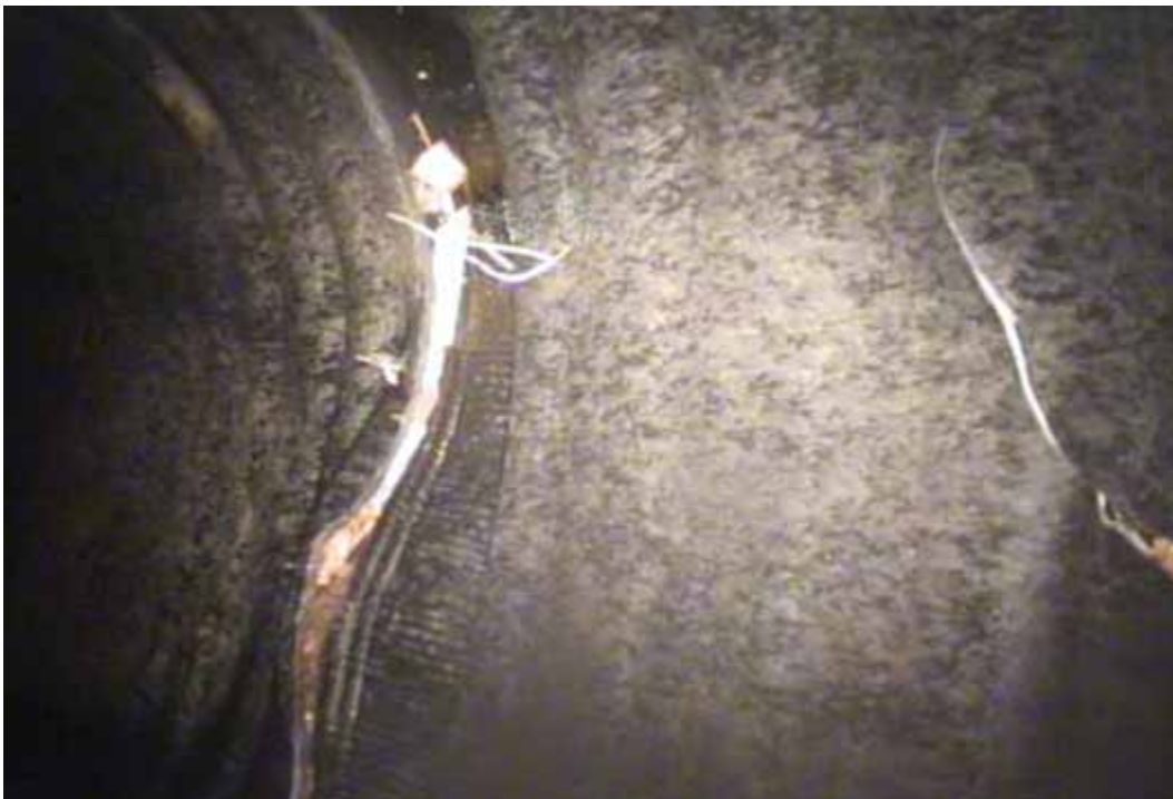
Figure 51 Joint displacement, buckling and cracking/fracture failures for pipeline No. 20 (Segment 1) (Site No. 8: Houston – Fennell)
