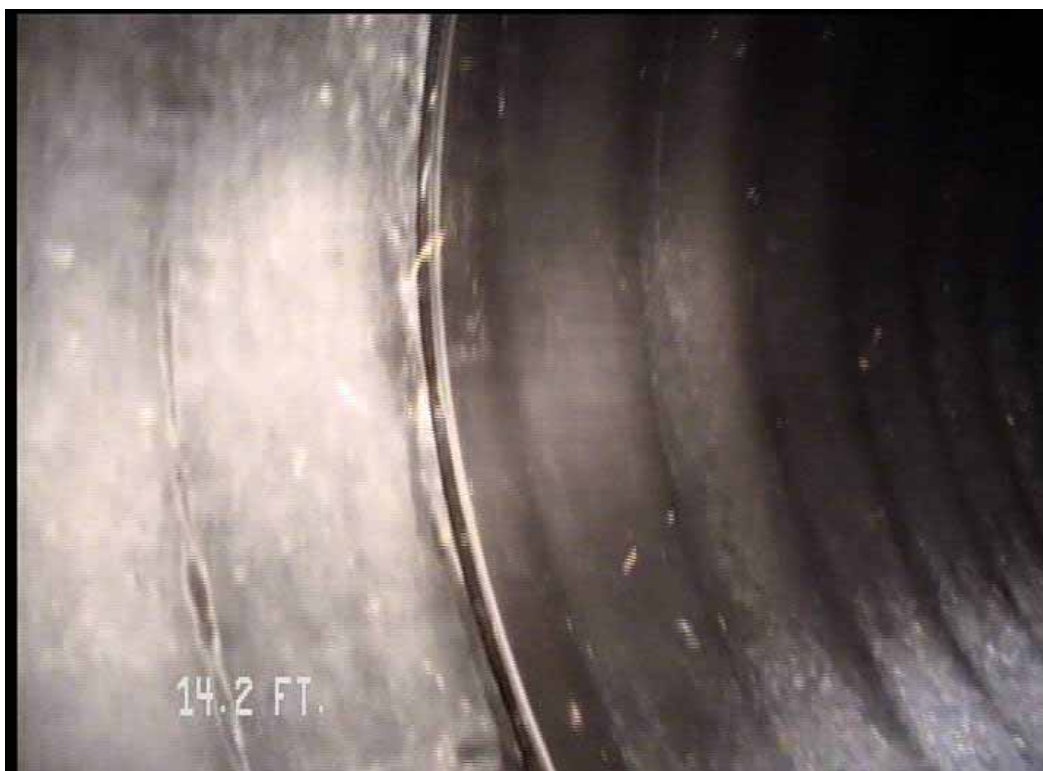
Figure 563 View of major joint displacement failure for pipeline No. 12 (Site No. 2: Apopka)
