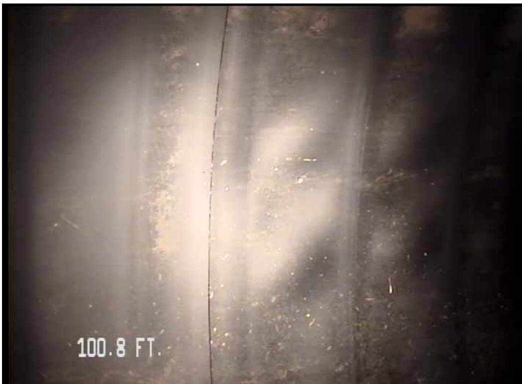
Figure 538 View of the buckling failure for pipeline No. 9 (Site No. 1: Orlando)
