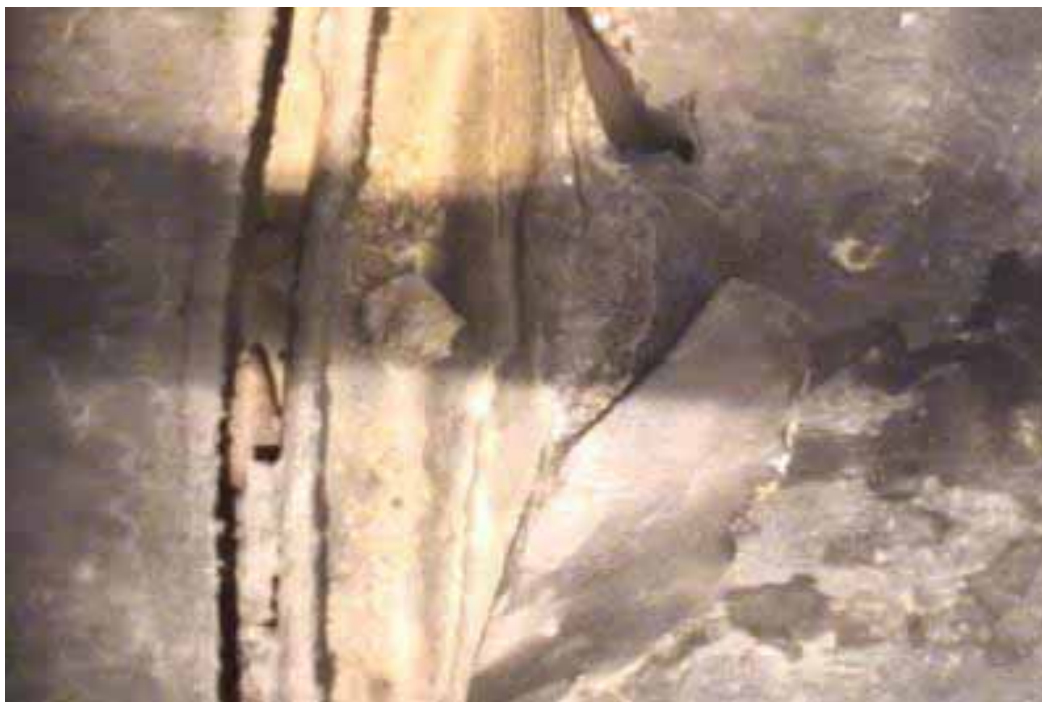
Figure 252 Cracking/fracture failure for Pipeline No. 1 (Site No. 1: Route 101)
