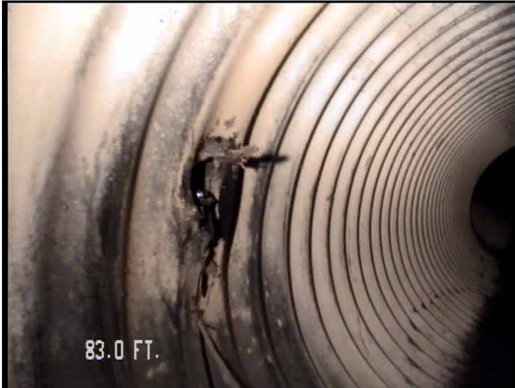
Figure 557 View of corrugation growth/cracking/fracture failures for pipeline No. 11 (Site No. 2: Apopka)
