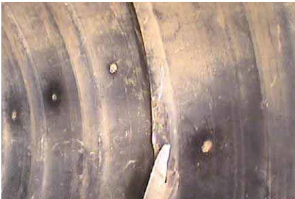
Figure 417 Cracking/fracture failure for Pipeline No. 7 (Site No. 7: West Island Road)
