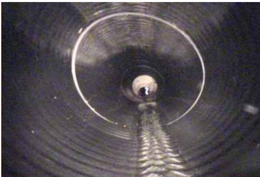
Figure 138 View of excessive deformation failure for pipeline No. 11 (Site No. 5: Staunton)
