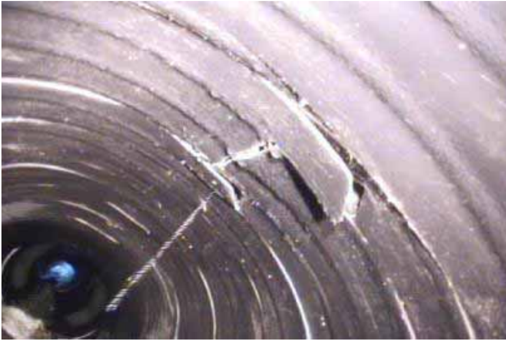
Figure 340 Cracking/fracture and corrugation growth failure for Pipeline No. 23 (Site No. 2: Route 36)
