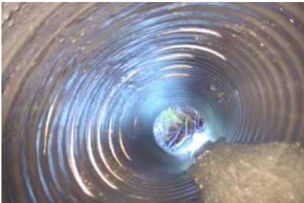
Figure 338 Cracking/fracture and corrugation growth failure for Pipeline No. 23 (Site No. 2: Route 36)
