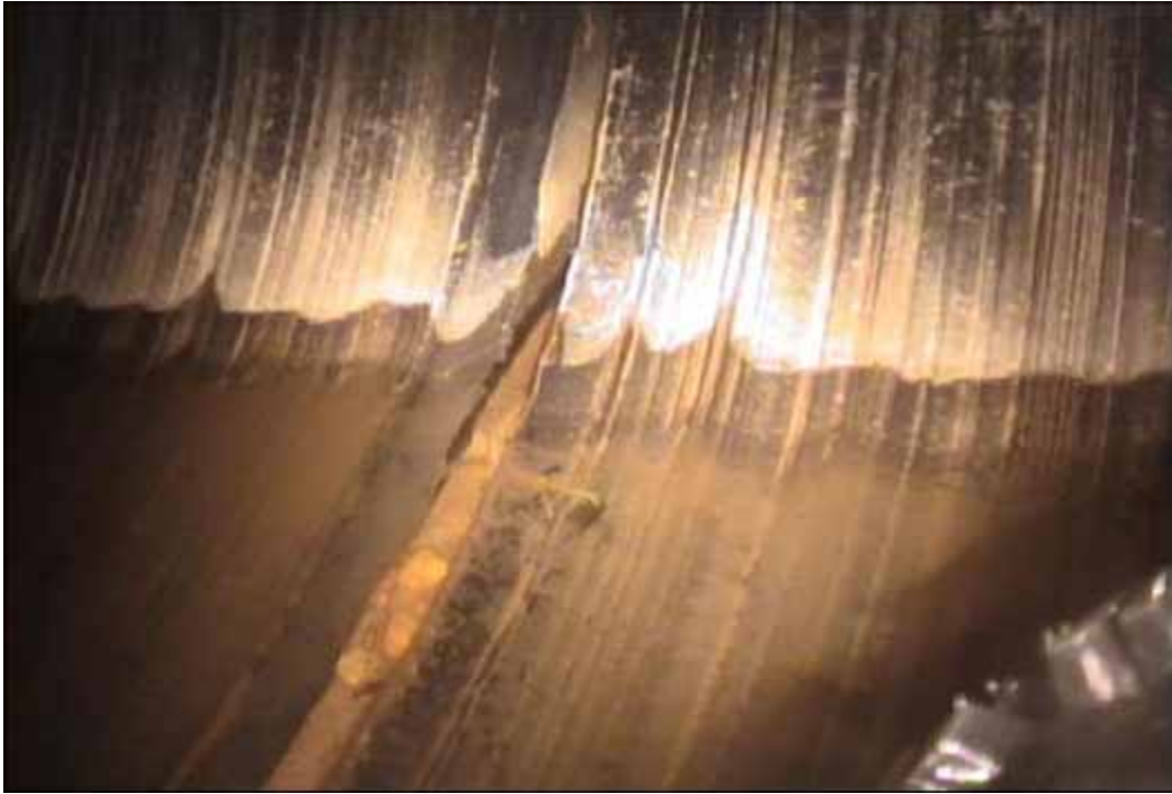
Figure 82 View of joint displacement failure for pipeline No. 10 (Site No. 6: Rockingham – Love Ln)
