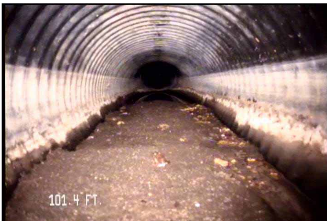
Figure 581 View of the excessive deformation, corrugation growth failures and heavy build up of sediment of pipeline No. 15 (Site No. 2: Apopka)
