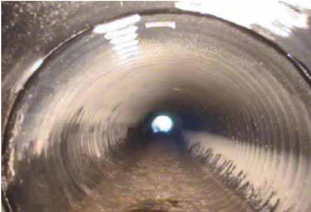
Figure 363 Excessive deformation failure (refer to Figure 362-d) for Pipeline No. 3 (Site No. 1: Legacy Parkway)
