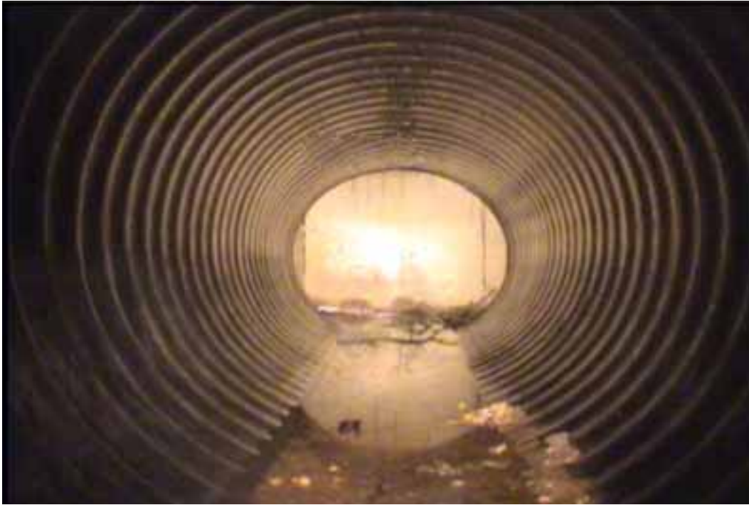
Figure 45 Excessive deformation and corrugation growth failures for pipeline No. 19 (Segment 1) (Site No. 8: Houston – Fennell)
