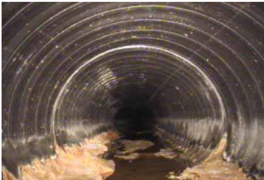
Figure 405 Corrugation growth failure and debris for Pipeline No. 6a (Site No. 6: Houghton County M92)
