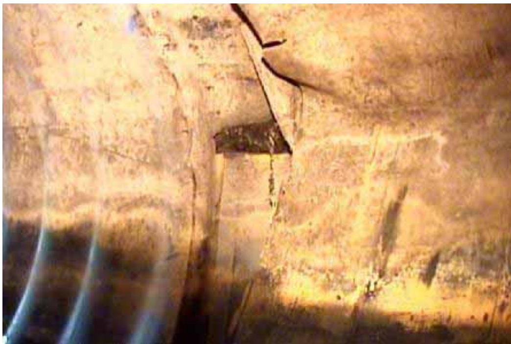
Figure 456 Buckling, cracking/fracture, joint displacement, and corrugation growth failure for Pipeline No. 23 (Site No. 12: 48 th Avenue)
