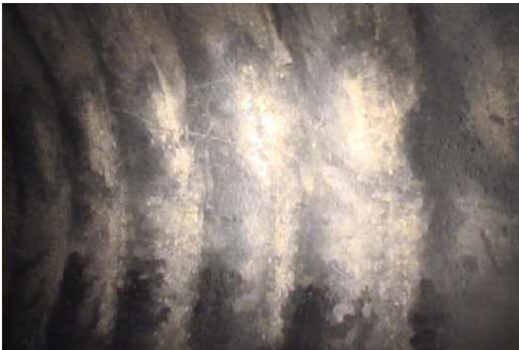
Figure 79 View of corrugation growth failure for pipeline No. 9 (Site No. 5: Hickory – Oxford School Rd)
