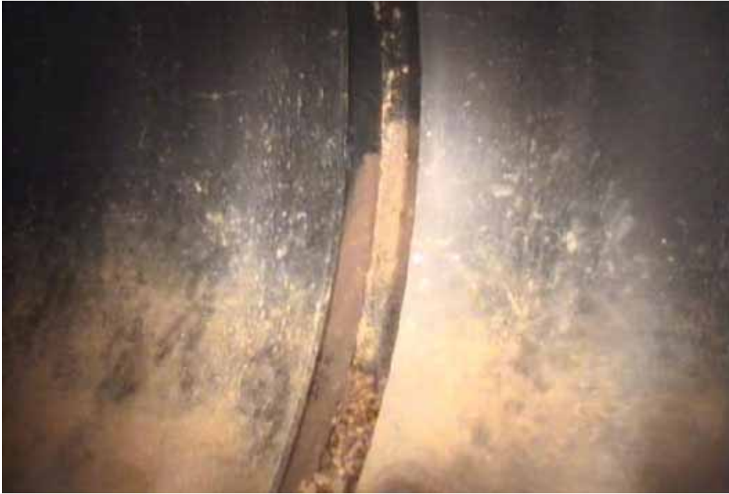
Figure 80 View of major joint displacement failure for pipeline No. 9 (Site No. 5: Hickory – Oxford School Rd)
