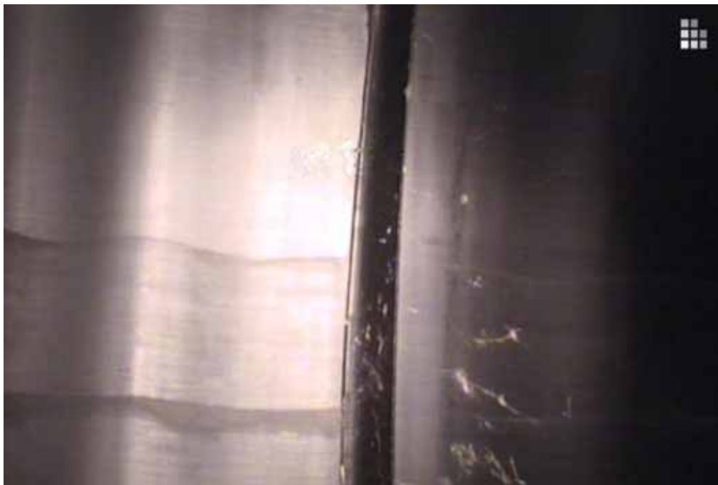
Figure 179 View of joint displacement failure for pipeline No. 18 (Site No. 6: Brooklyn Park - DuPont)
