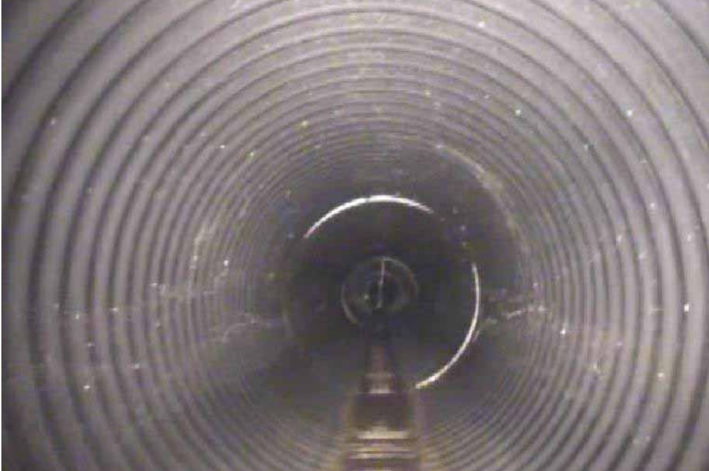
Figure 199 View of corrugation growth failure for pipeline No. 30 (Site No. 8: Fairmont)
