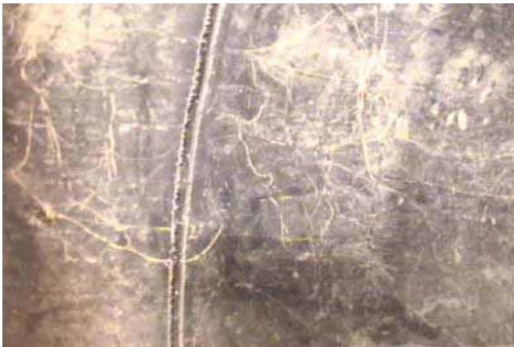
Figure 281 Cracking/fracture failure for Pipeline No. 5 (Site No. 1: Route 101)
