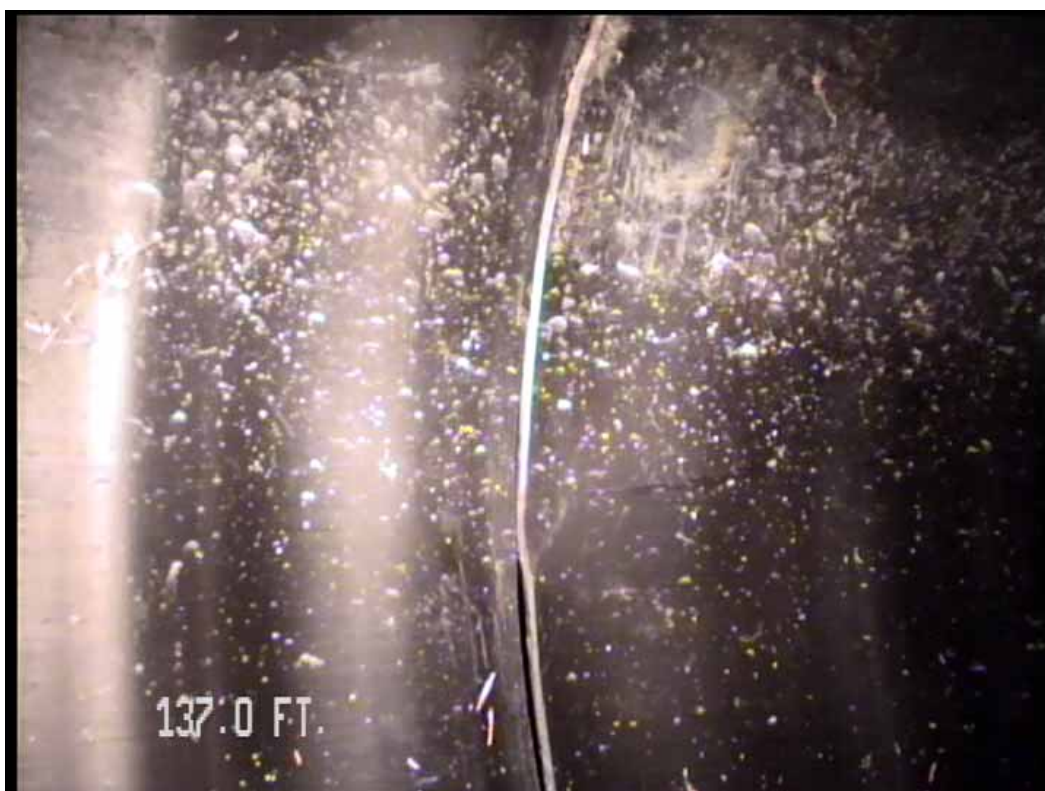
Figure 583 View of minor joint displacement for pipeline No. 15 (Site No. 2: Apopka)
