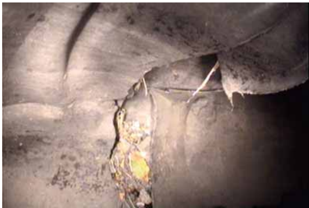
Figure 144 View of cracking/fracture failure for pipeline No. 15 (Site No. 6: Winchester)
