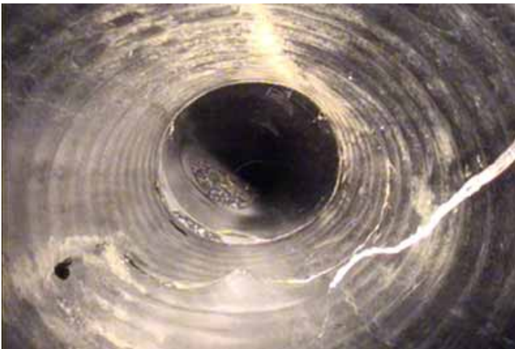
Figure 149 View of cracking/fracture failure for pipeline No. 16 (Site No. 6: Winchester)
