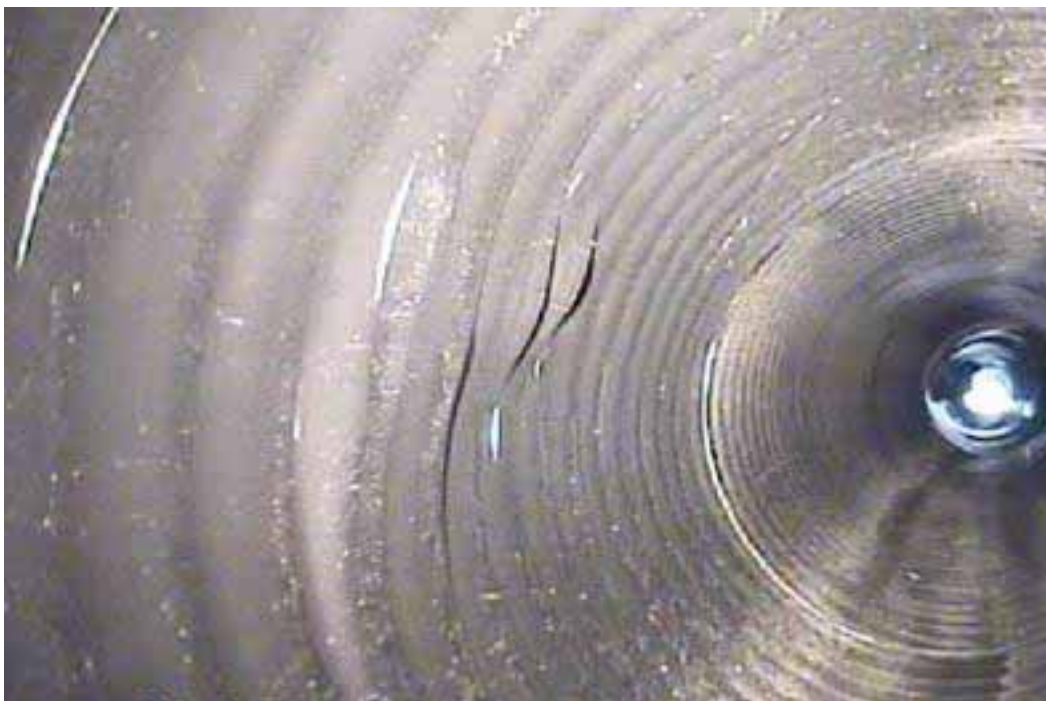
Figure 380 Cracking/fracture failure for Pipeline No. 9 (Site No. 2: Silver Creek Parkway)
