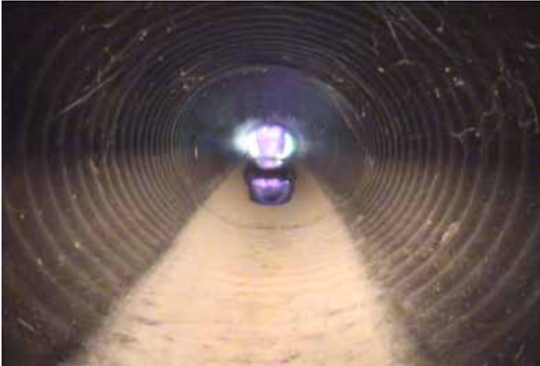
Figure 234 Corrugation growth for pipeline No. 5 (Site No. 3: Franklin County – Route FF)
