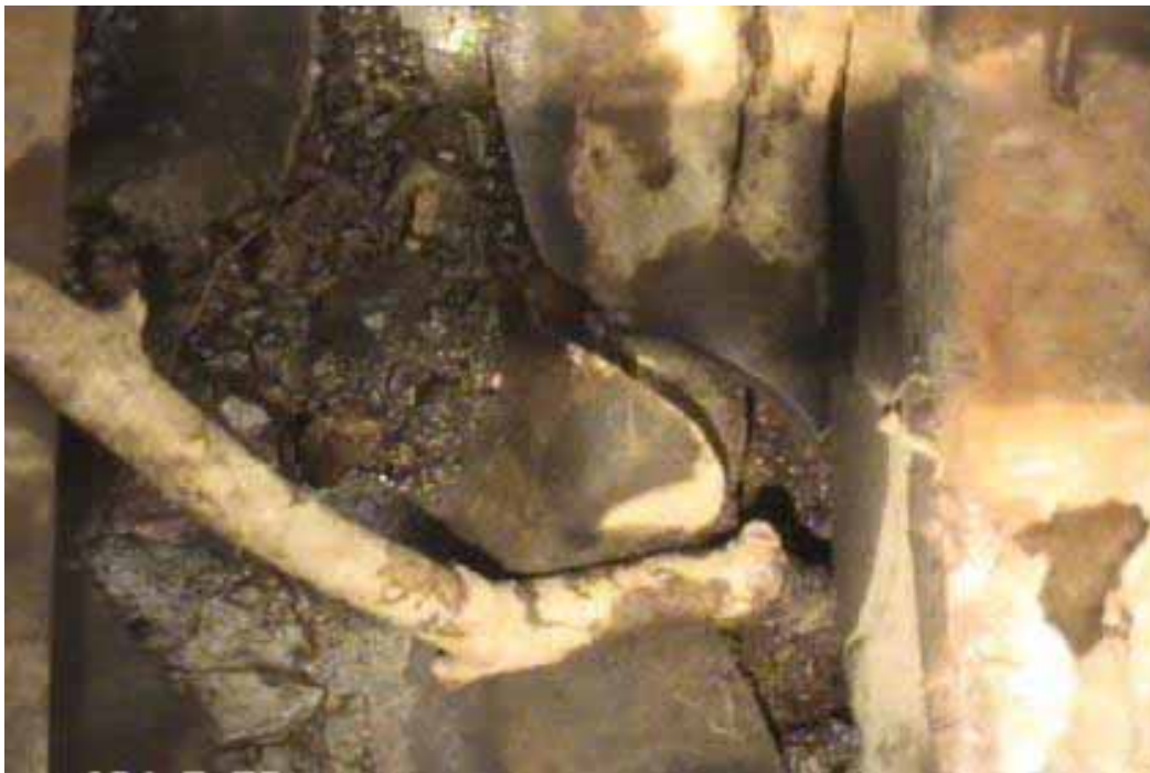
Figure 263 Cracking/fracture failure for Pipeline No. 2 (Site No. 1: Route 101)
