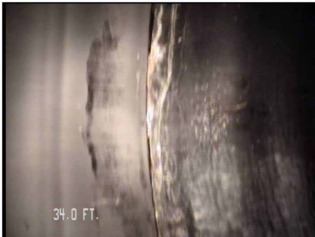
Figure 564 View of minor joint displacement for pipeline No. 12 (Site No. 2: Apopka)
