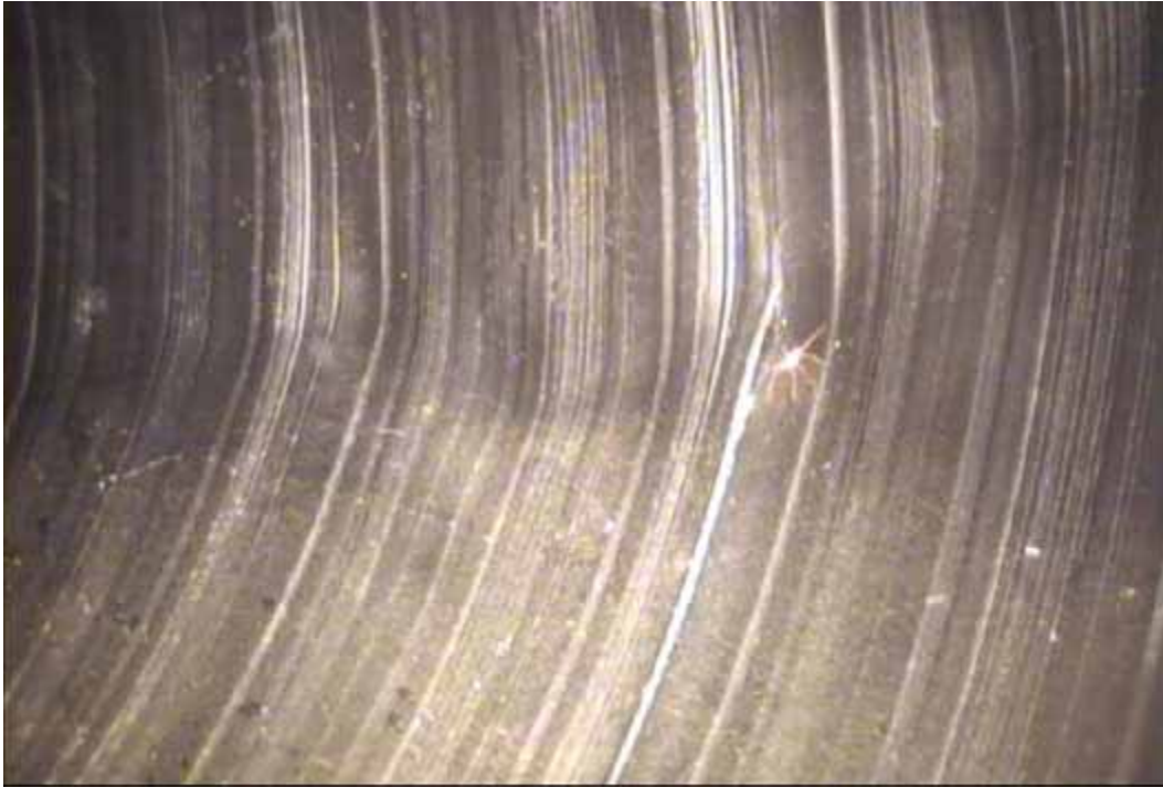
Figure 88 View of cracking and buckling failures for pipeline No. 10 (Site No. 6: Rockingham – Love Ln)
