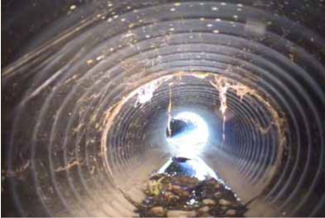
Figure 142 View of excessive deformation and major joint displacement failures for pipeline No. 14 (Site No. 6: Winchester)
