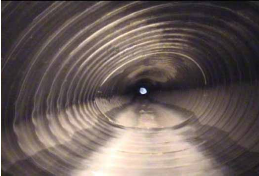
Figure 27 Buckling and excessive deformation failures for pipeline No. 2 (Site No. 1: San Antonio - HW 1604 and 1560)
