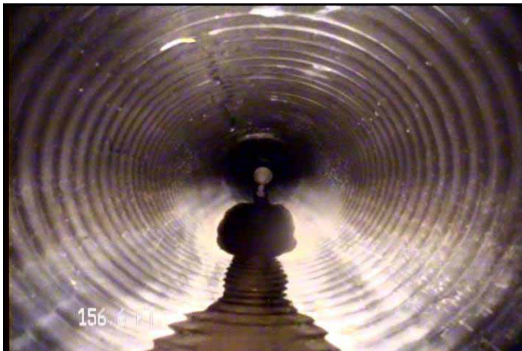
Figure 569 View of the excessive deformation, corrugation growth failures and dip in line and grade for pipeline No. 13 (Site No. 2: Apopka)
