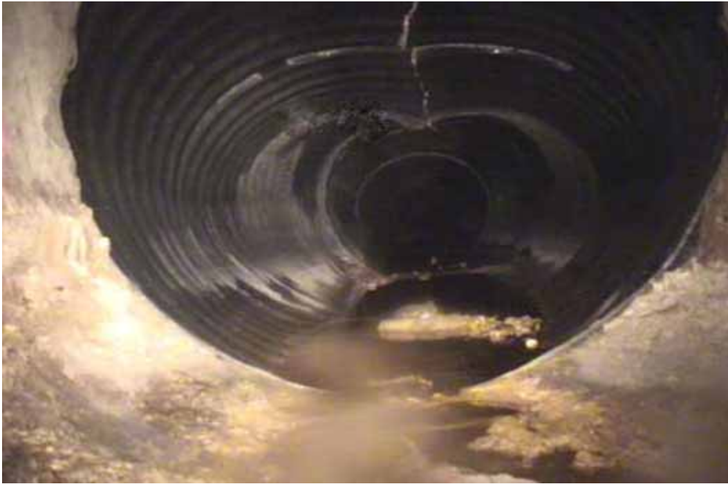
Figure 50 Excessive deformation, inverse curvature, and cracking/fracture failures for pipeline No. 20 (Segment 1) (Site No. 8: Houston – Fennell)
