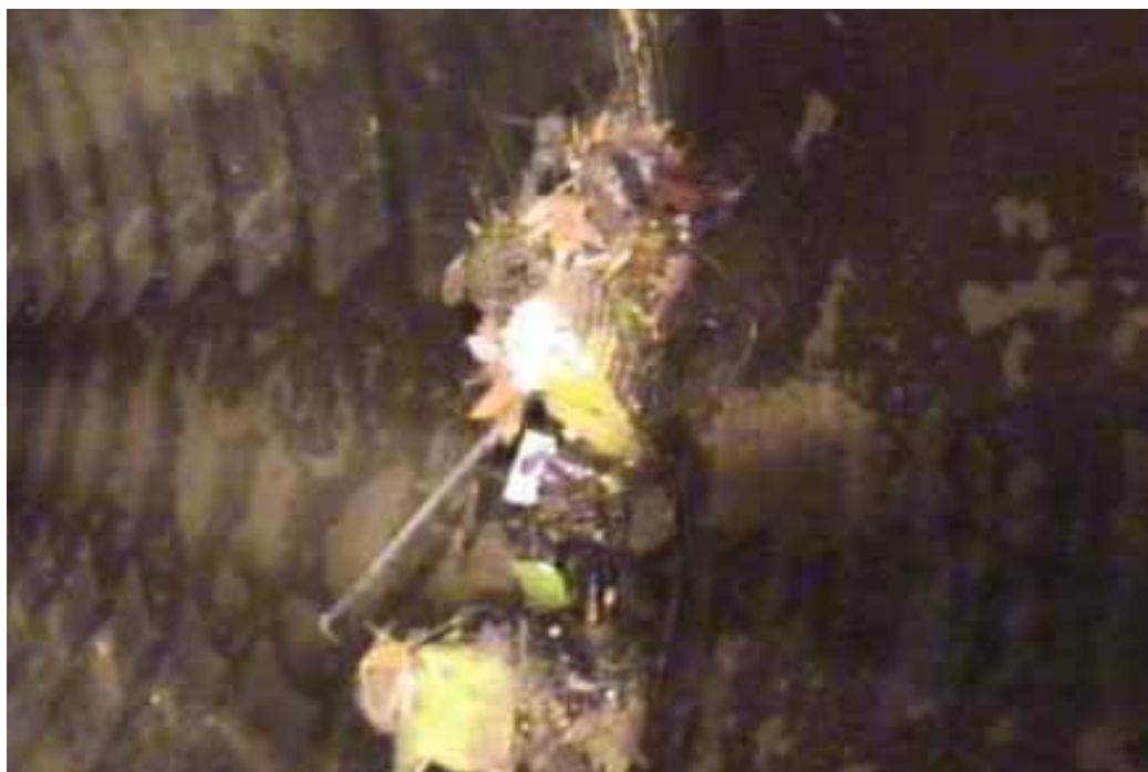
Figure 404 Corrugation growth and major joint displacement failure for Pipeline No. 5 (Site No. 5: Bad Axe)
