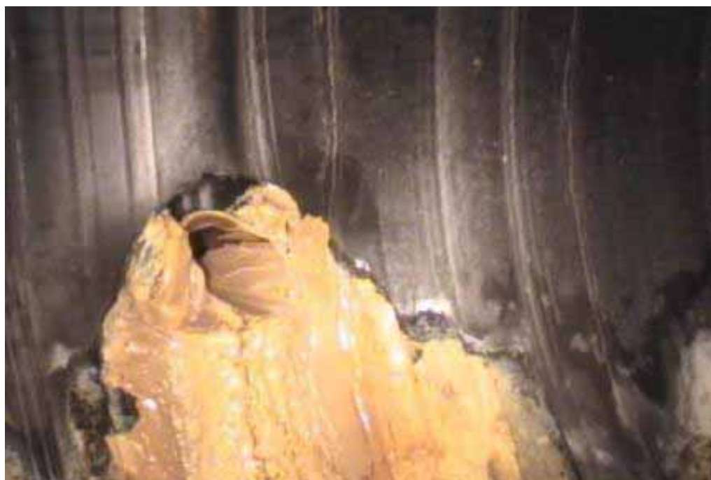
Figure 406 Corrugation growth failure with inlet added after installation for Pipeline No. 6a (Site No. 6: Houghton County M92)
