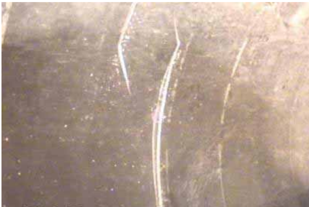
Figure 274 Cracking/fracture failure for Pipeline No. 3 (Site No. 1: Route 101)
