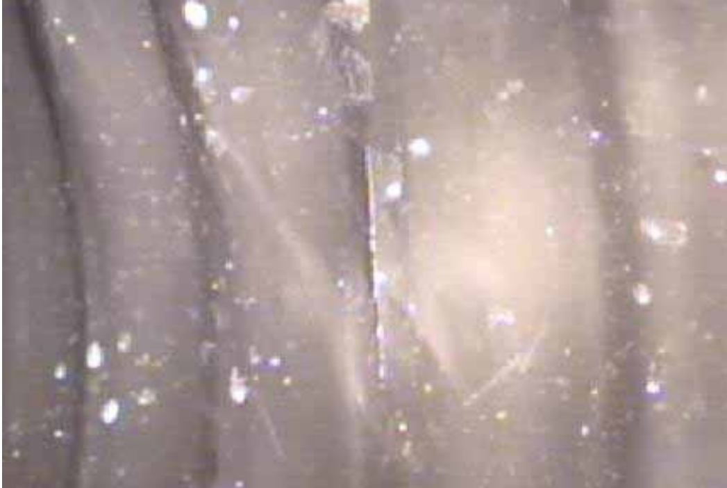
Figure 365 Cracking/fracture failure for Pipeline No. 4 (Site No. 1: Legacy Parkway)
