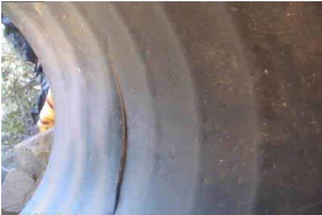
Figure 314 Cracking/fracture failure for Pipeline No. 10 (Site No. 1: Route 101)
