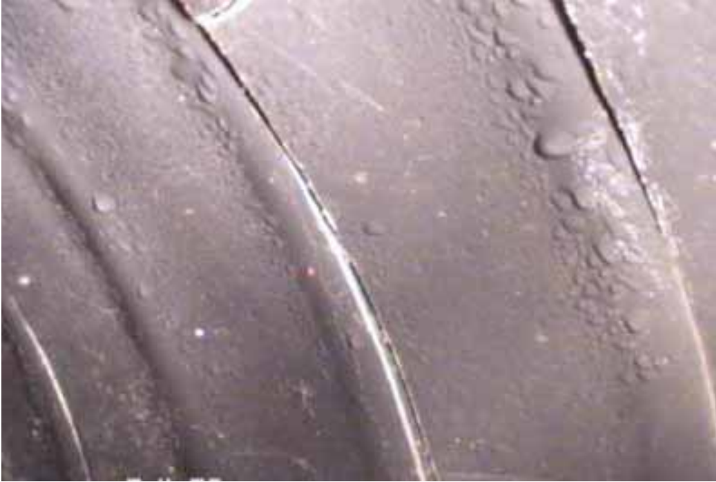
Figure 342 Cracking/fracture failure for Pipeline No. 23 (Site No. 2: Route 36)
