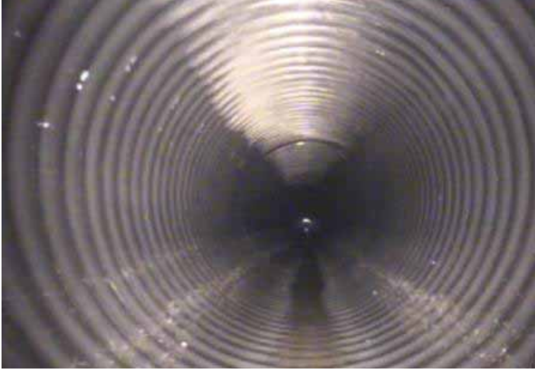
Figure 206 View of corrugation growth failure for pipeline No. 1 (Site No. 1: Lenexa)
