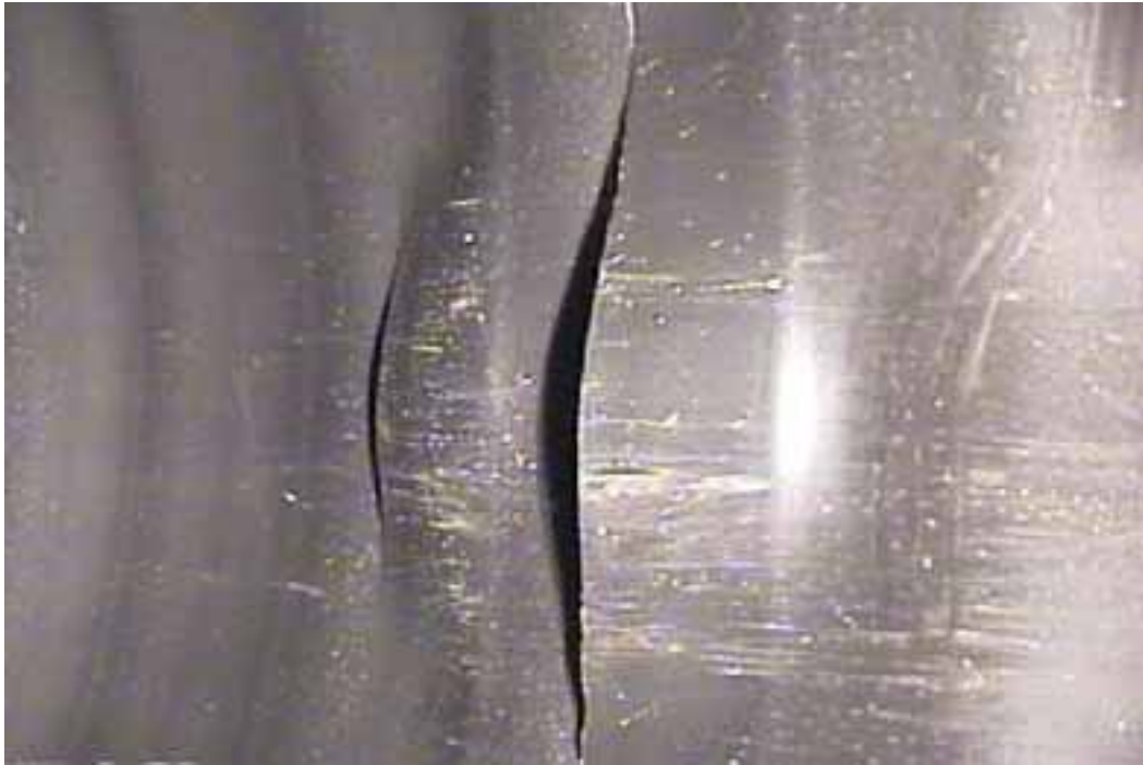
Figure 377 Cracking/fracture failure for Pipeline No. 9 (Site No. 2: Silver Creek Parkway)
