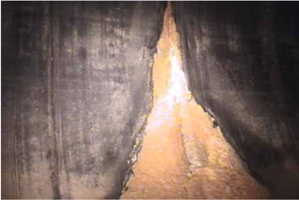
Figure 54 Cracking/fracture failure for pipeline No. 20 (Segment 2) (Site No. 8: Houston – Fennell)
