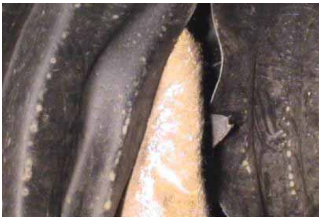
Figure 292 Cracking/fracture failure for Pipeline No. 7 (Site No. 1: Route 101)
