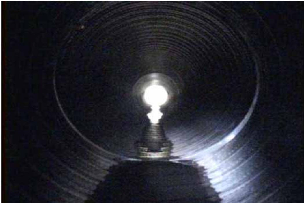
Figure 155 View of corrugation growth failure for pipeline No. 19 (Site No. 6: Winchester)
