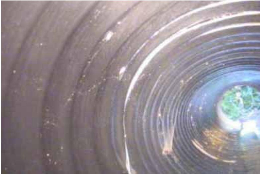
Figure 334 Cracking/fracture and corrugation growth failure for Pipeline No. 22 (Site No. 2: Route 36)
