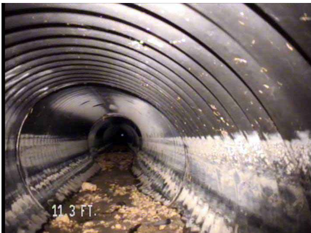
Figure 552 View of the excessive deformation and corrugation growth failures for pipeline No. 11 (Site No. 2: Apopka)
