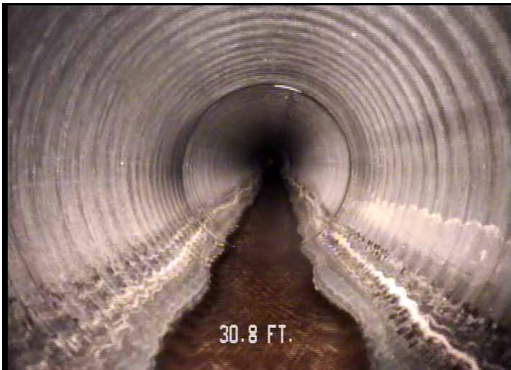
Figure 543 View of the corrugation growth, and dip in line and grade for pipeline No. 10 (Site No. 2: Apopka)
