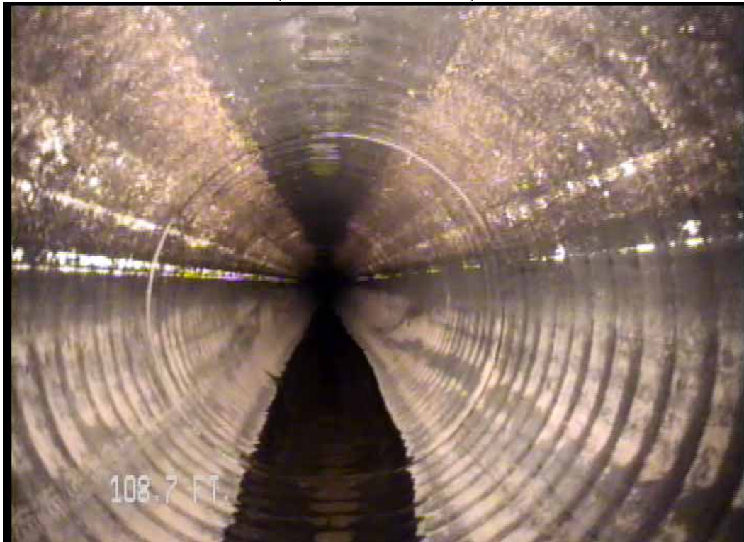
Figure 508 View of the corrugation growth failure for pipeline No. 6 (Site No. 1: Orlando)
