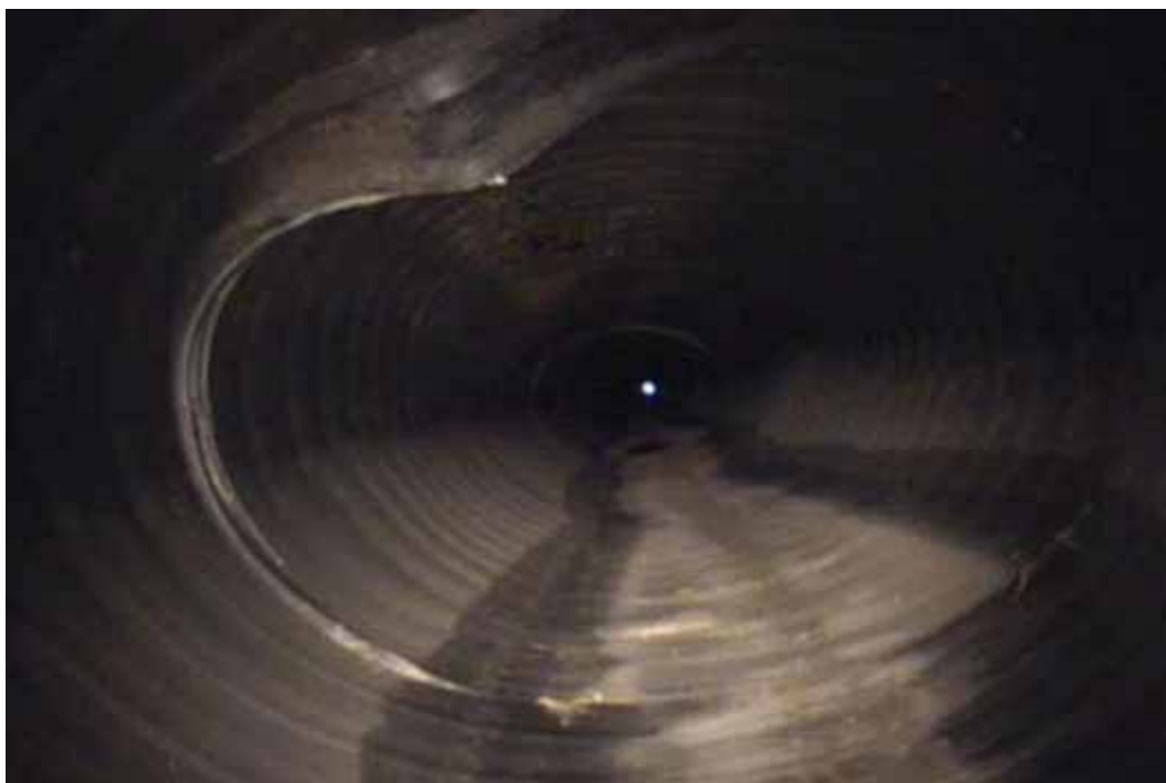
Figure 22 Inverse curvature and corrugation growth failure modes for pipeline No. 1 (Site No. 1: San Antonio – HW 1604 & 1560)
