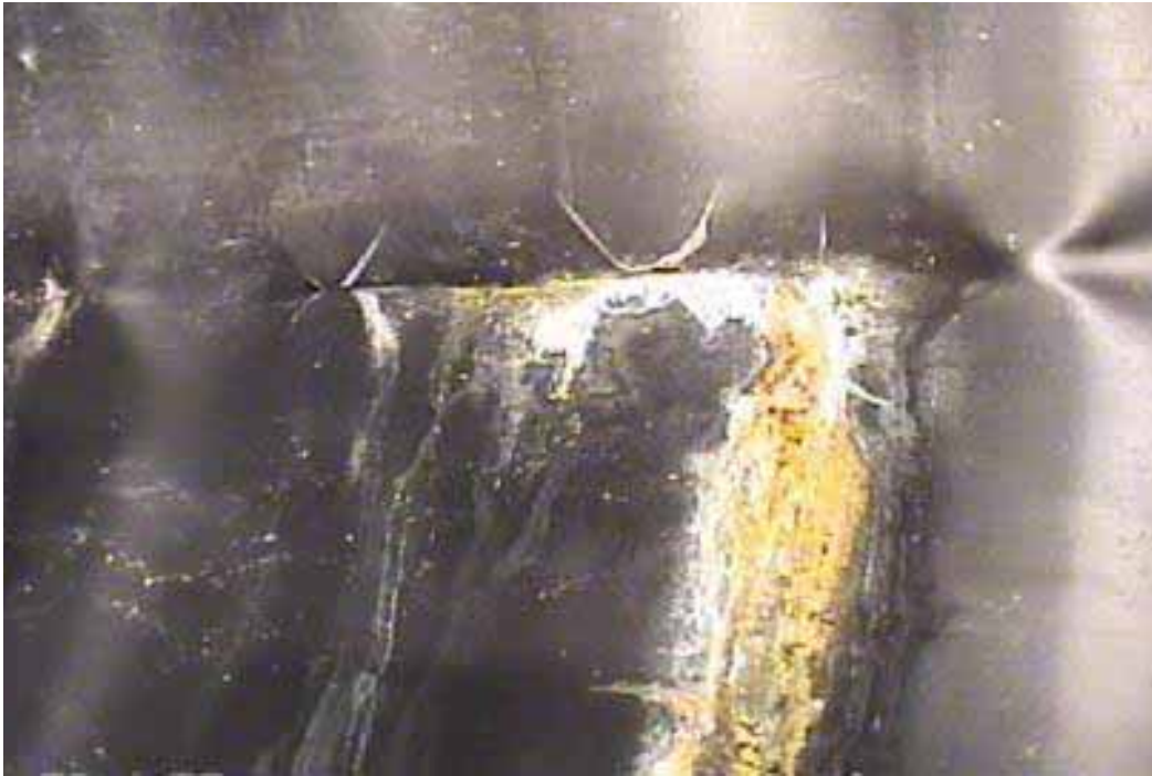
Figure 379 Cracking/fracture and buckling failure for Pipeline No. 9 (Site No. 2: Silver Creek Parkway)
