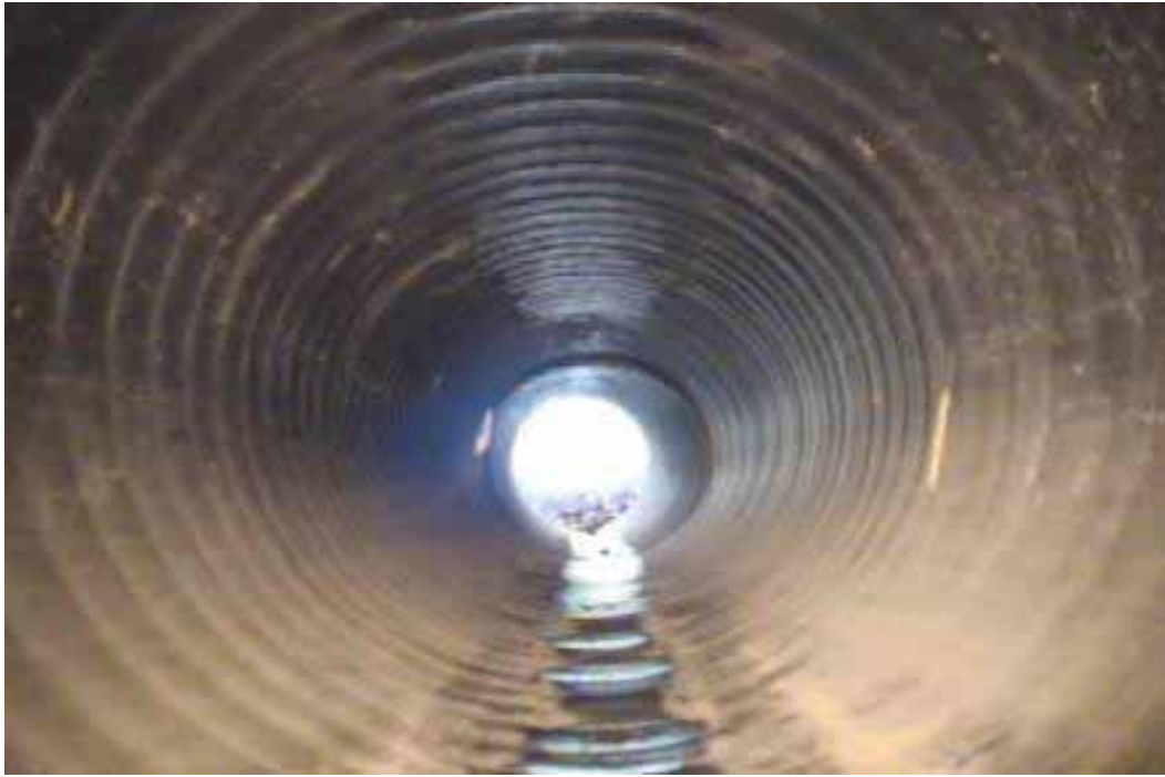
Figure 325 Corrugation growth failure for Pipeline No. 18 (Site No. 2: Route 36)
