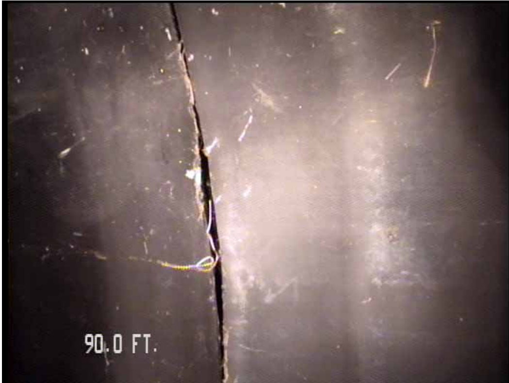
Figure 577 View of minor joint displacement for pipeline No. 14 (Site No. 2: Apopka)
