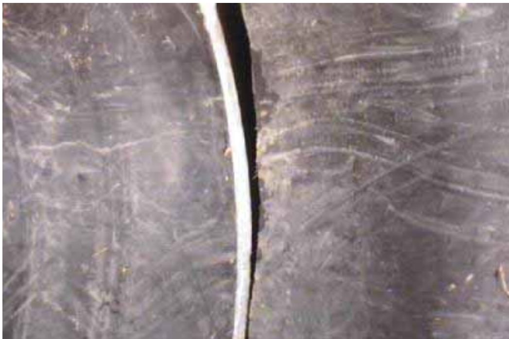
Figure 285 Cracking/fracture failure for Pipeline No. 6 (Site No. 1: Route 101)
