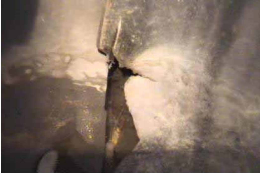
Figure 271 Cracking/fracture failure for Pipeline No. 3 (Site No. 1: Route 101)
