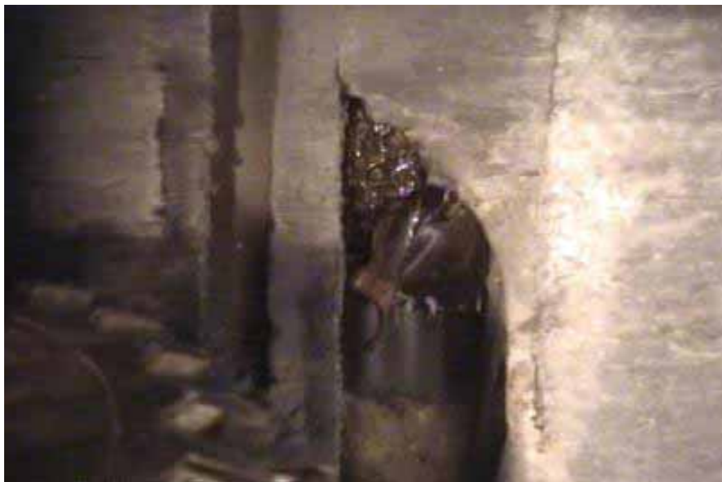
Figure 256 Cracking/fracture failure for Pipeline No. 1 (Site No. 1: Route 101)
