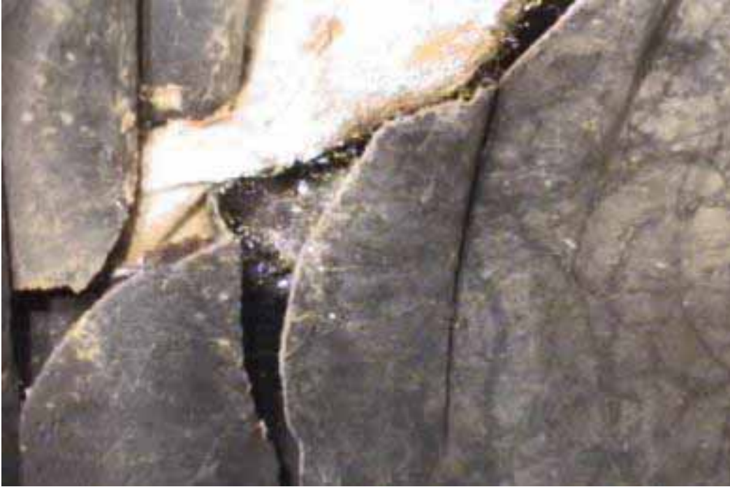
Figure 293 Cracking/fracture for Pipeline No. 7 (Site No. 1: Route 101)
