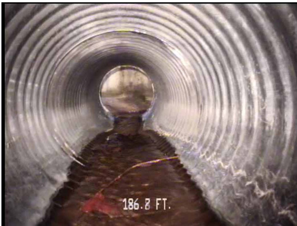
Figure 546 View of the corrugation growth and dips in line and grade for pipeline No. 10 (Site No. 2: Apopka)
