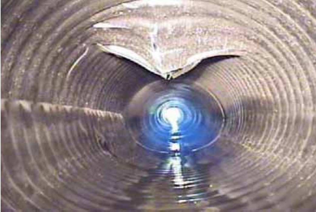
Figure 383 Cracking/fracture, inverse curvature, buckling, and excessive deformation (refer to Figure 376-c), and corrugation growth failure for Pipeline No. 9 (Site No. 2: Silver Creek Parkway)
