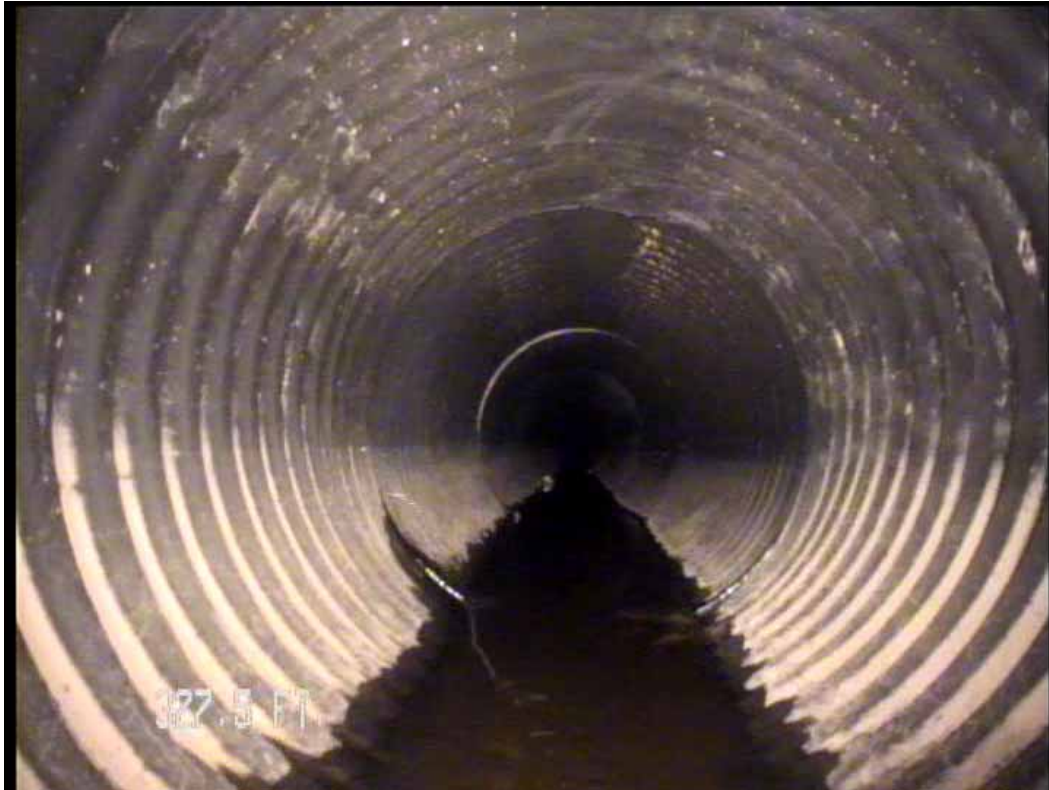
Figure 499 View of the corrugation growth failure for pipeline No. 3 (Site No. 1: Orlando)
