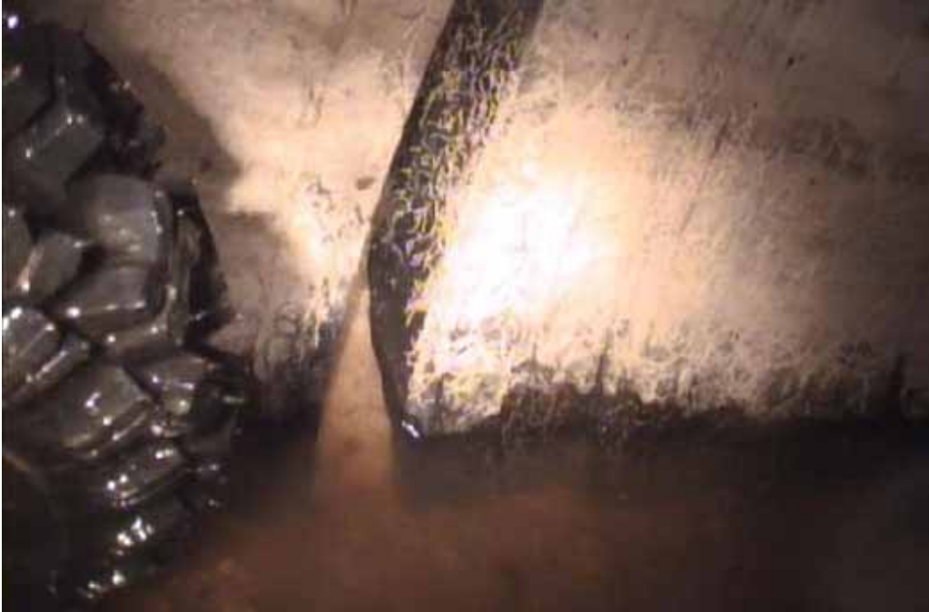
Figure 77 View of and joint displacement failures for pipeline No. 8 (Site No. 4: Wendell – Hunt dell Main Drive)
