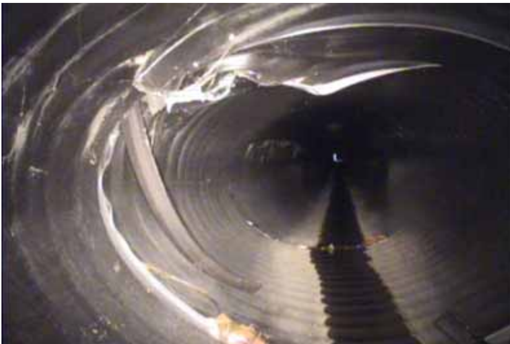
Figure 126 View of cracking/fracture and excessive deformation failures for pipeline No. 6 (Site No. 4: Mechanicsville)
