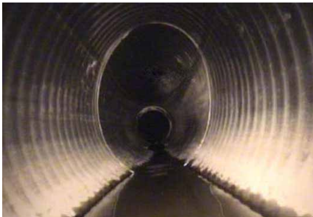
Figure 180 View of corrugation growth and excessive deformation failures for pipeline No. 18 (Site No. 6: Brooklyn Park - DuPont)
