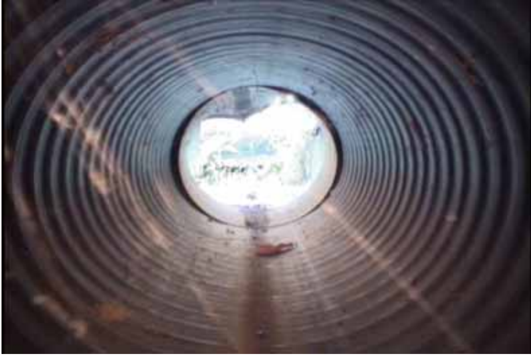
Figure 240 Corrugation growth for pipeline No. 9 (Site No. 3: Franklin County – Route FF)
