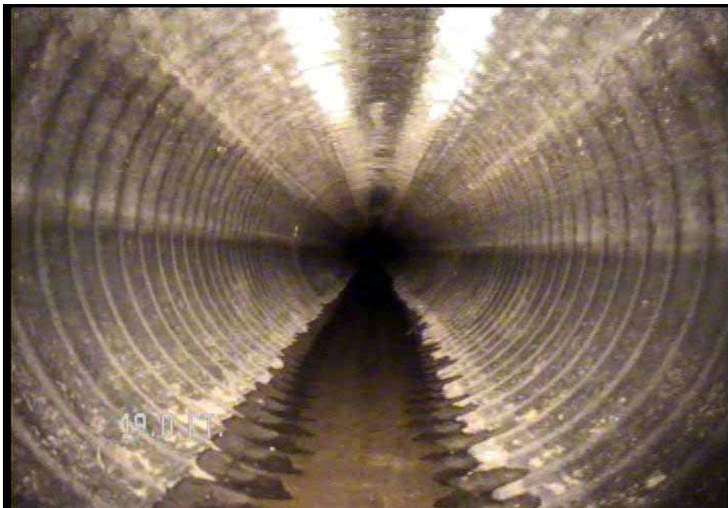
Figure 516 View of corrugation growth failure for pipeline No. 7 (Site No. 1: Orlando)
