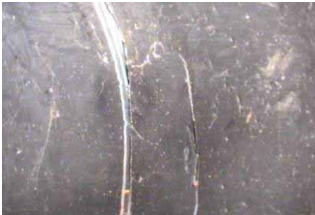
Figure 309 Cracking/fracture failure for Pipeline No. 10 (Site No. 1: Route 101)
