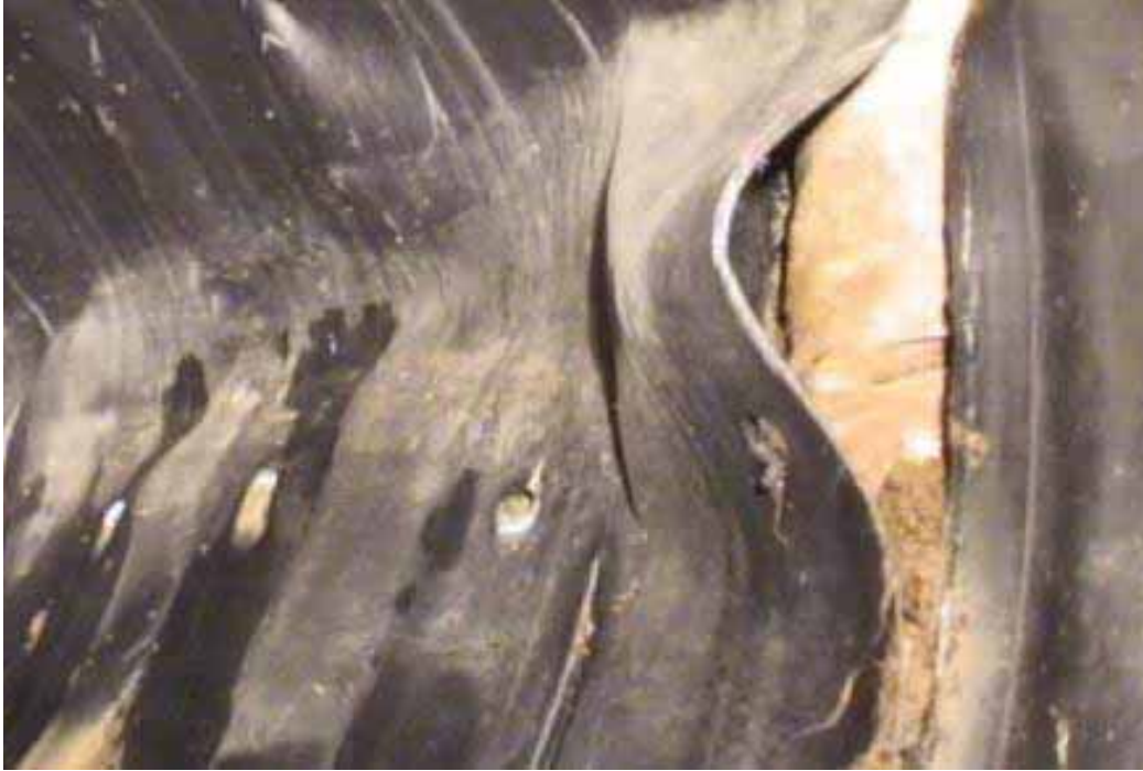
Figure 409 Cracking/fracture failure for Pipeline No. 6a (Site No. 6: Houghton County M92)
