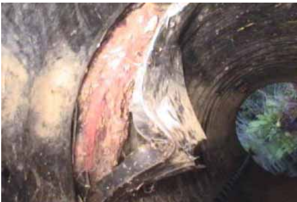
Figure 329 Cracking/fracture failure for Pipeline No. 20 (Site No. 2: Route 36)
