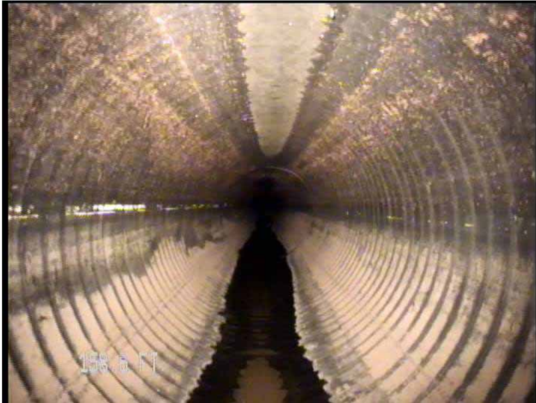
Figure 512 View of the corrugation growth failure for pipeline No. 6 (Site No. 1: Orlando)
