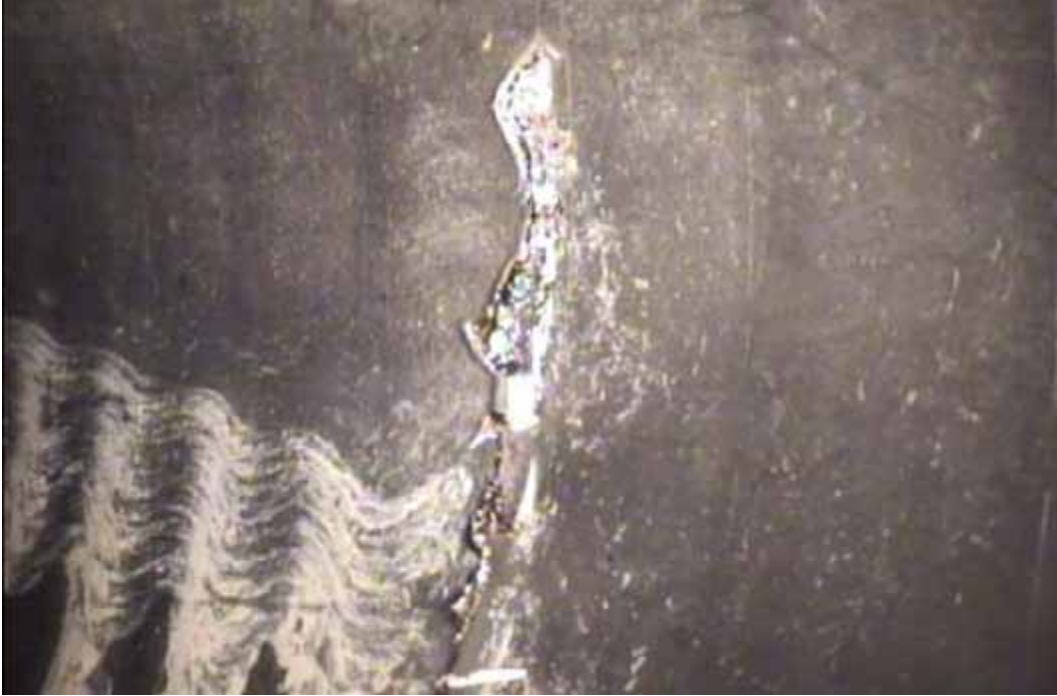
Figure 67 View of cracking failures for pipeline No. 5 (Site No. 2: Elm City – Lake Wilson Rd)
