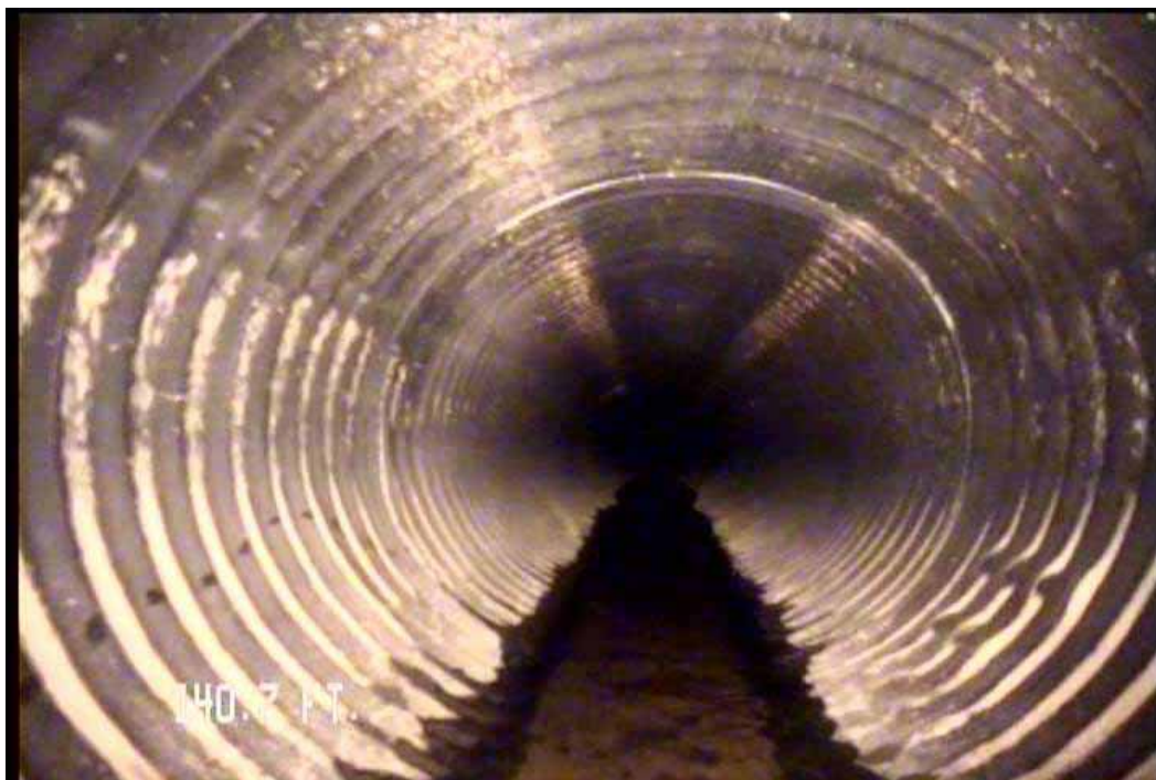
Figure 502 View of the excessive deformation, corrugation growth and buckling failures for pipeline No. 3 (Site No. 1: Orlando)
