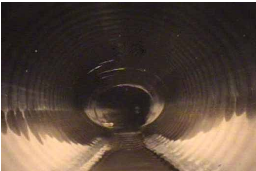
Figure 43 Excessive deformation and corrugation growth failures for pipeline No. 19 (Segment 1) (Site No. 8: Houston – Fennell)
