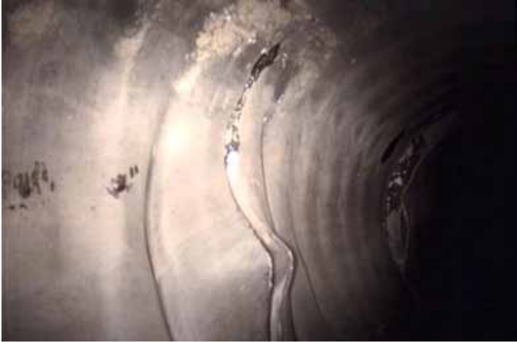
Figure 148 View of buckling and cracking/fracture failures for pipeline No. 16 (Site No. 6: Winchester)
