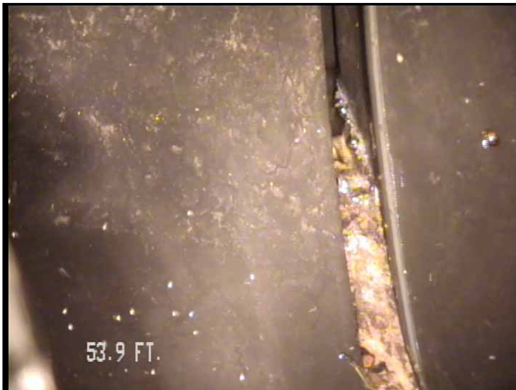
Figure 486 View of the major joint displacement failure for pipeline No. 2 (Site No. 1: Orlando)
