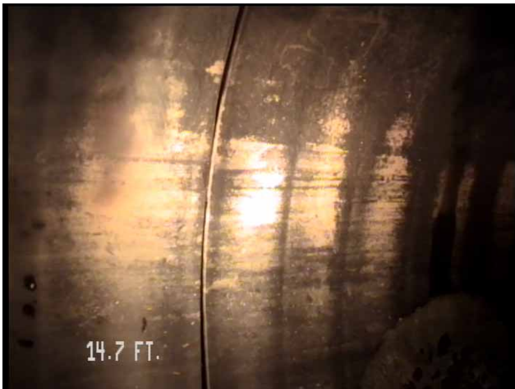
Figure 483 View of the minor joint displacement failure for pipeline No. 2 (Site No. 1: Orlando)
