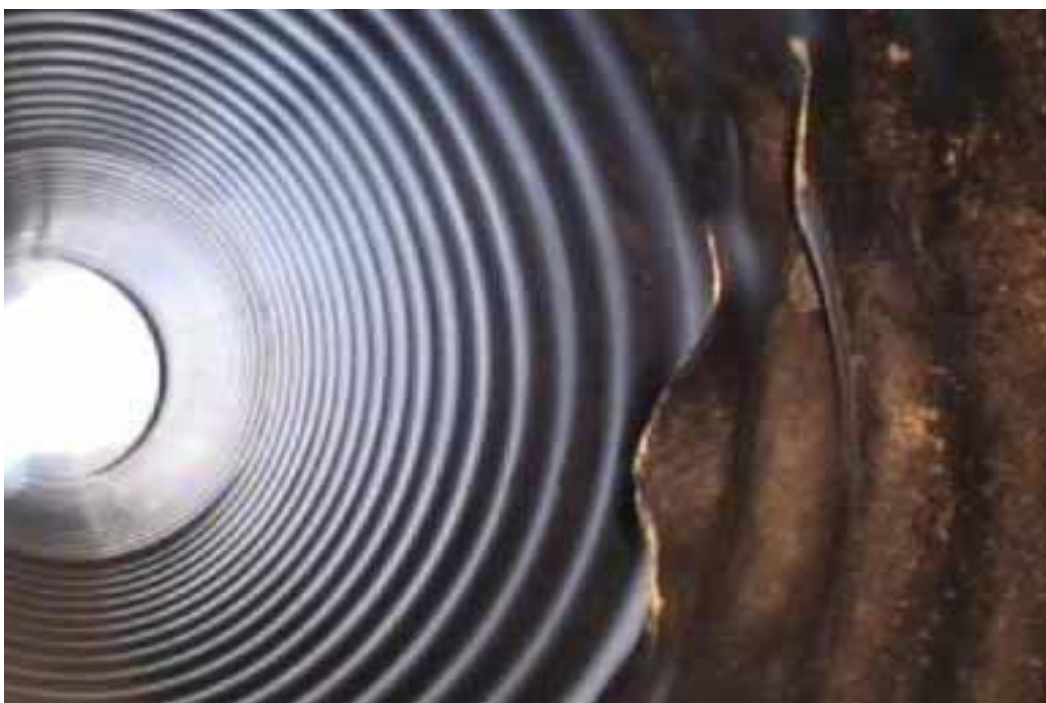
Figure 389 Cracking/fracture, corrugation growth, and inverse curvature failure for Pipeline No. 10 (Site No. 2: Silver Creek Parkway)
