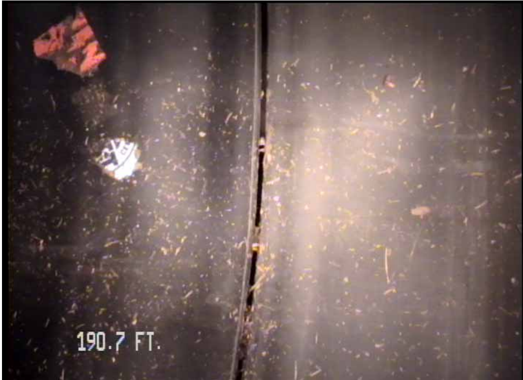
Figure 510 View of the minor joint displacement failure for pipeline No. 6 (Site No. 1: Orlando)
