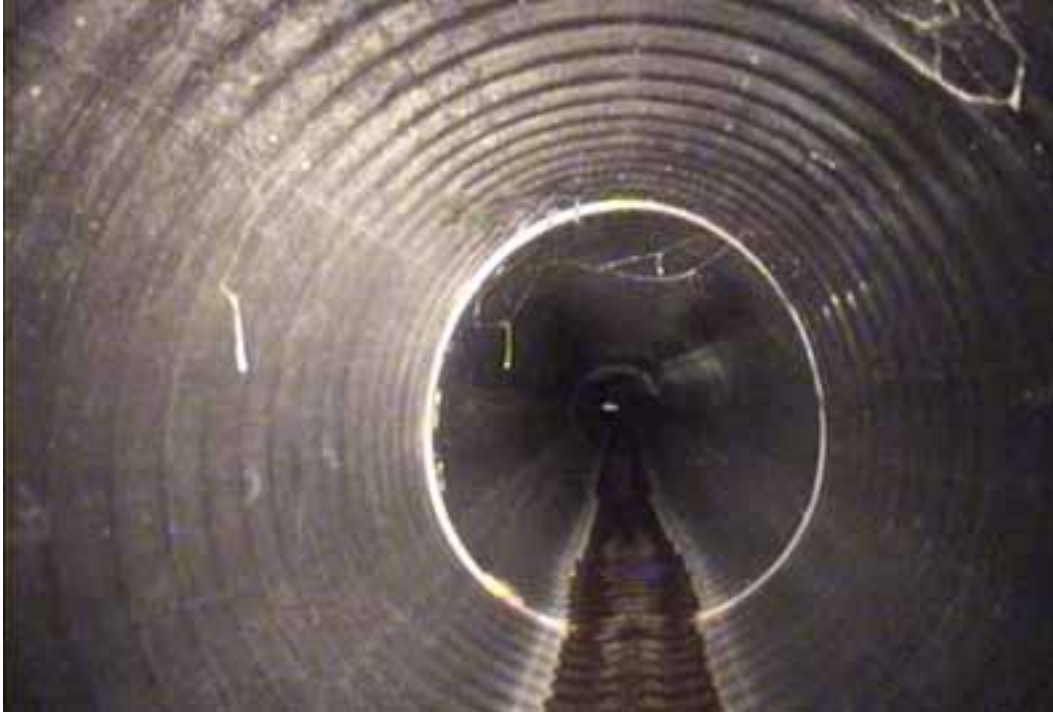
Figure 116 View of the excessive deformation failure for pipeline No. 3 (Site No. 2: Chesterfield – Bandermill)
