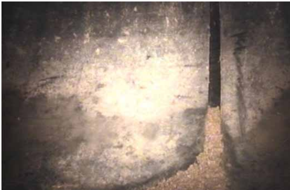
Figure 109 View of the joint displacement failure for pipeline No. 1 (Site No. 1: Chesterfield - Commonwealth Pkwy)
