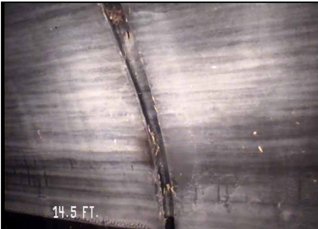
Figure 574 View of the major joint displacement failure for pipeline No. 14 (Site No. 2: Apopka)
