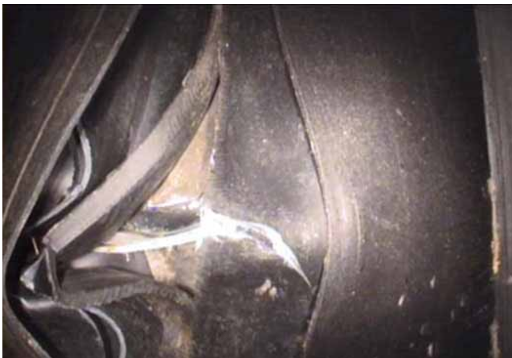
Figure 24 Cracking/fracture and buckling failures for pipeline No. 1 (Site No. 1: San Antonio - HW 1604 and 1560)
