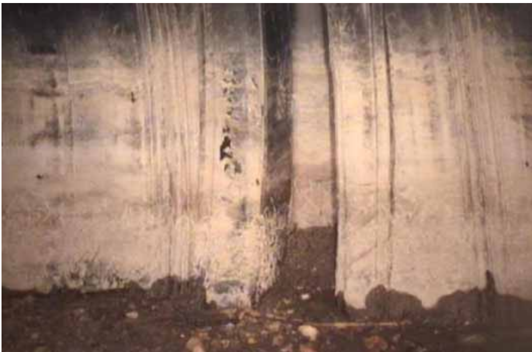
Figure 76 View of major joint displacement failure for pipeline No. 8 (Site No. 4: Wendell – Huntzell Main Drive)
