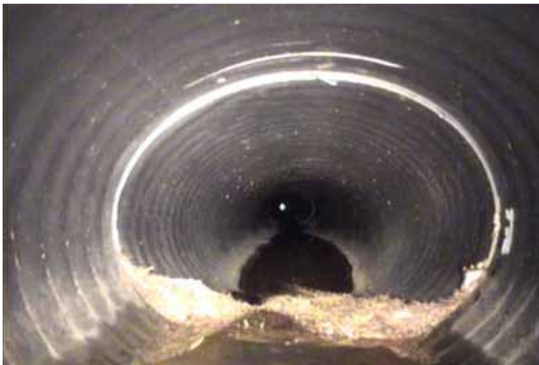
Figure 120 View of joint between two segments of the pipes for pipeline No. 4 (Site No. 3: Spotsylvania County)
