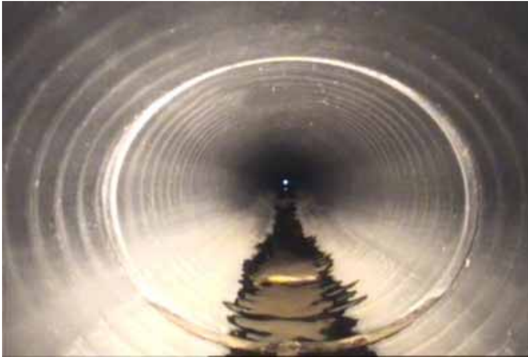
Figure 135 View of excessive deformation failure for pipeline No. 9 (Site No. 4: Mechanicsville)
