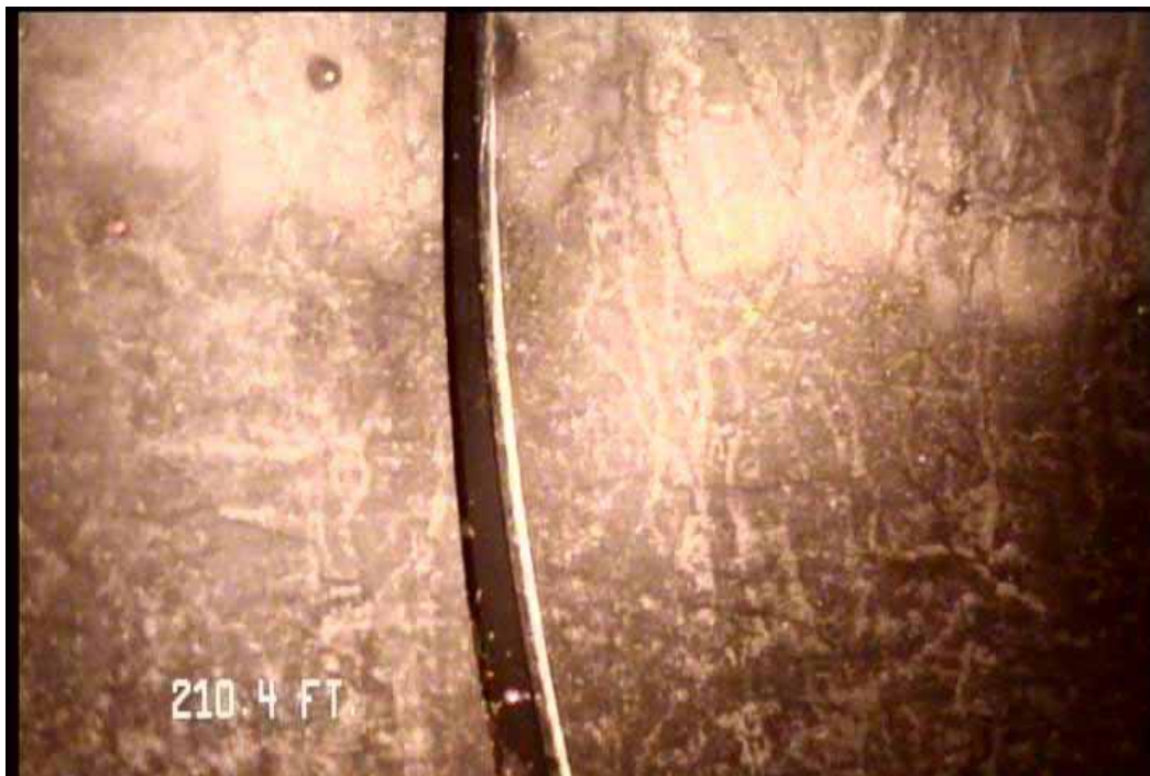
Figure 488 View of major joint displacement failure for pipeline No. 2 (Site No. 1: Orlando)
