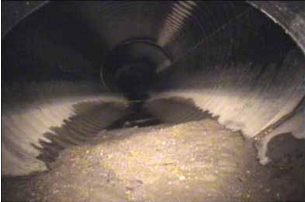
Figure 111 View of opening of the pipe for pipeline No. 2 (Site No. 1: Chesterfield - Commonwealth Pkwy)
