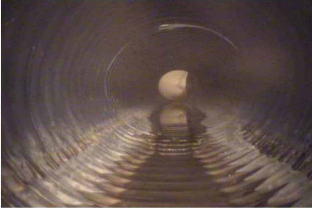
Figure 193 View of excessive deformation failure for pipeline No. 27 (Site No. 8: Fairmont)
