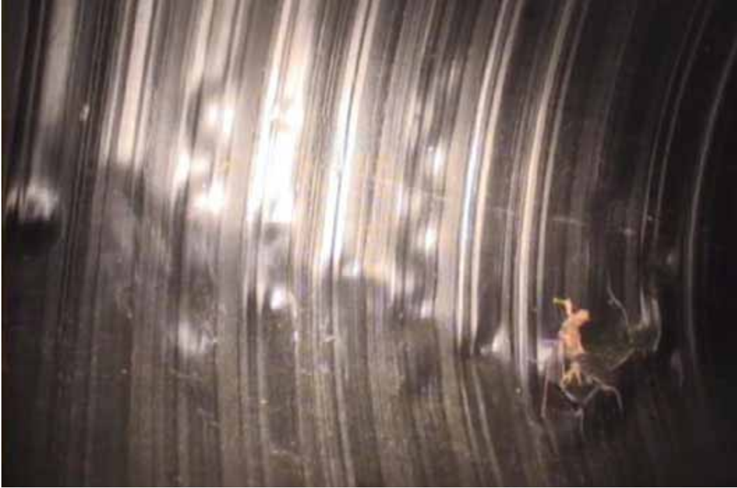
Figure 86 View of buckling and cracking failures for pipeline No. 10 (Site No. 6: Rockingham – Love Ln)
