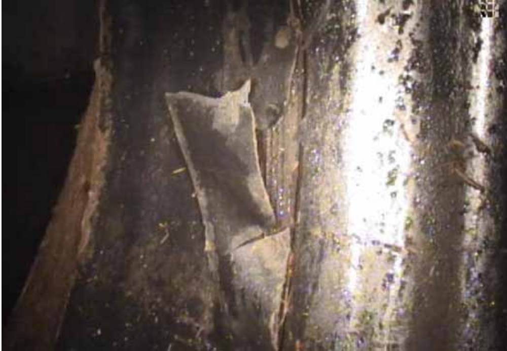
Figure 161 View of the cracking/fracture failure for pipeline No. 3 (Site No. 1: Brooklyn Park - 64 th Ave)
