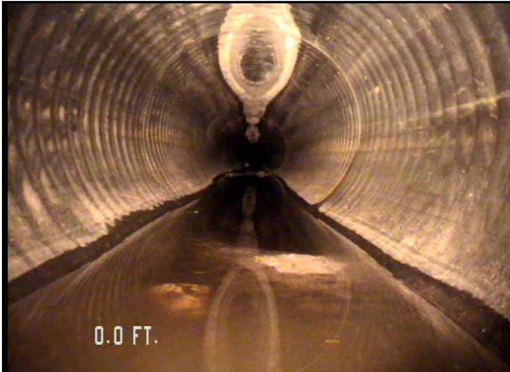
Figure 524 View of corrugation growth failure at the opening of pipeline No. 8 (Site No. 1: Orlando)
