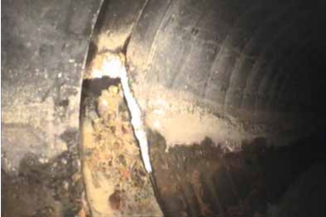
Figure 134 View of major joint displacement failure for pipeline No. 8 (Site No. 4: Mechanicsville)
