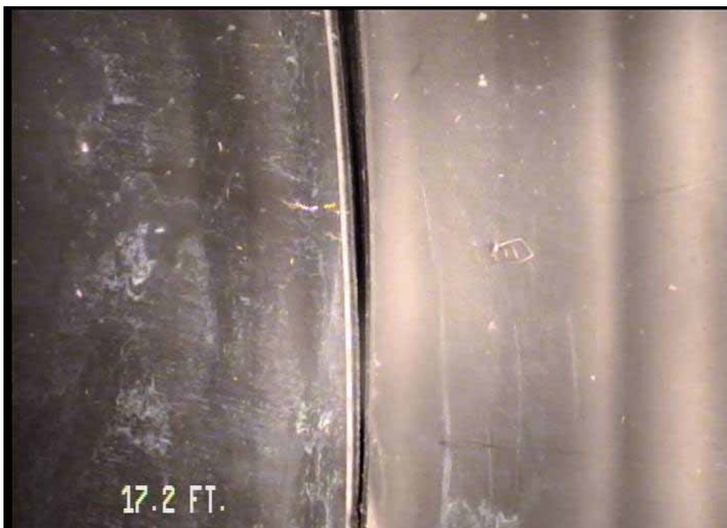
Figure 568 View of minor joint displacement failure for pipeline No. 13 (Site No. 2: Apopka)
