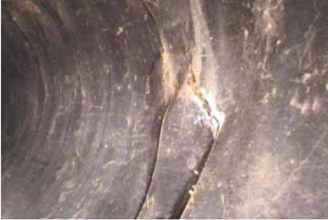
Figure 324 Cracking/fracture failure for Pipeline No. 17 (Site No. 2: Route 36)
