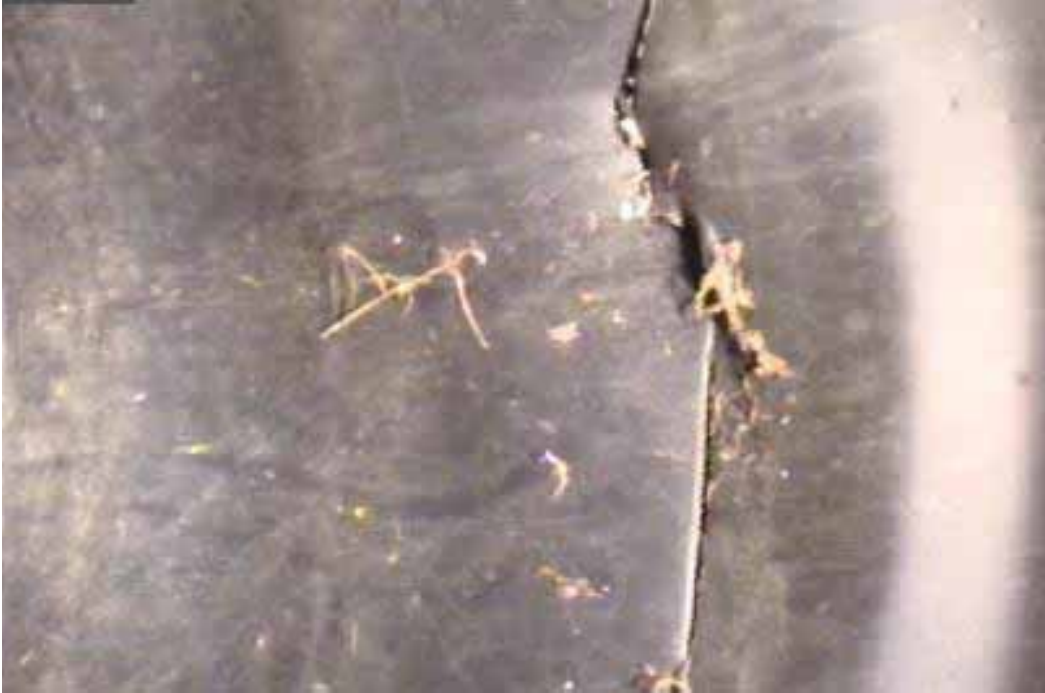
Figure 286 Cracking/fracture failure for Pipeline No. 6 (Site No. 1: Route 101)
