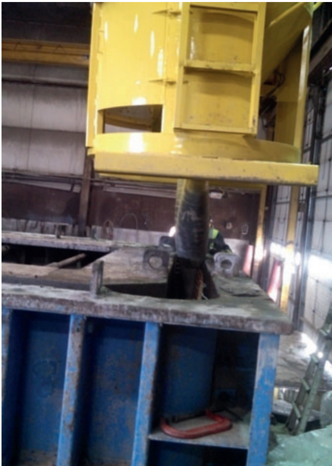
A radio-controlled pour bucket with flexible pouring boot attached to the clam gate on the bottom of the pour bucket
