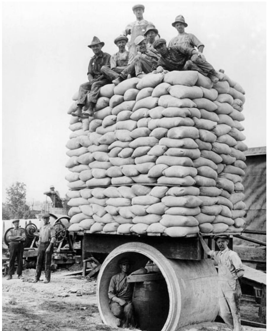
Workers loading large diameter concrete pipe with sand bags for load bearing test. The photo strongly suggests that pipe producers were aware of the need for long-lasting durable pipelines and culverts constructed with their pipe. Legacy pipelines and culverts attest to the quality of the pipe. Photo: Courtesy of American Concrete Pipe Association
